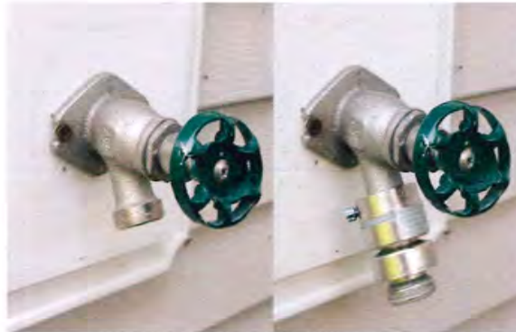
Vacuum Breaker installed on outside hose bib
