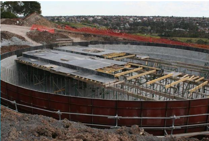
Underground Storage Chamber
