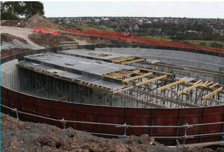
Underground Storage Chamber
