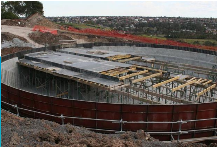
Underground Storage Chamber
