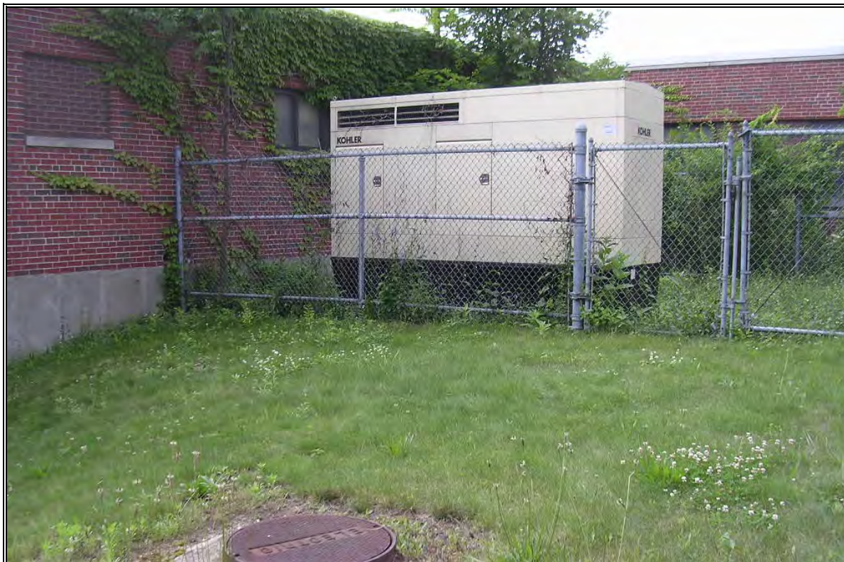
Photo Number 21: Diesel generator adjacent to Farrell Hall, location of AST 3A.
