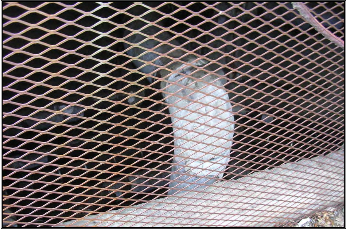
Photo Number 41: Damaged thermal system insulation in open steam pipe vault.
