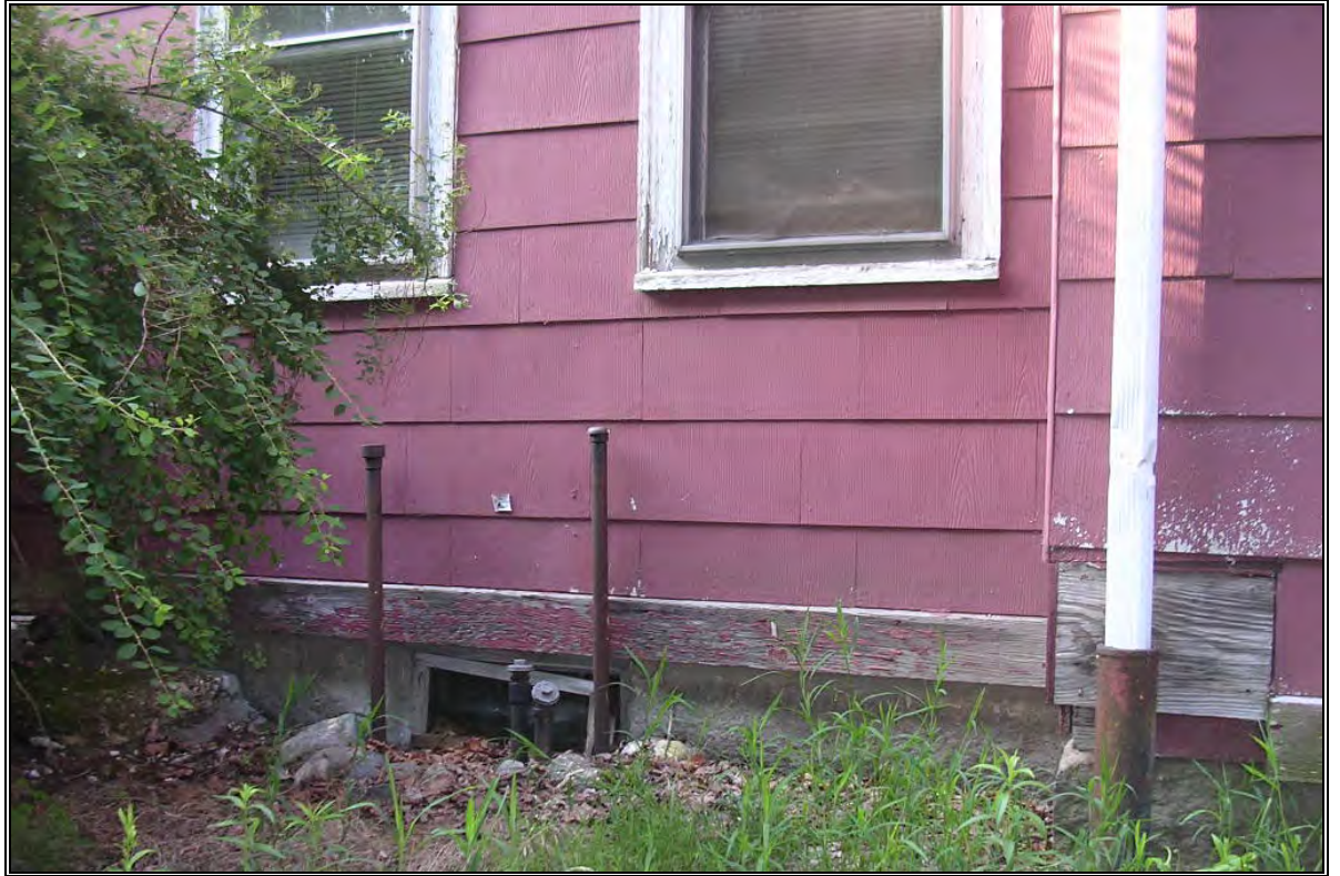
Photo Number 25: Fill and vent pipes for two ASTs in basement of Volunteer Center. Note asbestos siding.
