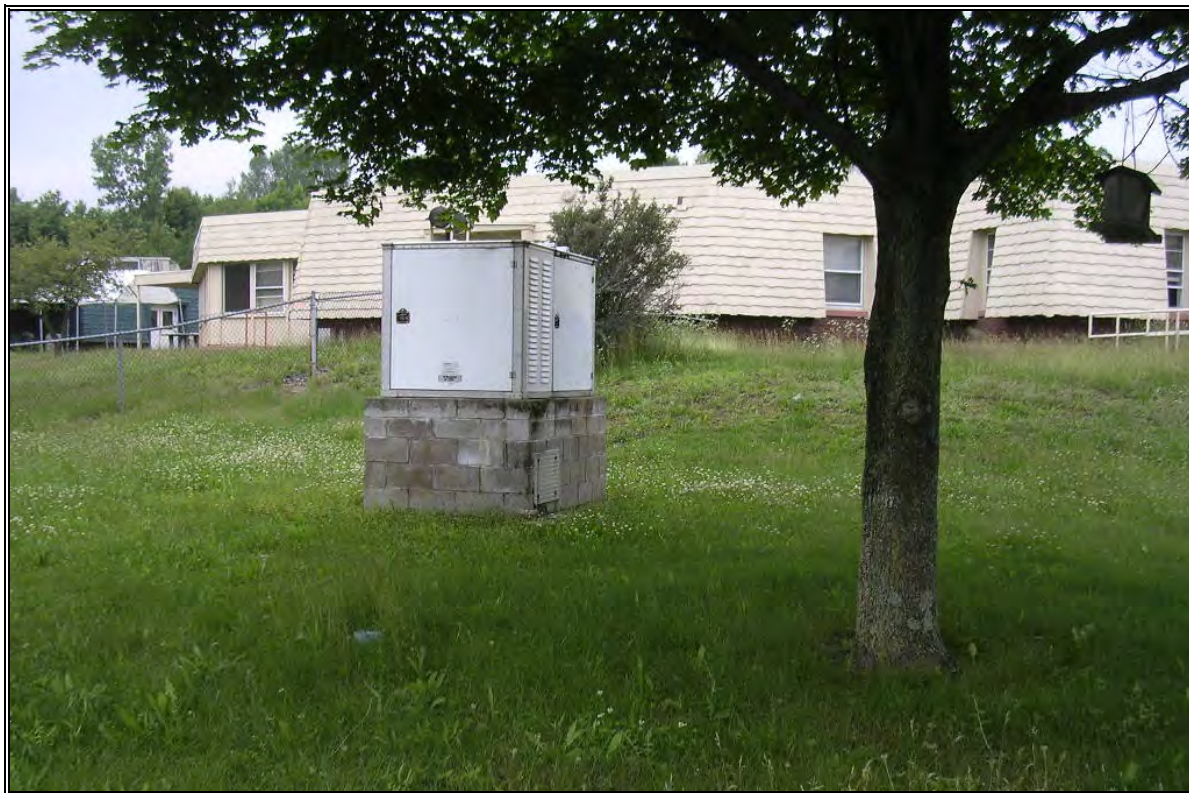
Photo Number 13: Generator near Cottage #11 with AST (14A) in inside concrete block structure.
