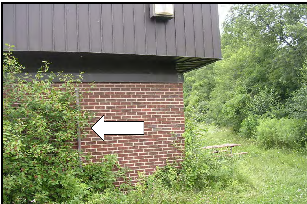
Photo Number 12: View of UST vent pipe adjacent to Site 5 building.
