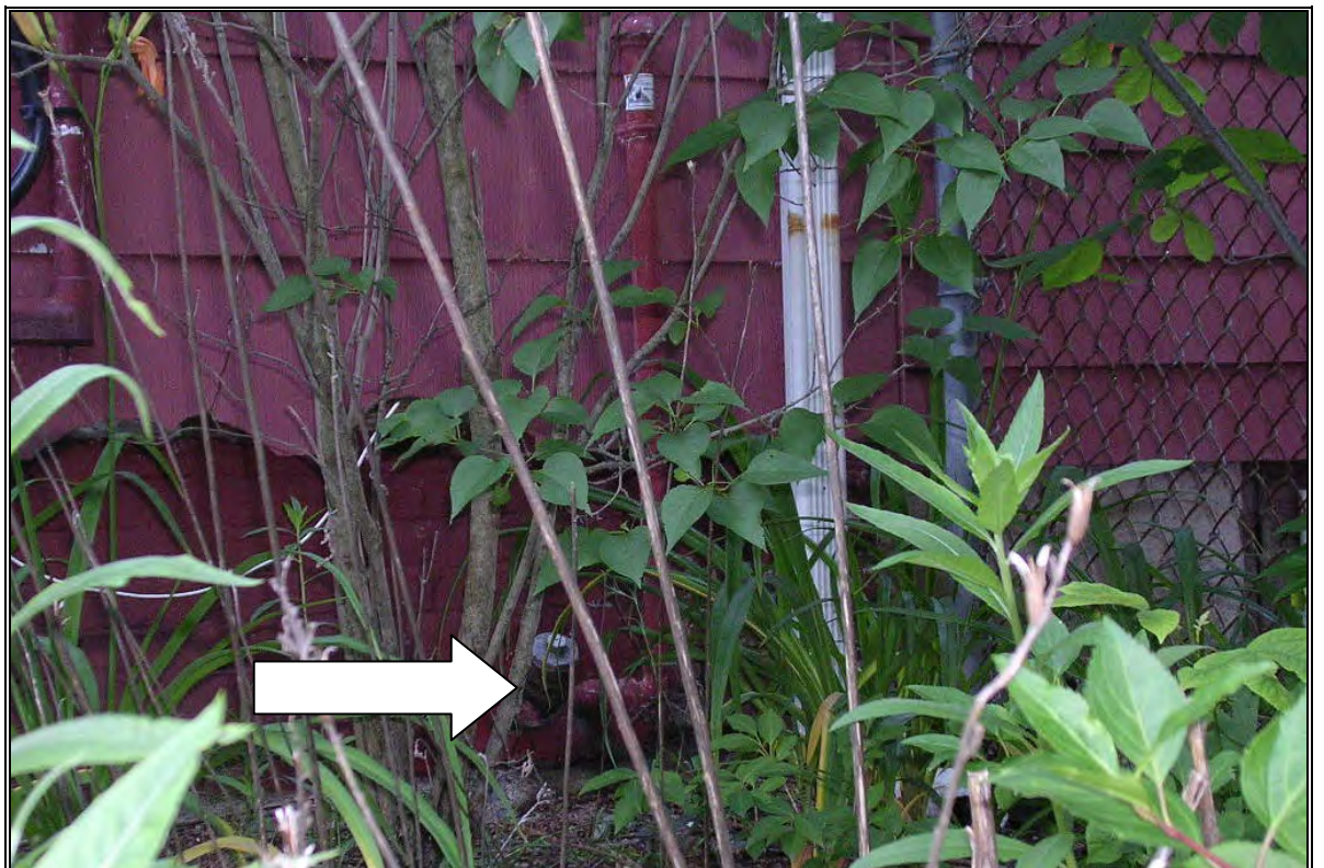
Photo Number 26: AST fill and vent pipes at 180 Trapelo Road (former Day Care Center) and asbestos siding.
