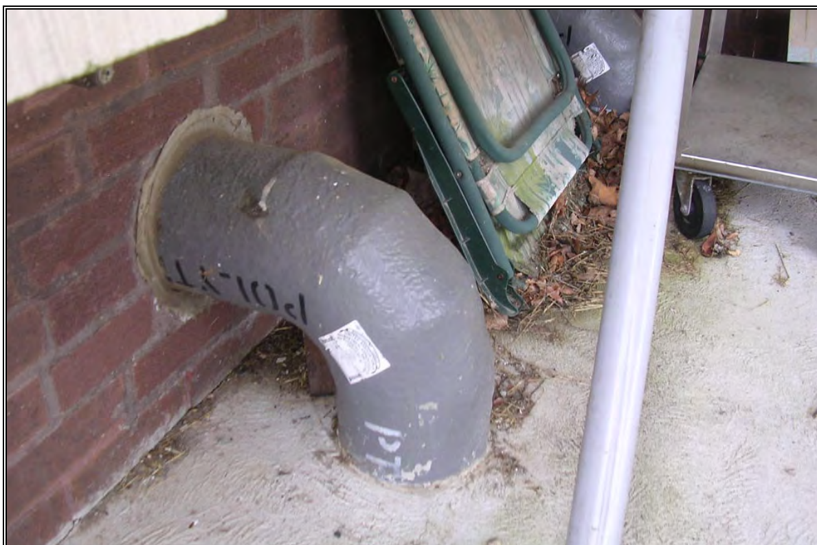
Photo Number 14: Hot water heating pipe enters Cottage Complex buildings from ground.
