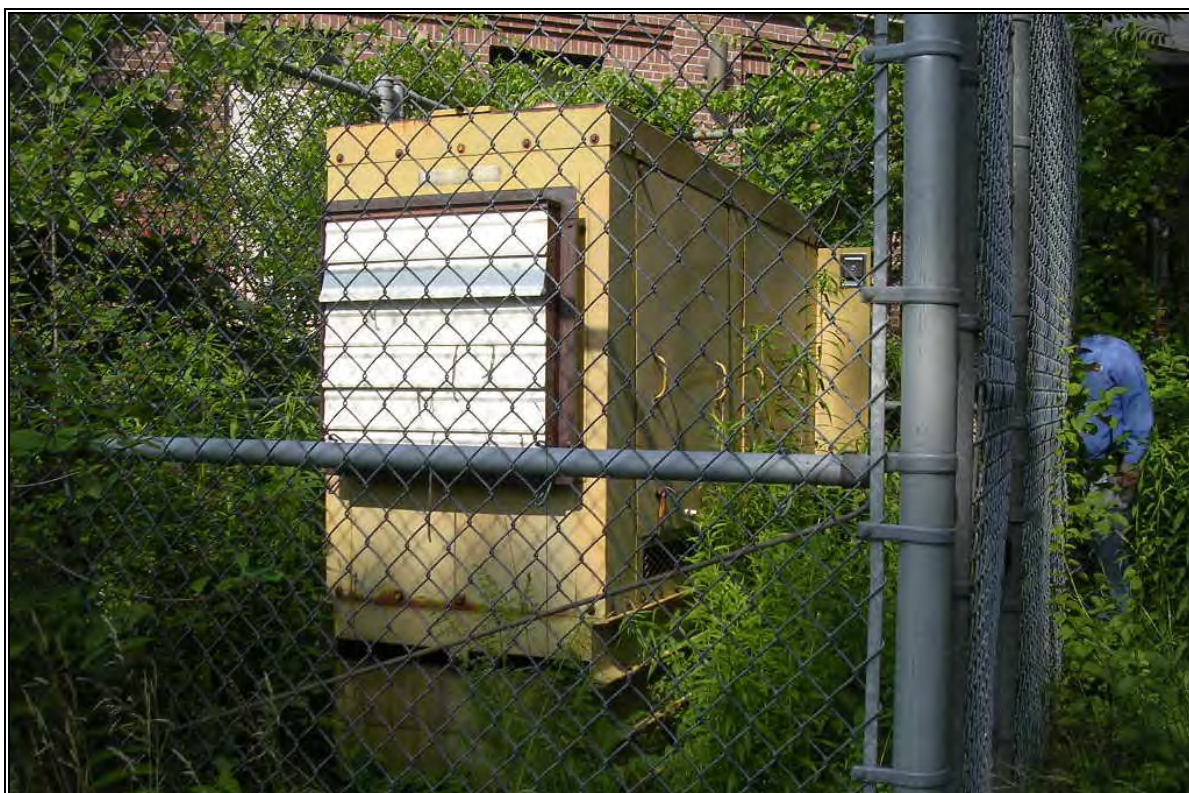
Photo Number 22: Diesel generator adjacent to Seguin Hall (location of AST 12A)
