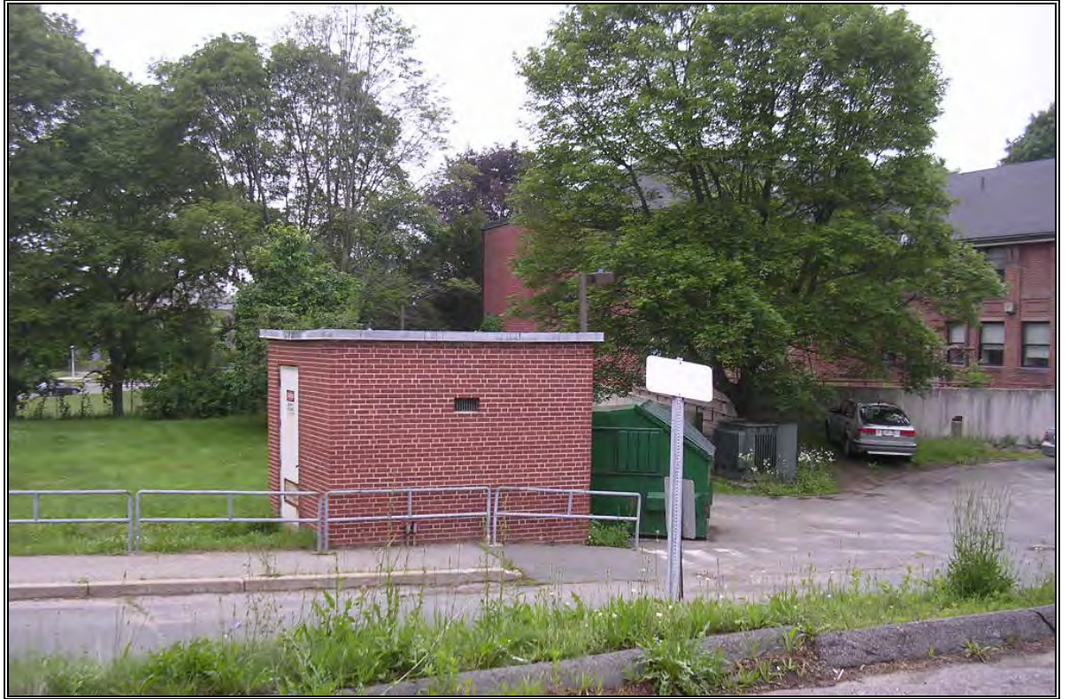
Photo Number 29: Transformer house between North Building (right) and Old Activities Center (not shown).
