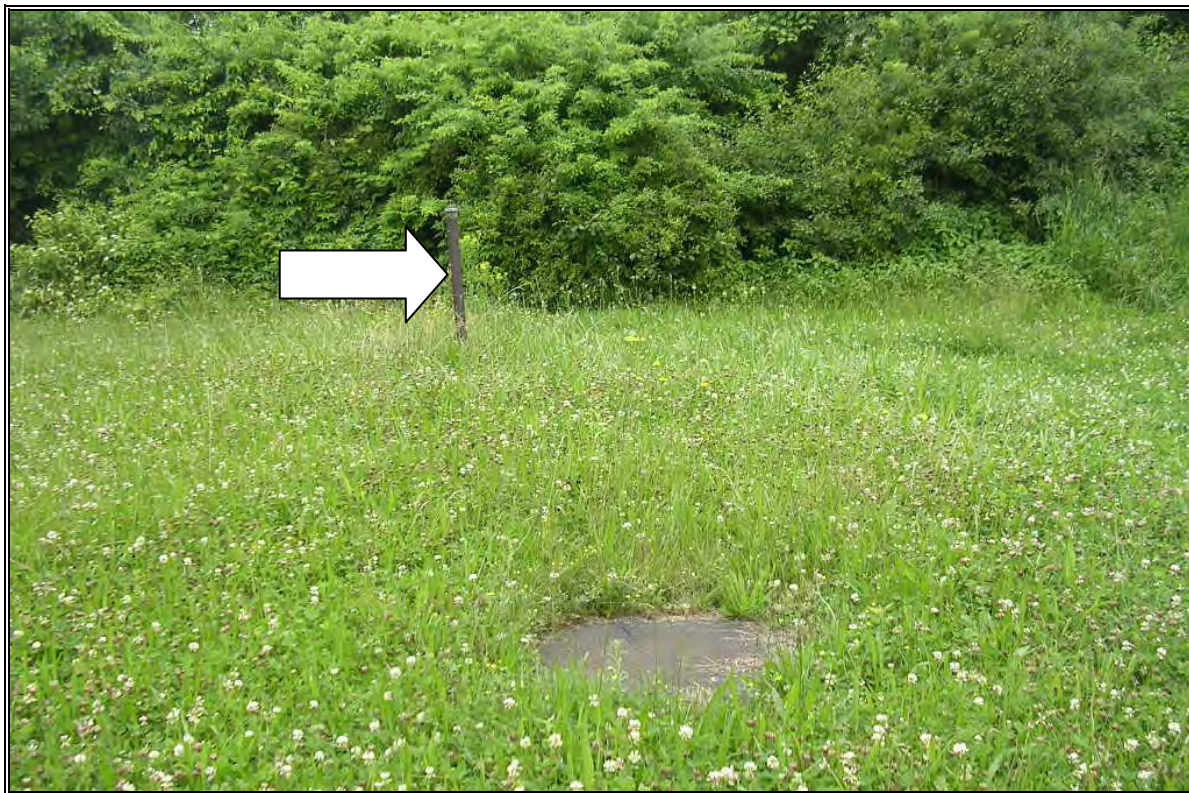
Photo Number 11: UST (5U) fill pipe and manhole access to tank in lawn south of Site 5.
