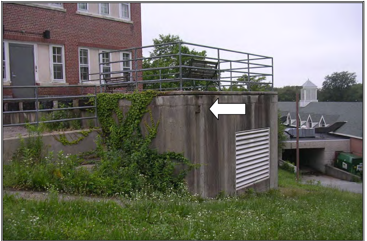
Photo Number 4: Thom Building AST vent pipe on north side of building.
