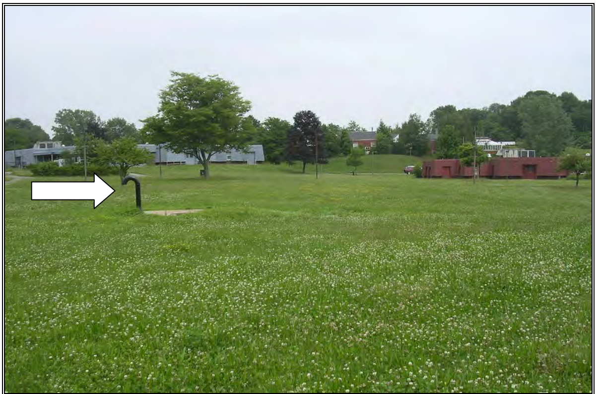
Photo Number 16: Vent pipe for underground hot water pipe system in Cottage Complex.
