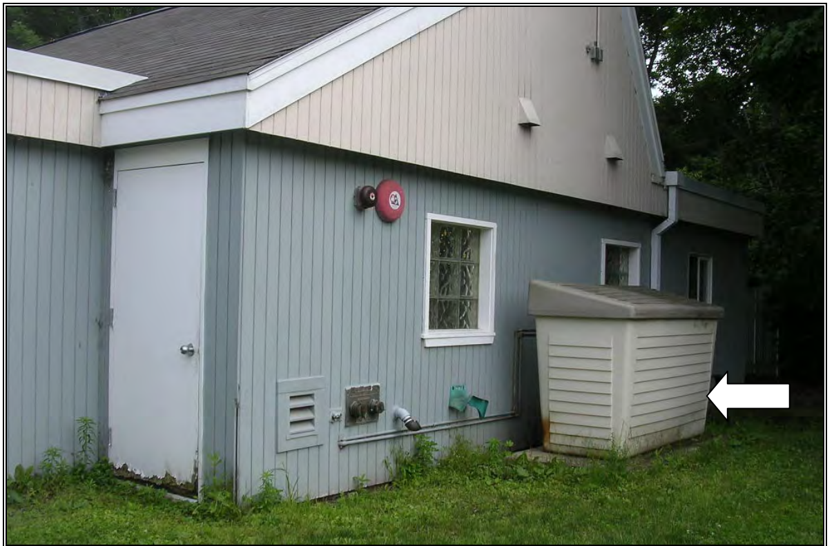
Photo Number 18: Fuel oil AST enclosure outside ICF 24 (8A).
