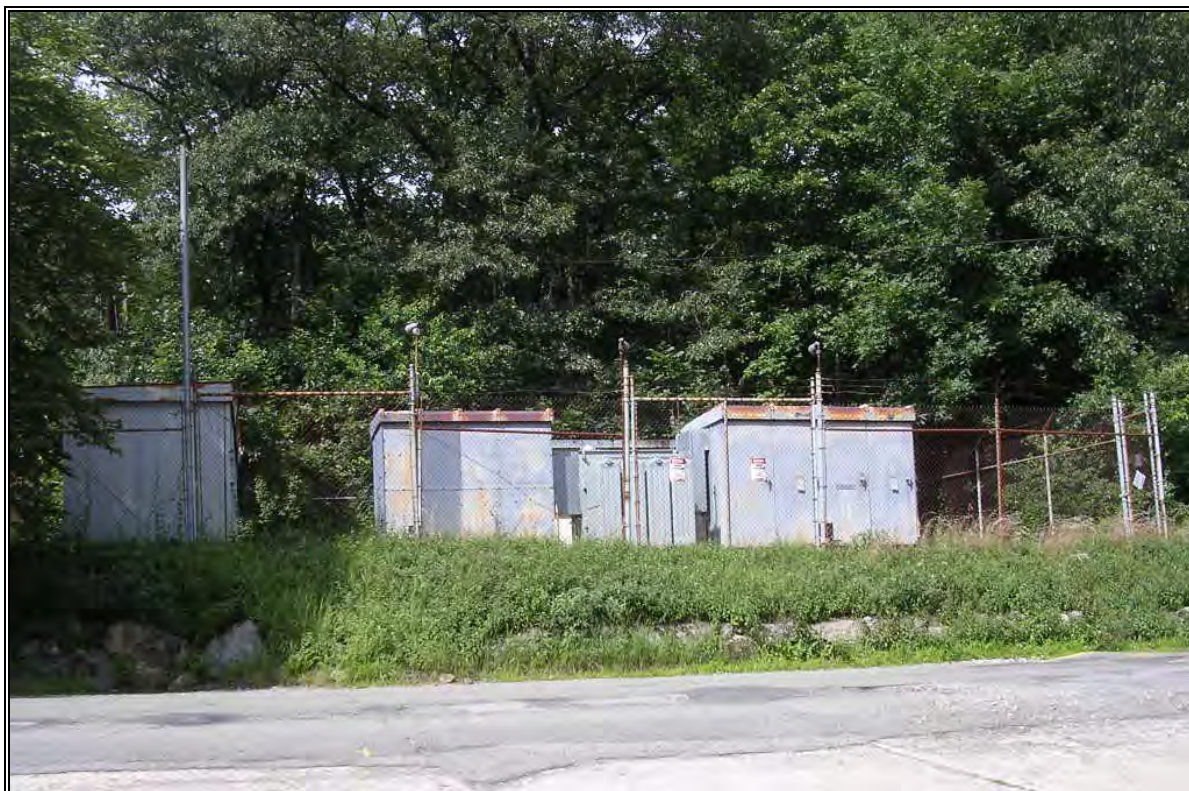
Photo Number 52: Main Transformer Yard east of Power Plant.
