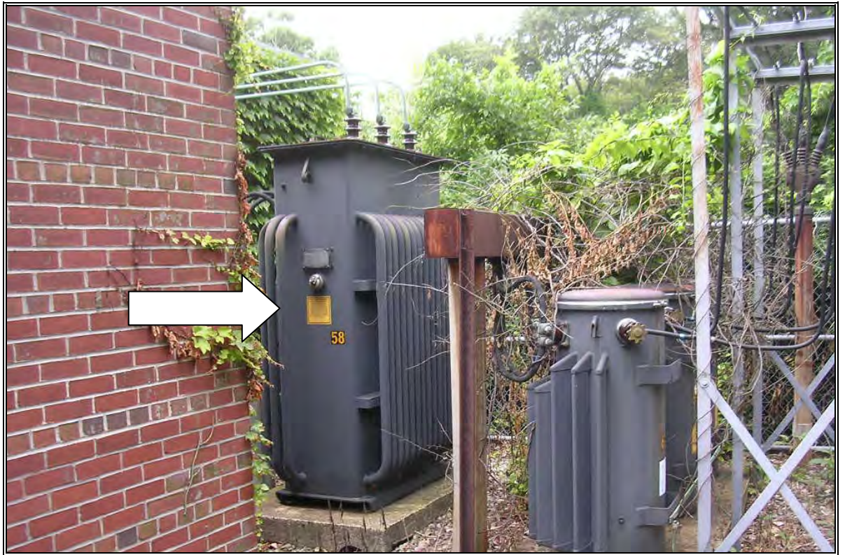
Photo Number 7: View of transformers on pad in Building 55 transformer yard. Note PCB label.
