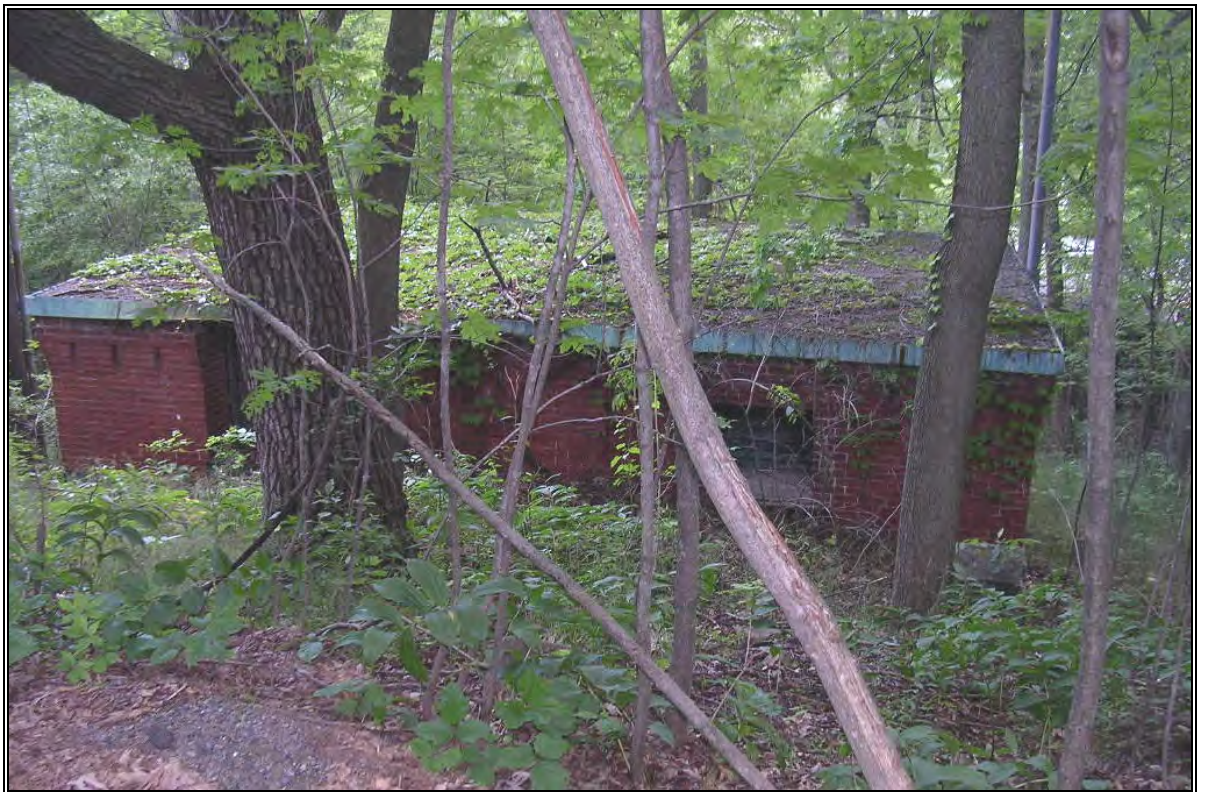
Photo Number 36: Building 14 containing transformers on hillside West of Stephen Bowen Hall.
