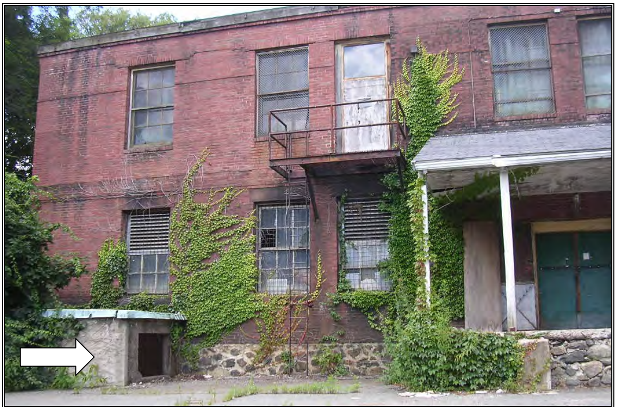
Photo Number 40: Southwest wall of Store Room and open steam pipe vault (on left).
