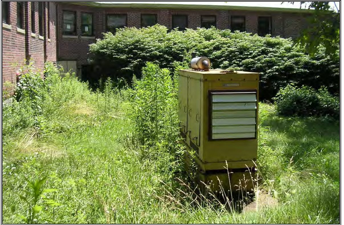
Photo Number 35: Diesel generator and AST (12A) on south side of Wallace Building
