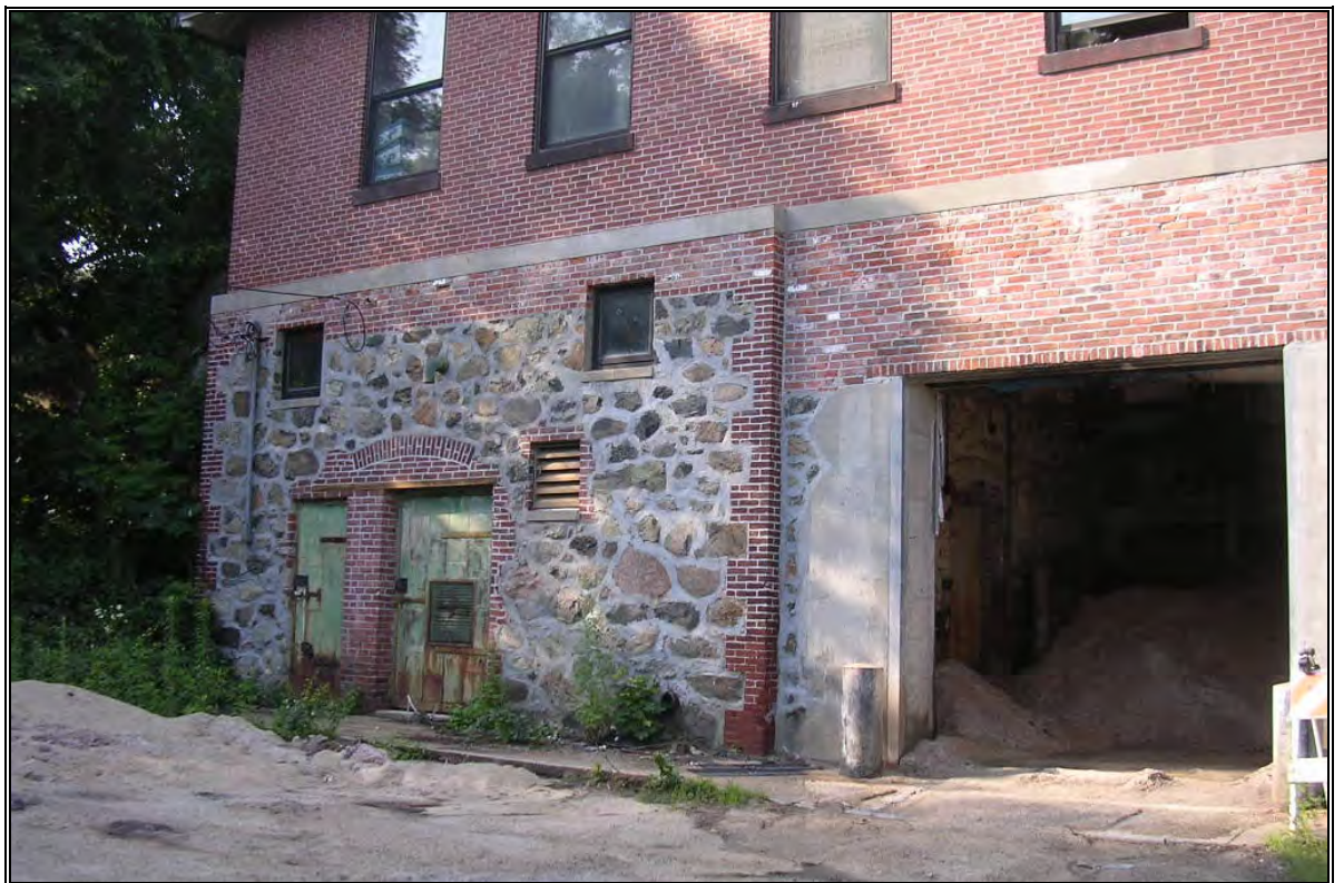
Photo Number 24: South (rear) wall of Belmont House and road salt in garage.
