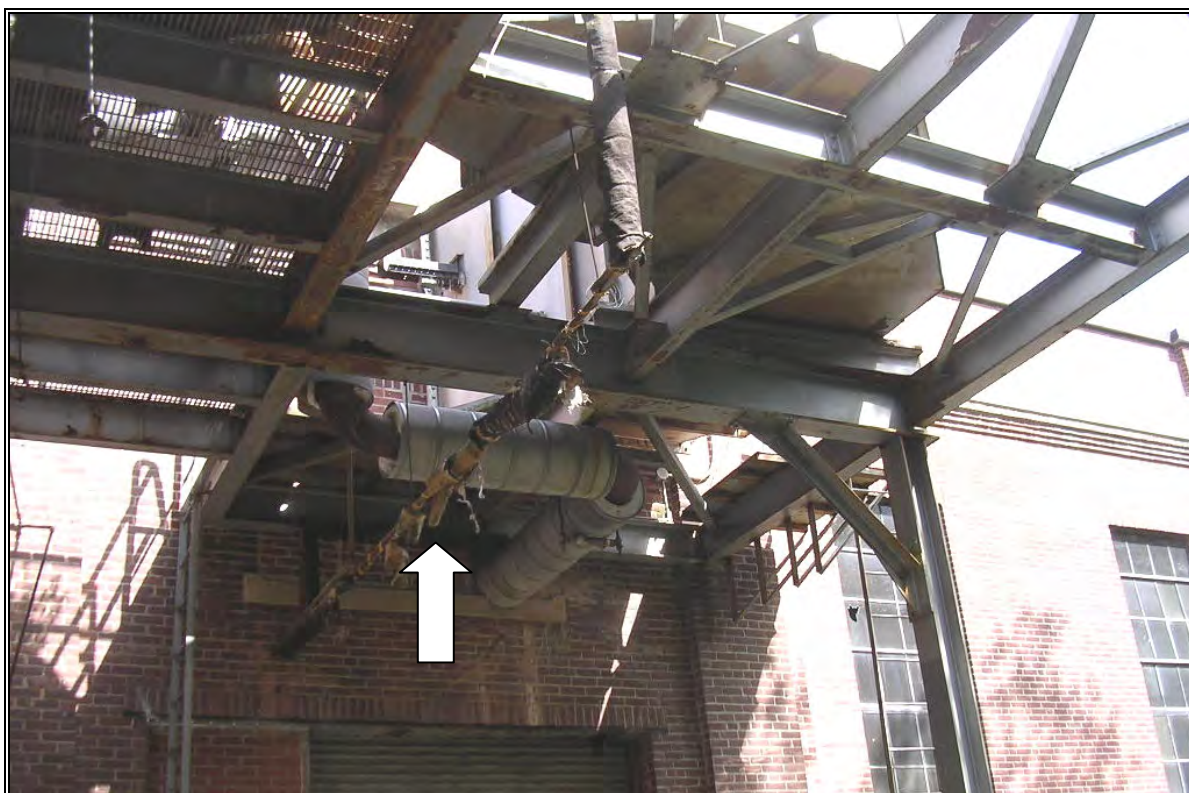
Photo Number 54: Damaged pipe insulation on northwest side of Power Plant.
