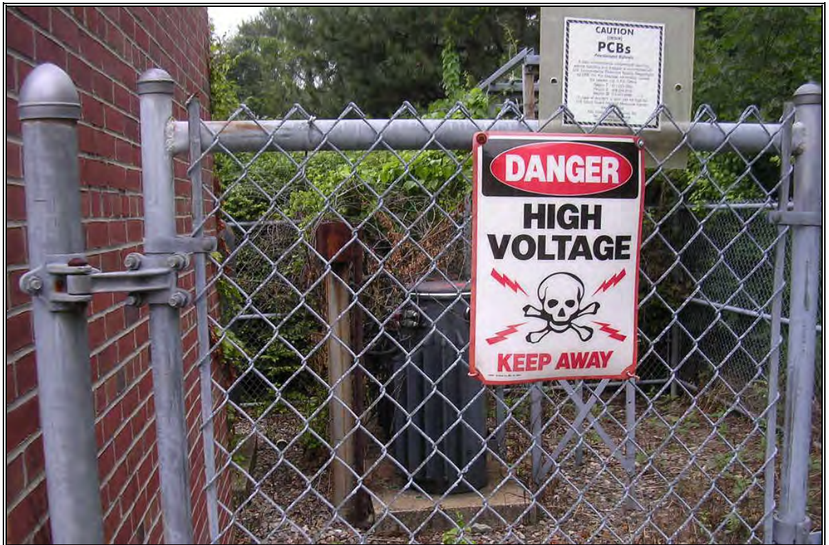
Photo Number 6: View of PCB sign in transformer yard north of Building 55.
