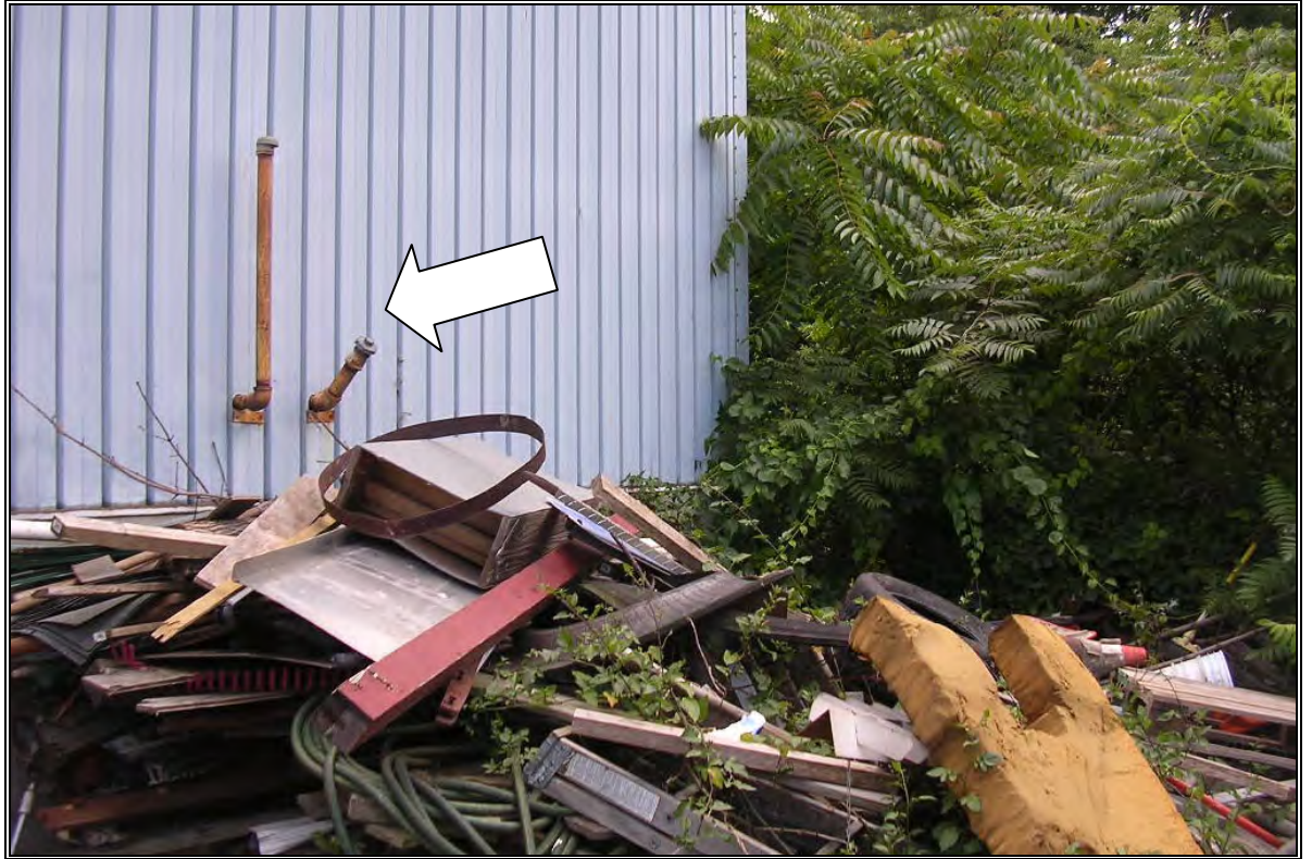
Photo Number 47: AST Fill and vent pipe and debris pile next to Farm and Grounds Department building
