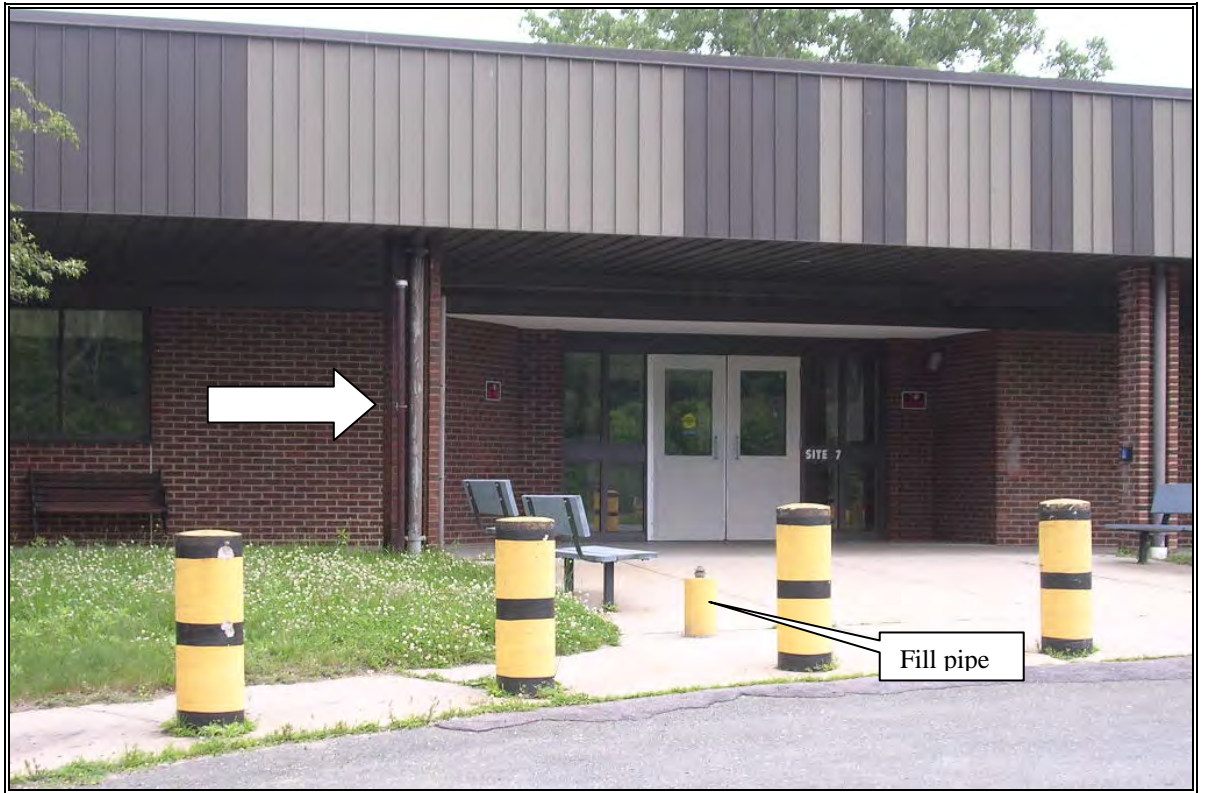
Photo Number 15: UST (6U) fill and vent pipes outside entrance to Site 7.
