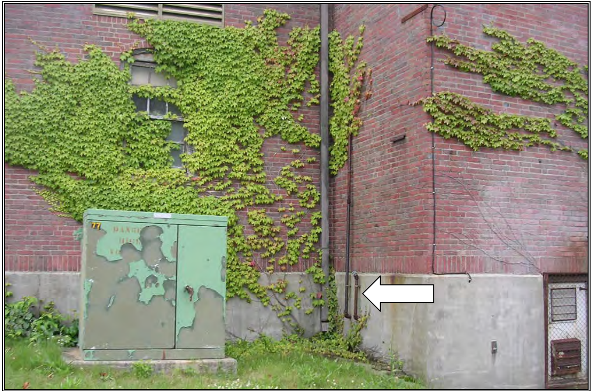
Photo Number 3: Howe Hall AST fill and vent pipe on northwest side of building.
