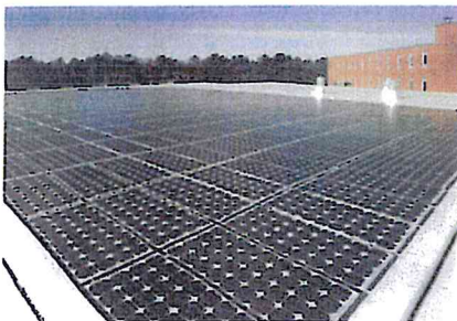
Photovoltaic Panels Supplement Conventional Fuel Sources Turners Falls High School
