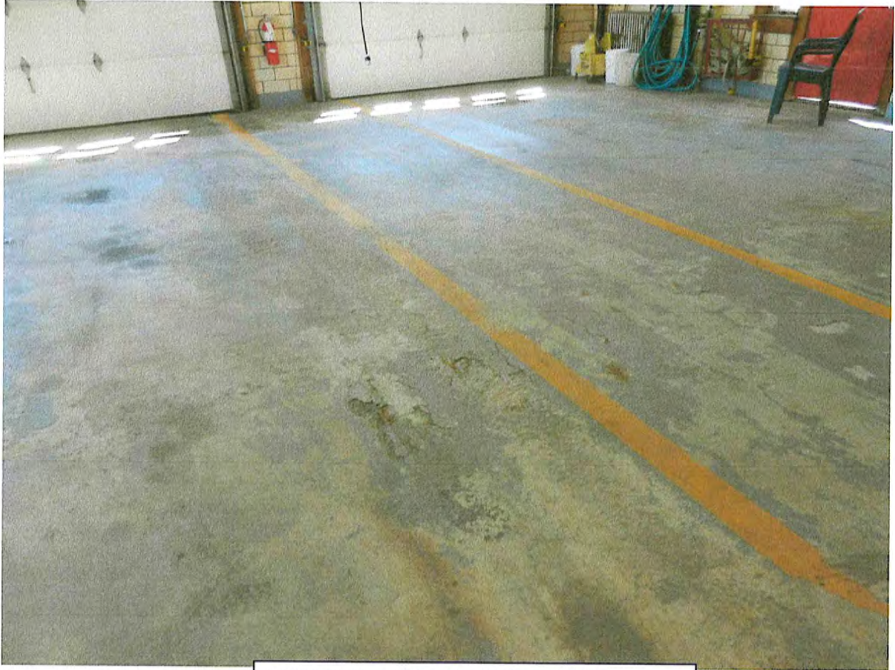
MINOR CONCRETE SPALLS WITH EXPOSED REBAR AND MISC. MAP CRACKS PHOTO-8
