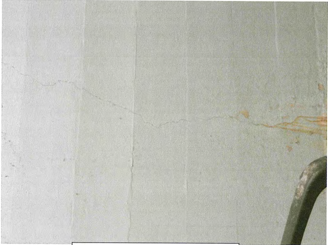
CONCRETE WALL HORIZONTAL CRACK WITH WATER STAIN PHOTO-13
