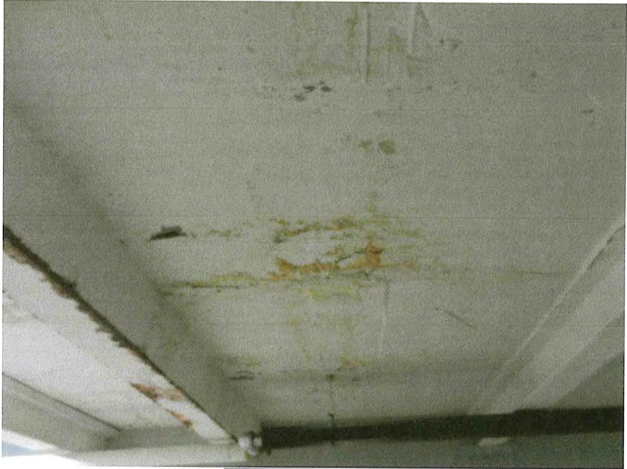
LONGITUDINAL CONCRETE CRACK IN SECOND BAY FROM FRONT WALL AND RUSTED STEEL BEAM BIOTTOM FLANGE
