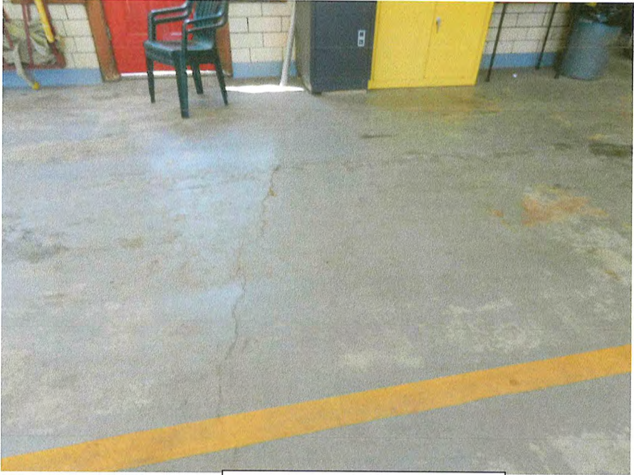
TRANSVERSE CRACK IN CONCRETE SLAB W/RUST STAIN IN VARIOUS LOCATIONS PHOTO-11
