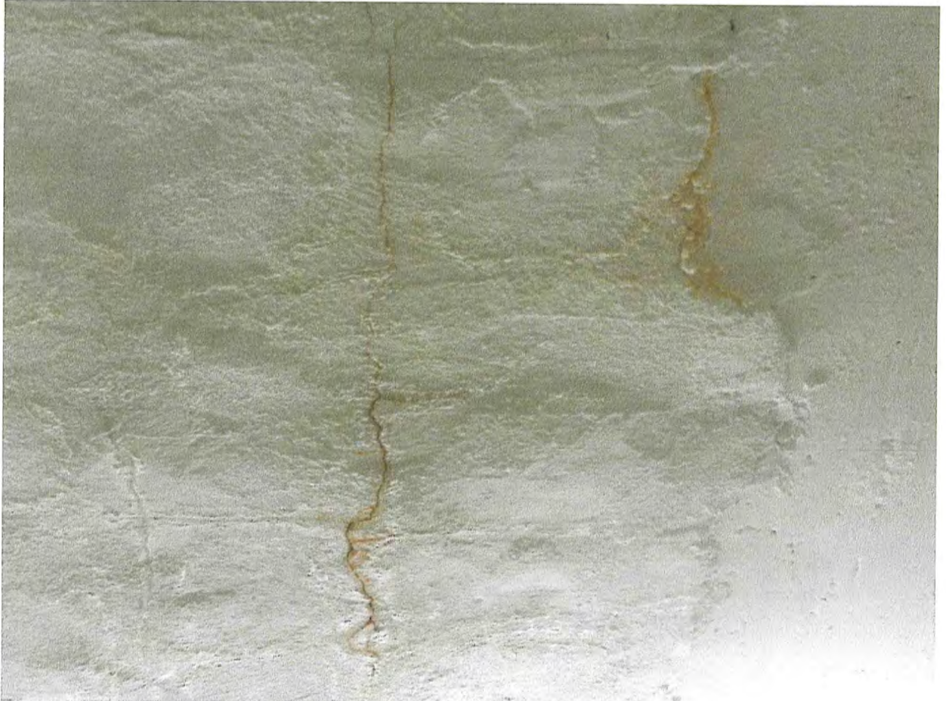
CONCRETE PATCH ON UNDERSIDE OF SLAB WITH LONGITUDINAL CRACK-LEFT SIDE
