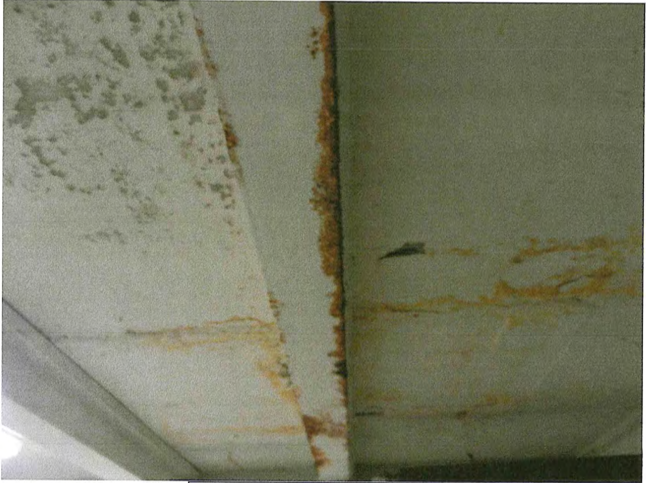
UNDERSIDE OF SLAB WITH LONGITUDINAL CRACK AND RUSTED BOTTOM FLANGE PHOTO-19
