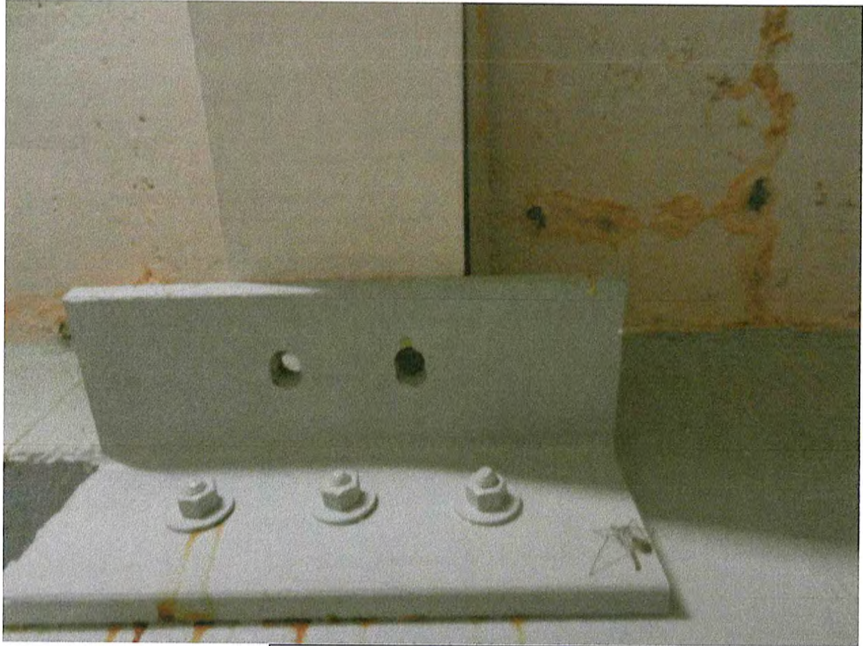
W8 BEAM WITH CONNECTION BOLTS MISSING AT SUPPORT PHOTO-20
