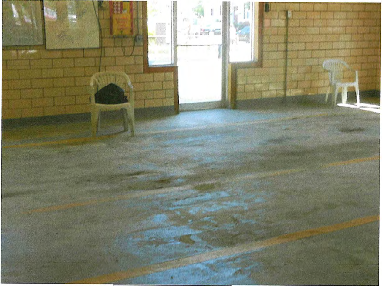
MINOR CONCRETE SPALL PHOTO-9
