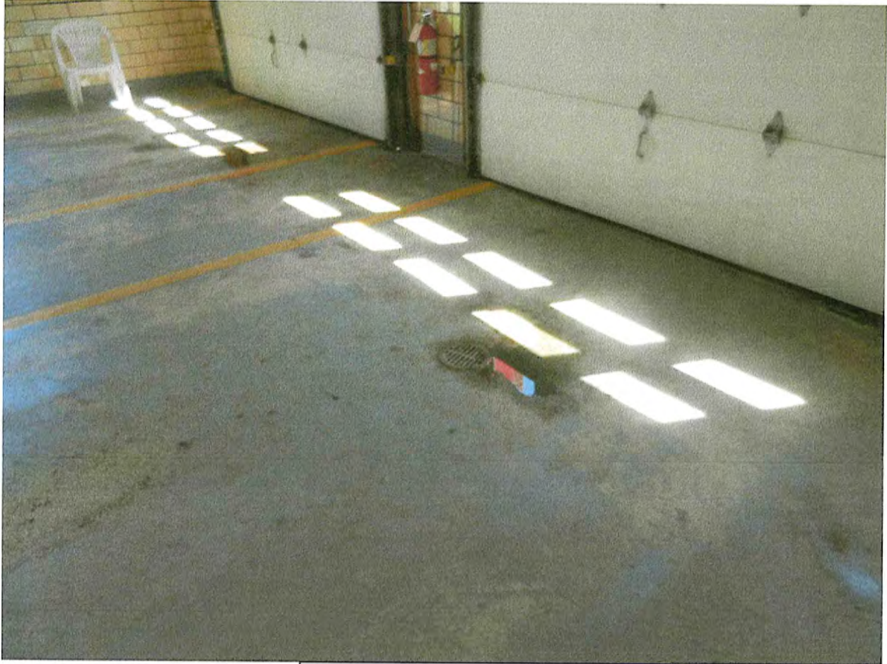
EXISTING FLOOR DRAINS AT ENTRANCE DOORS PHOTO-12
