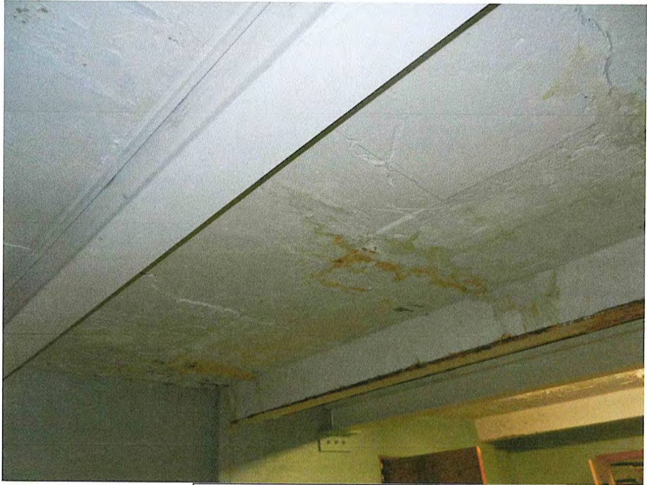
3rd BAY FROM FRONT WALL WITH W8 BEAM, CONCRETE CRACK WITH RUST AND WATER STAIN. PHOTO-17
