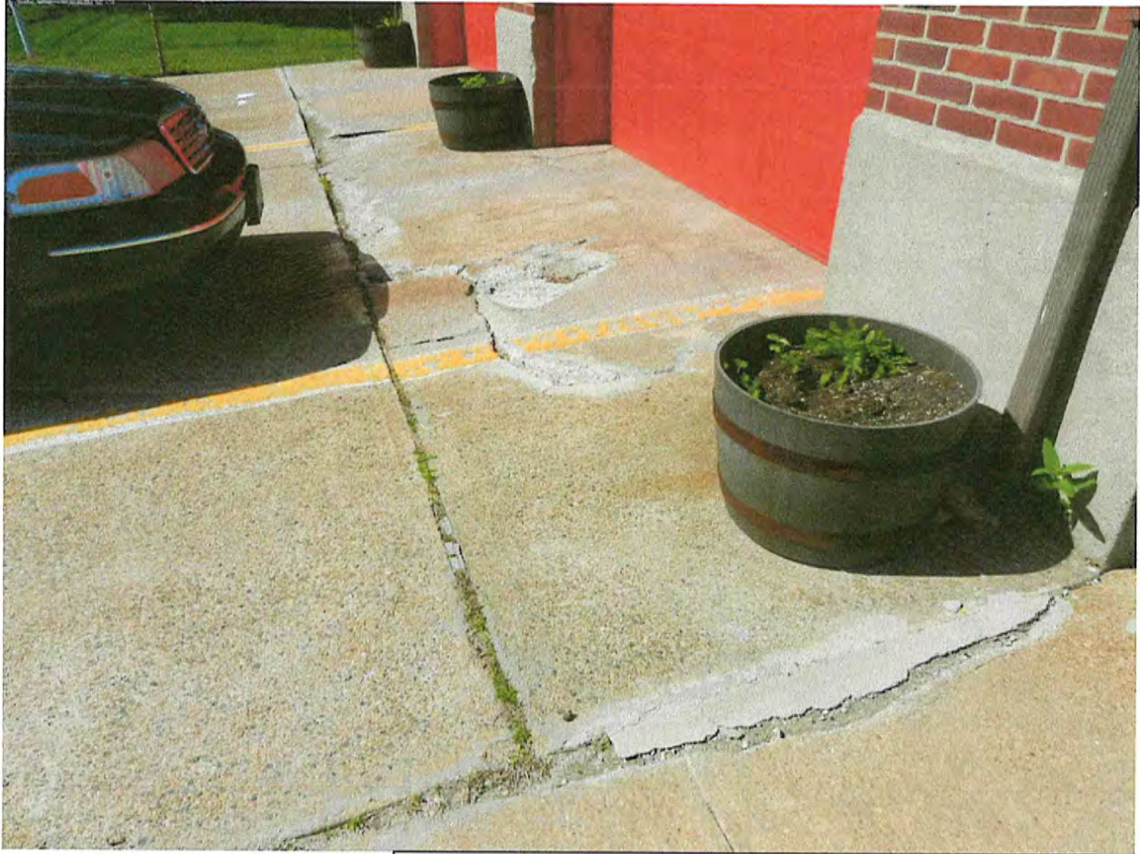
PROSPECT STREET FIRE STATION ENTRANCE DRIVEWAY DETERIORATED CONCRETE PHOTO-4
