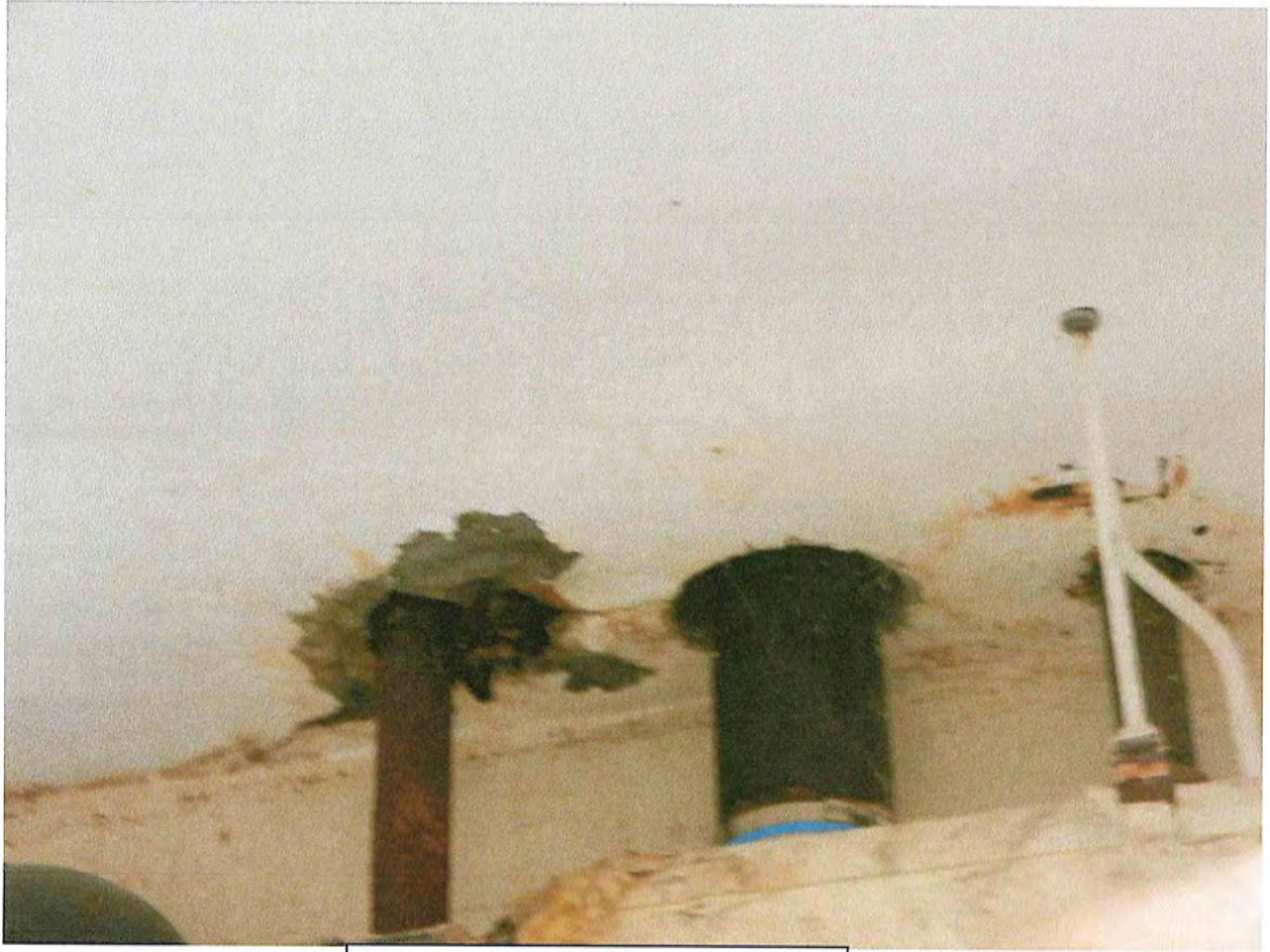
CONCRETE SPALLS WITH RUST STAIN AROUND FLOOR DRAIN PHOTO-23
