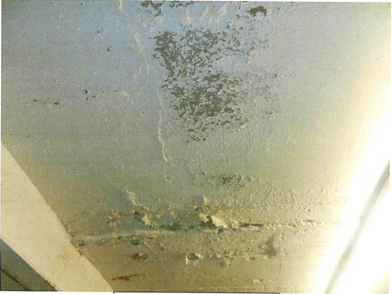
CONCRETE CRACK ON UNDERSIDE OF SLAB AND MINOR SPALL PHOTO-21
