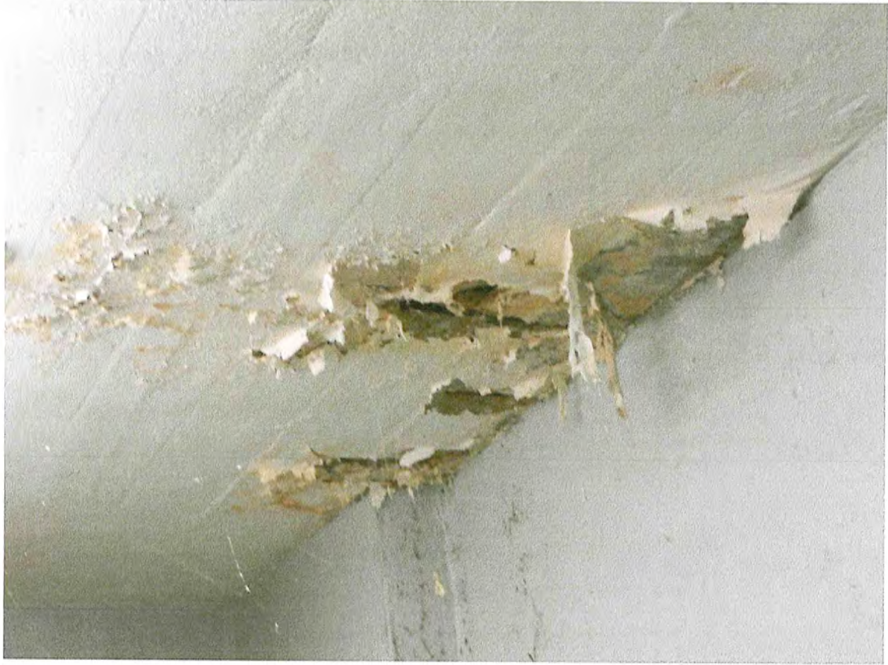
UNDERSIDE OF SLAB FRONT WALL CONCRETE SPALLS WITH EXPOSED RUSTED REBARS AND WATER STAIN
