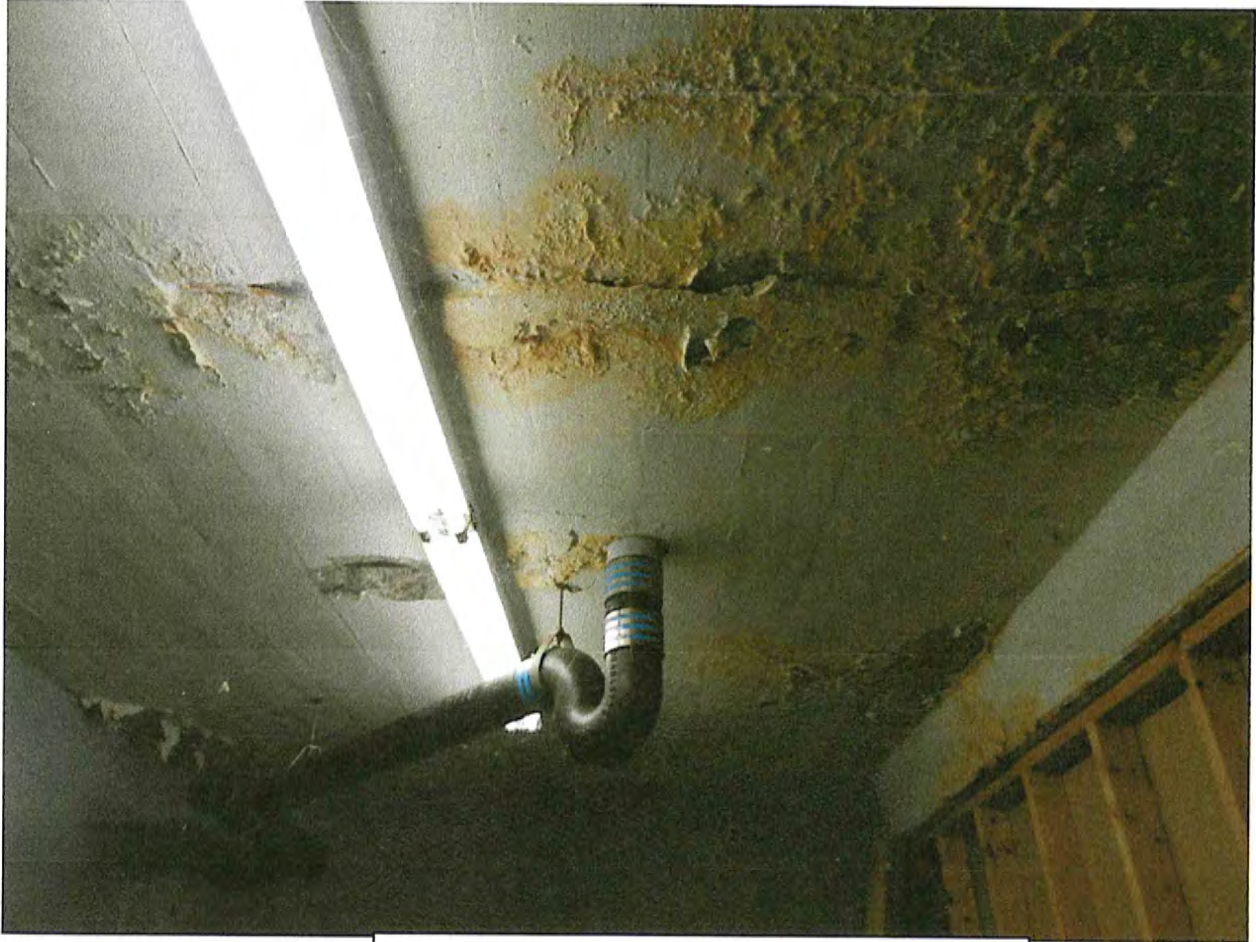
SECOND BAY FROM FRONT WALL, CRACK IN CONCRETE SLAB WITH RUST STAIN, SPALLS WITH RUSTED REBAR AND W8 BEAM SET BETWEEN 1 ST & 2 ND ORIGINAL STEEL BEAMS PHOTO-16
