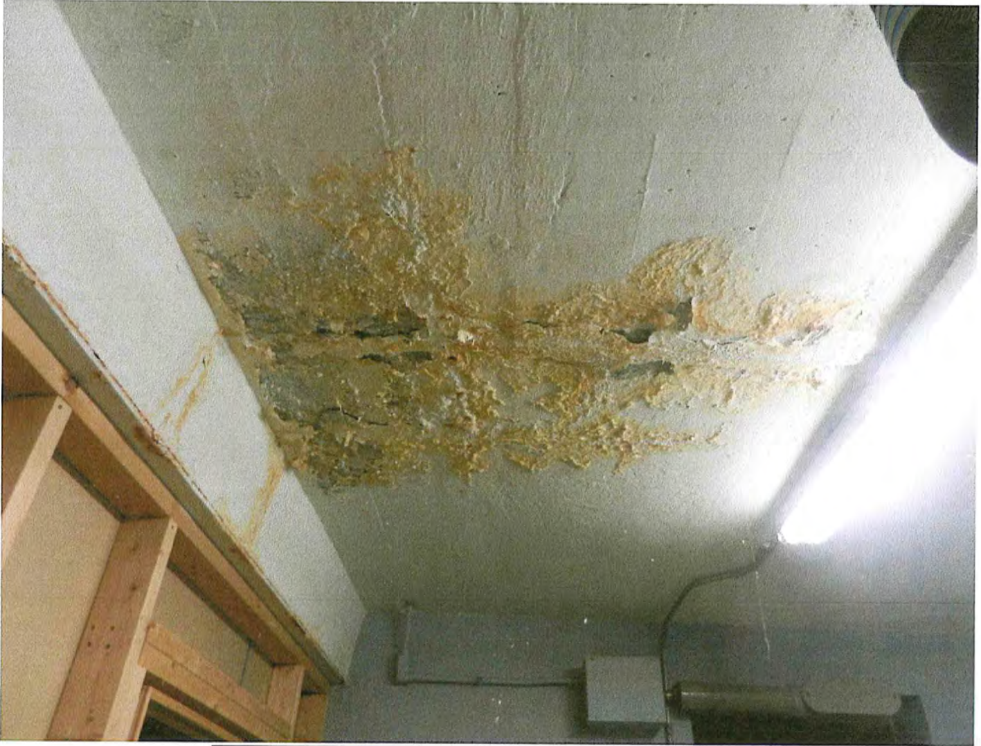
FIRST BAY FROM FRONT WALL RIGHT SIDE OF BASEMENT AREA SPALL ED CONCRETE WITH WATER AND RUST STAIN AND MINOR RUST IN BEAM BOTTOM FLANGES PHOTO-15
