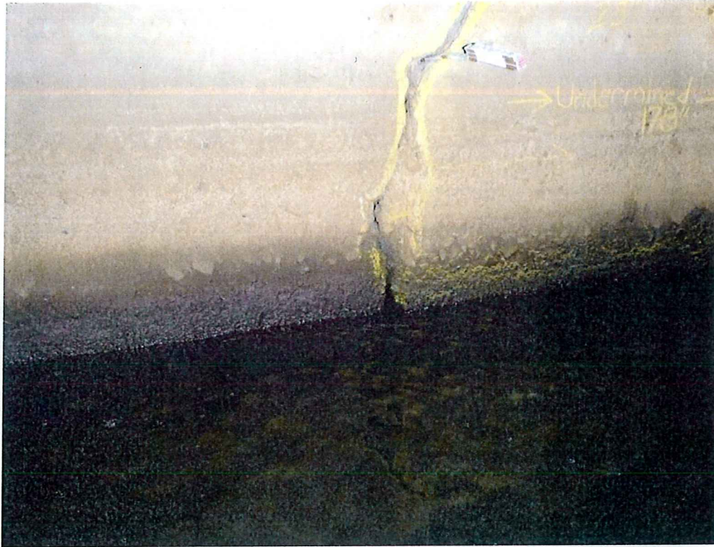
Photo 11: South wall has a 1" displacement at water line
