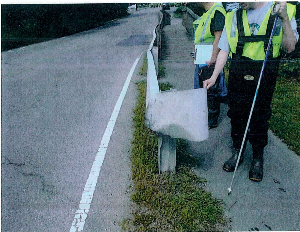
Photo 34: Southeast guardrail end showing impact damage
