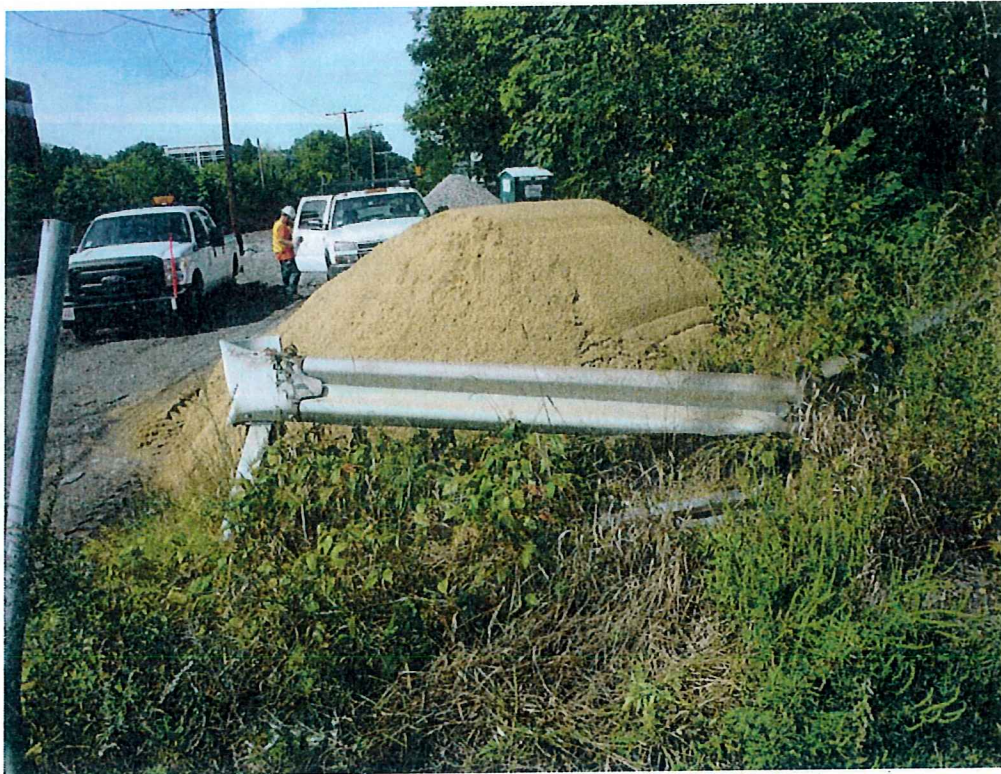
Photo 33: Impact damage to the Southwest approach guardrail
