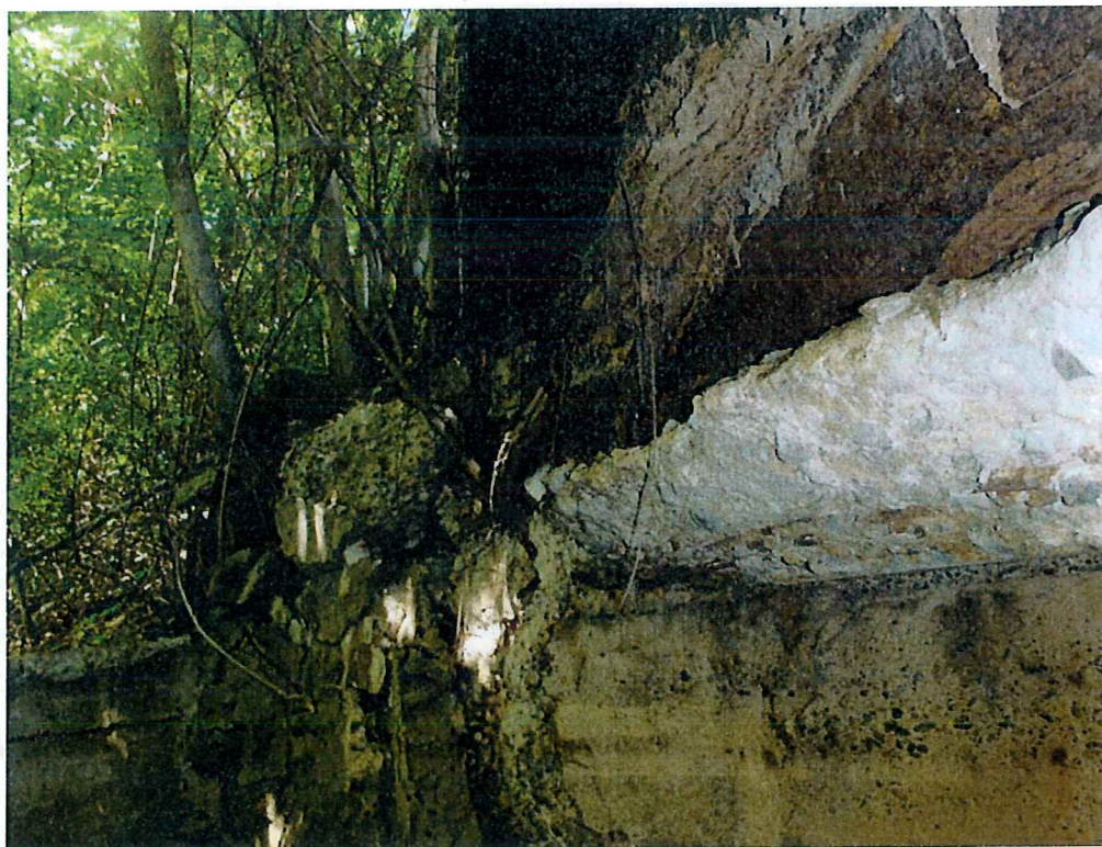
Photo 26: Tree root & corrosion on 12" CI pipe, Northwest corner
