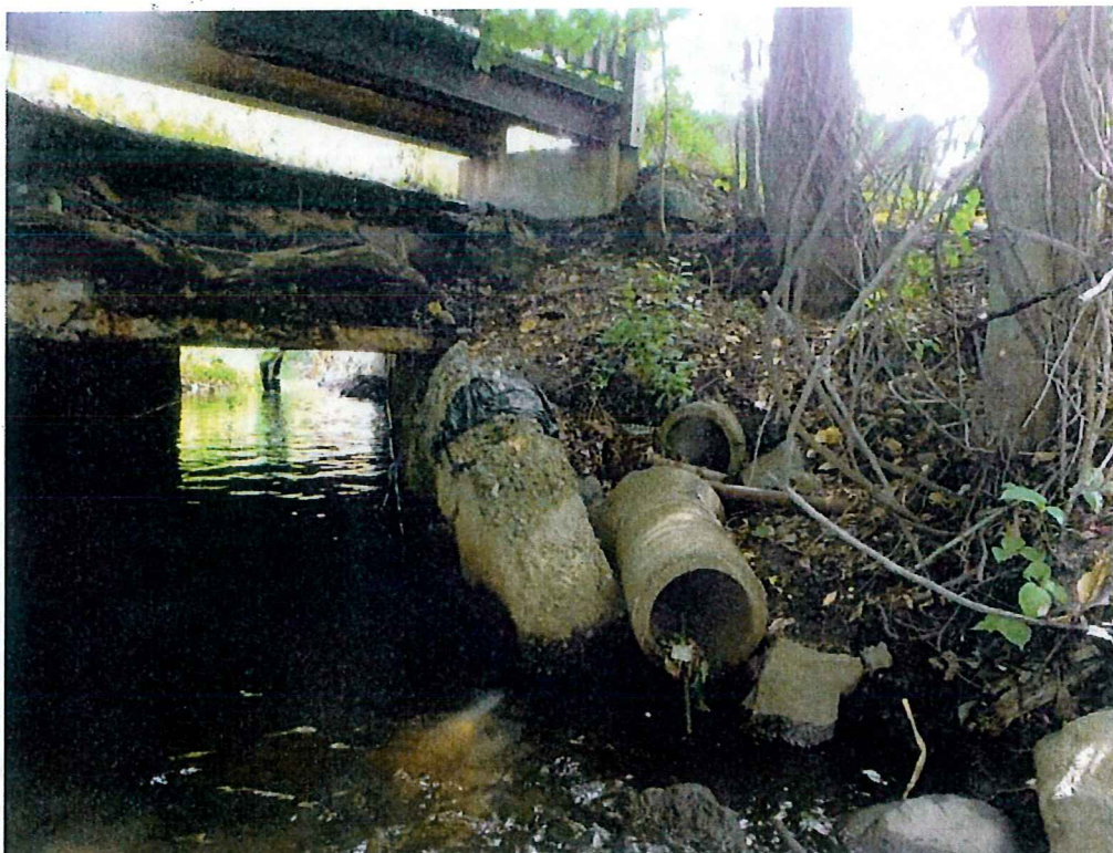
Photo 24: Significant erosion and undercutting of the embankment at the Southwest corner
