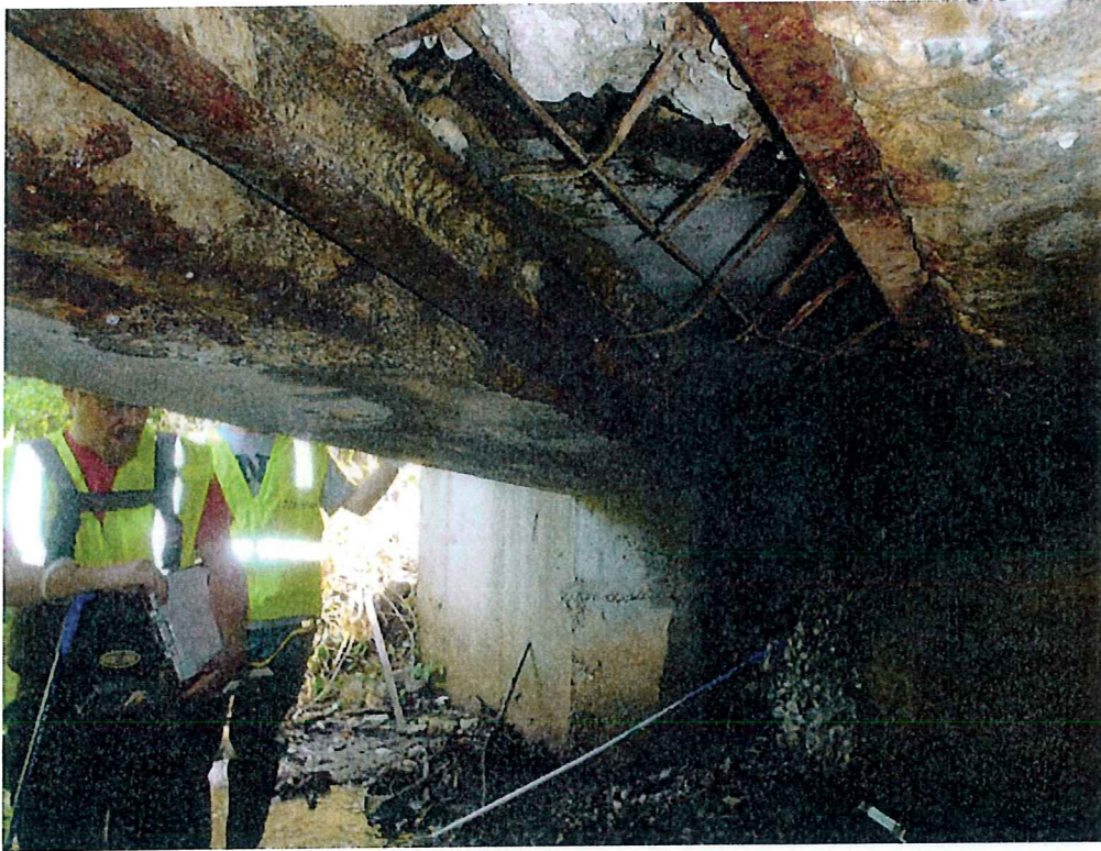
Photo 1: Hole in the East side of the roof looking towards the South wall showing unsupported railroad rail and corroded reinforcement
