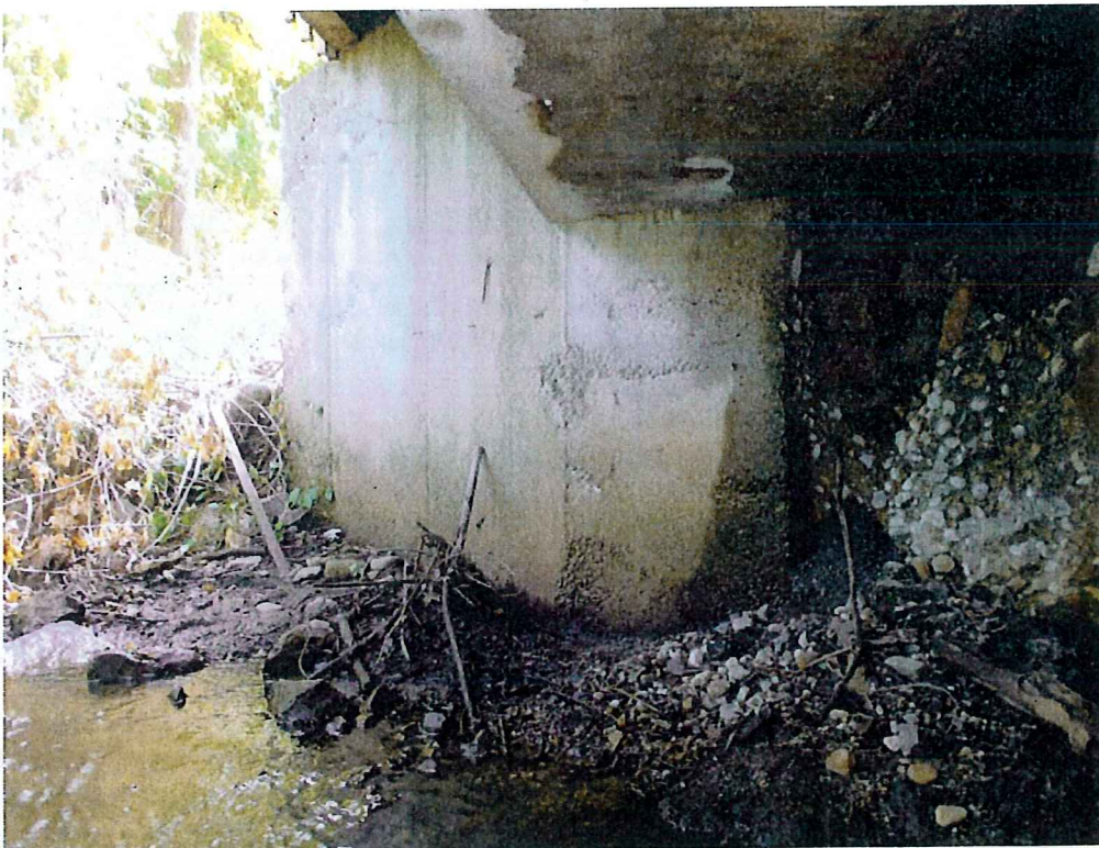
Photo 22: Erosion at the Southeast corner, backfill material is washing out from behind wingwall and South wall
