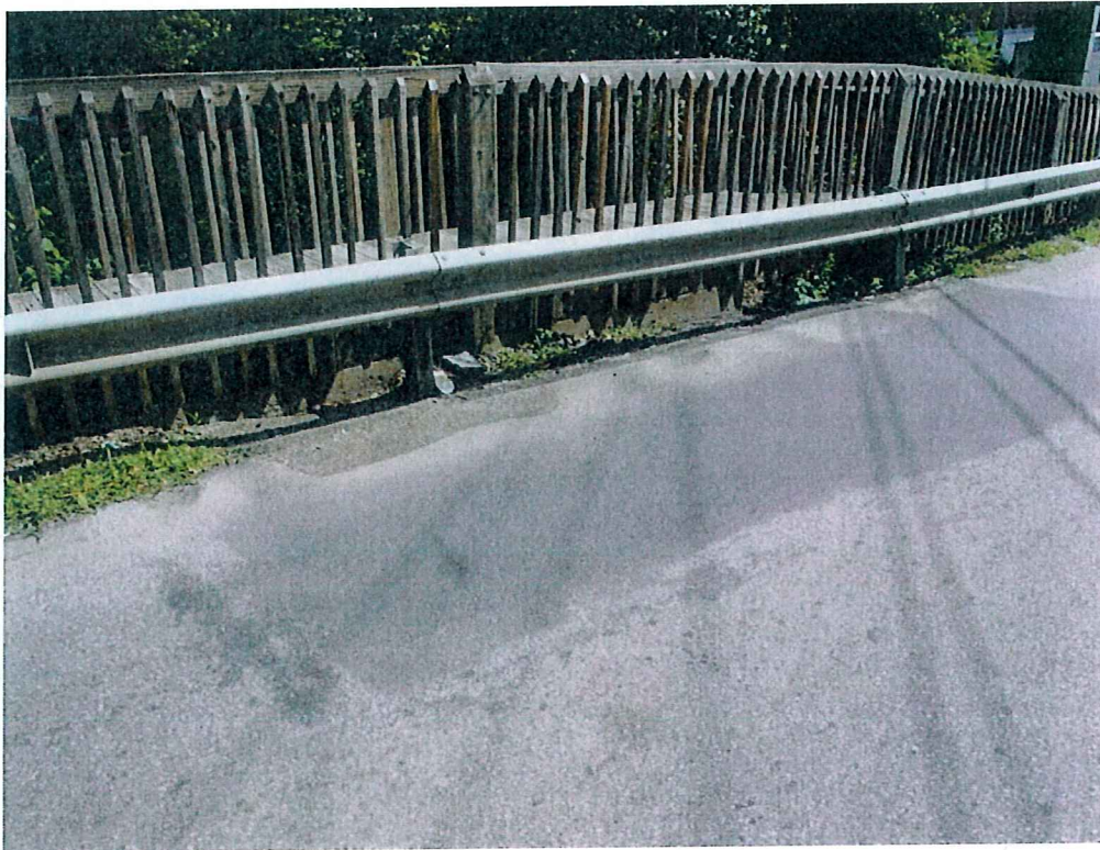
Photo 29: Type SS guardrail at the East side of the Northbound travel lane showing excessive post spacing and bent posts
