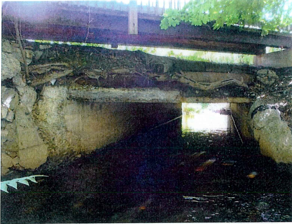
Photo 27: Tree root spans the entire West edge of the culvert is retaining the 12" CI utility pipe
