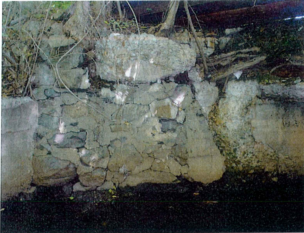
Photo 19: Northwest wingwall is undermined and leaning in towards the channel
