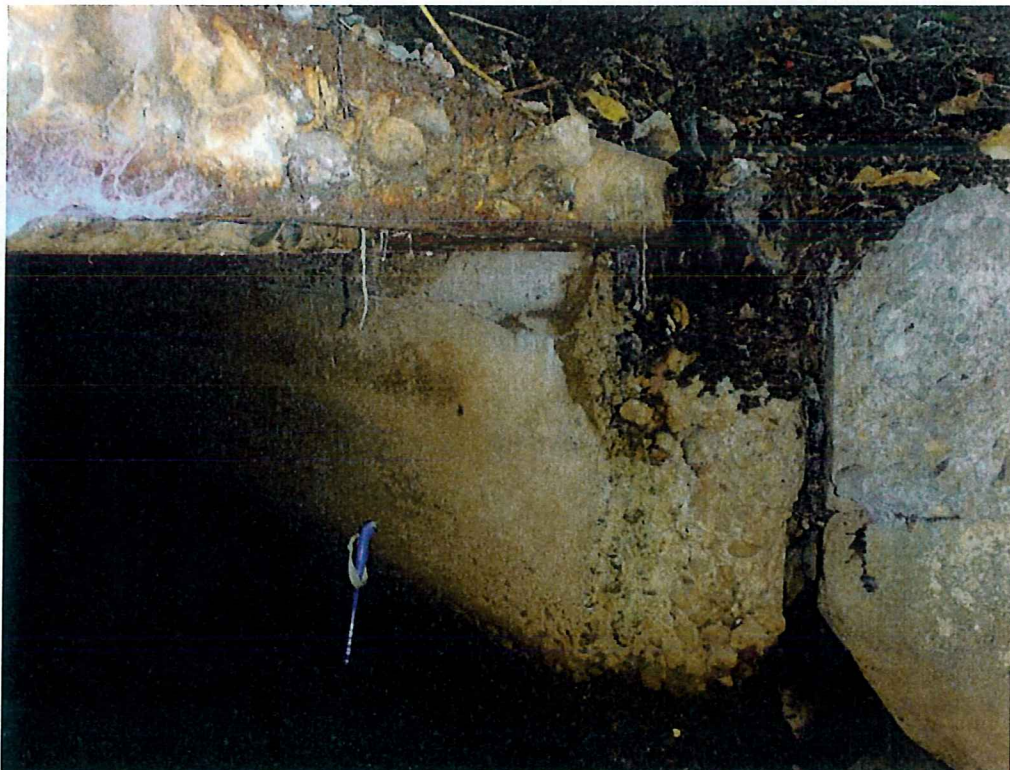
Photo 8: South west wingwall is spalled 16" wide x full height
