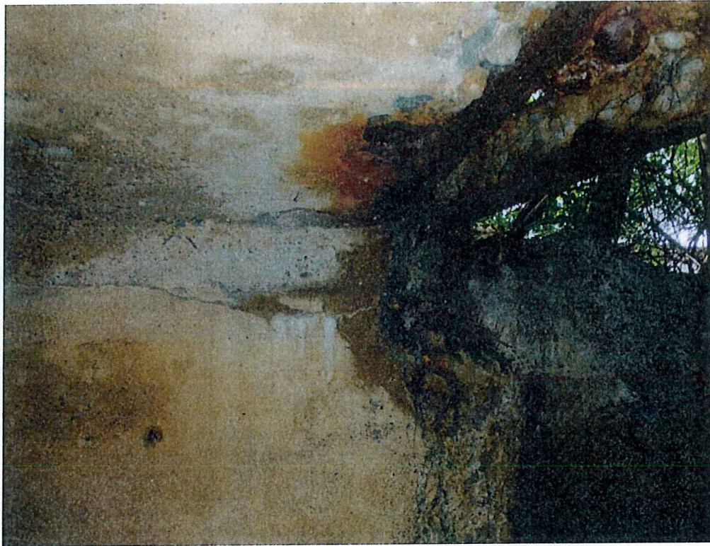
Photo 9: Unsupported rail at Southwest corner of South wall, top of wall is crushing for a length of 14"
