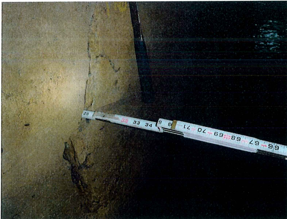
Photo 12: South wall has a crack up to 1-1/4" wide. Tape was able to penetrate wall 29"
