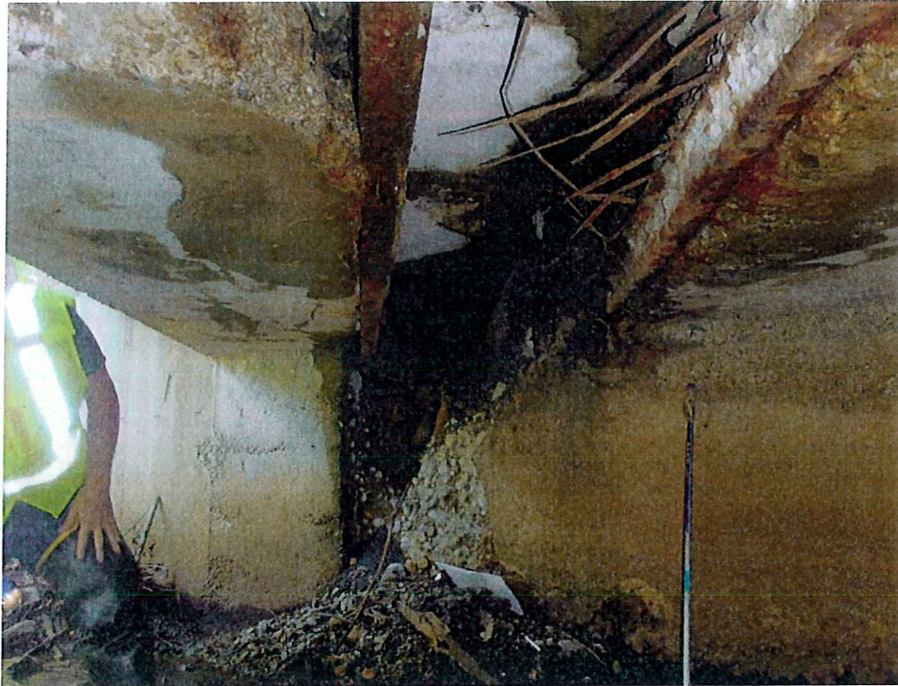
Photo 3: Hole in deck on the East end looking towards the South Wall
