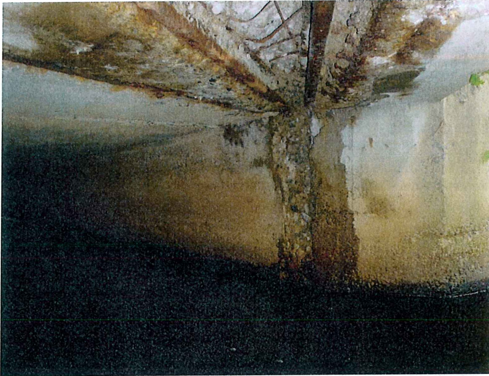
Photo 17: Spall at Eastern end of the North wall measuring 43" high x 14" wide x 7" deep with active leakage
