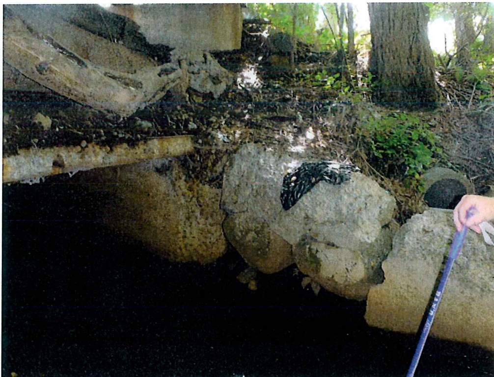
Photo 20: Southwest wingwall is undermined and leaning in towards channel
