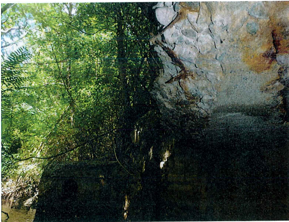
Photo 6: Northwest corner showing spalled edge of roof and corroded reinforcement
