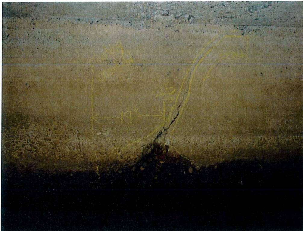
Photo 16: North wall has a full height crack; footing is exposed and undermined at this location
