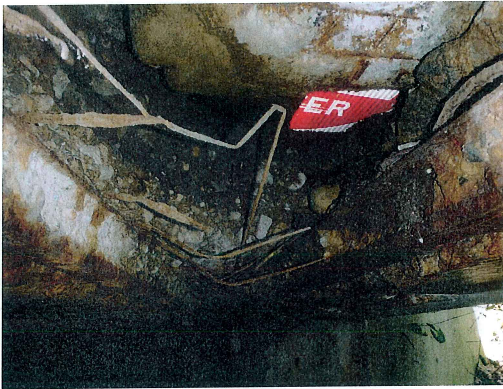
Photo 5: Hole on deck, East end looking towards the North wall
