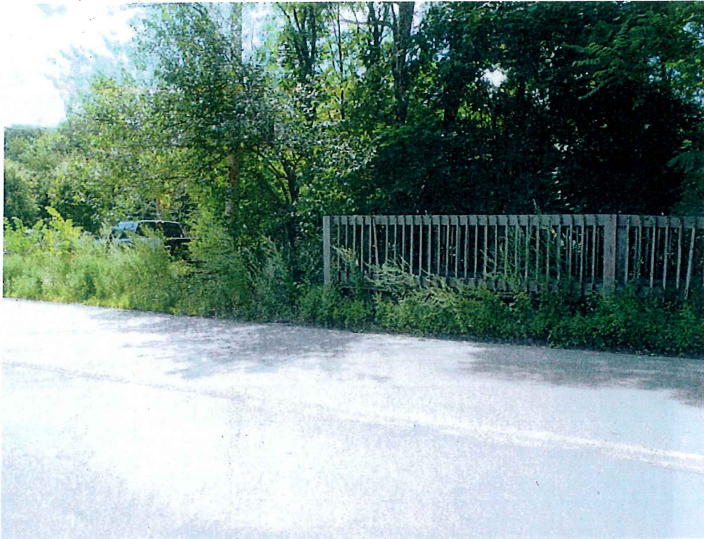
Photo 31: There is no bridge rail on the West side of the Southbound roadway
