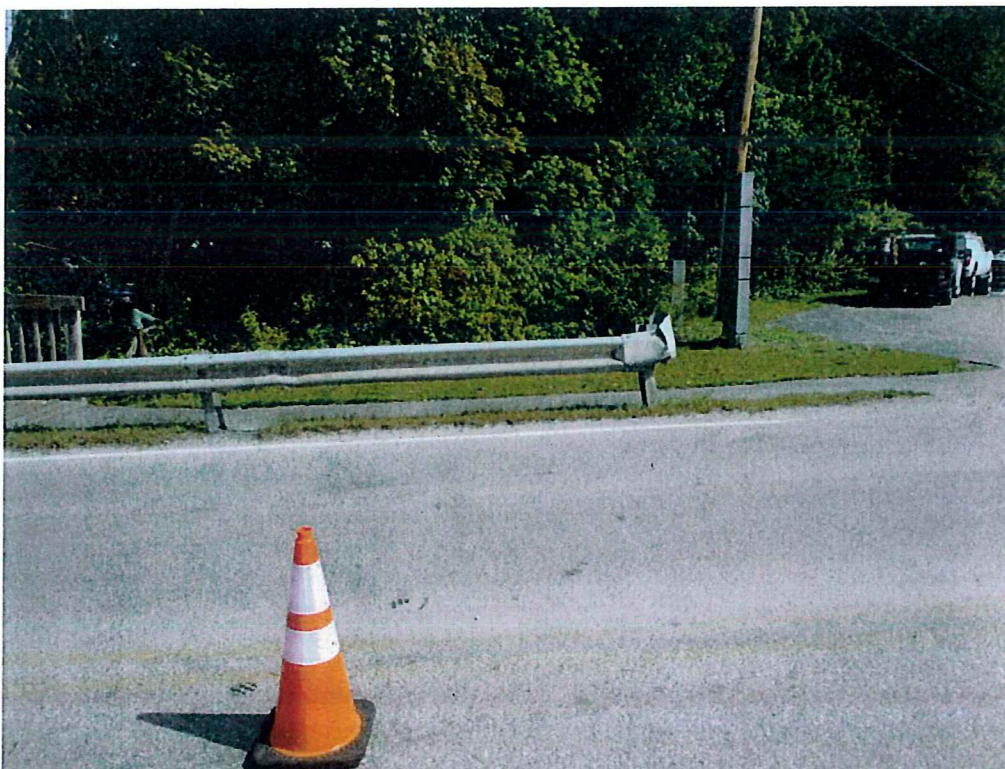
Photo 32: Impact damage to the Southeast approach guardrail showing excessive spacing and bent posts
