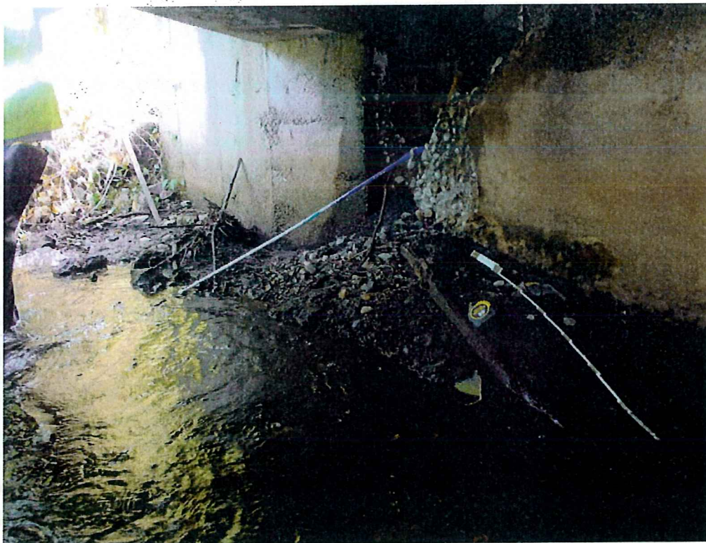
Photo 28: Aggradation at the Southeast corner is restricting the channel flow at the upstream side of the culvert
