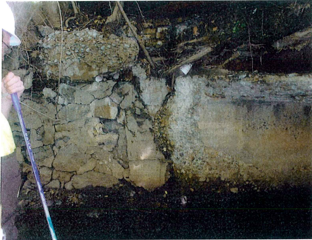
Photo 15: North wall has a full height spall at the Northwest corner
