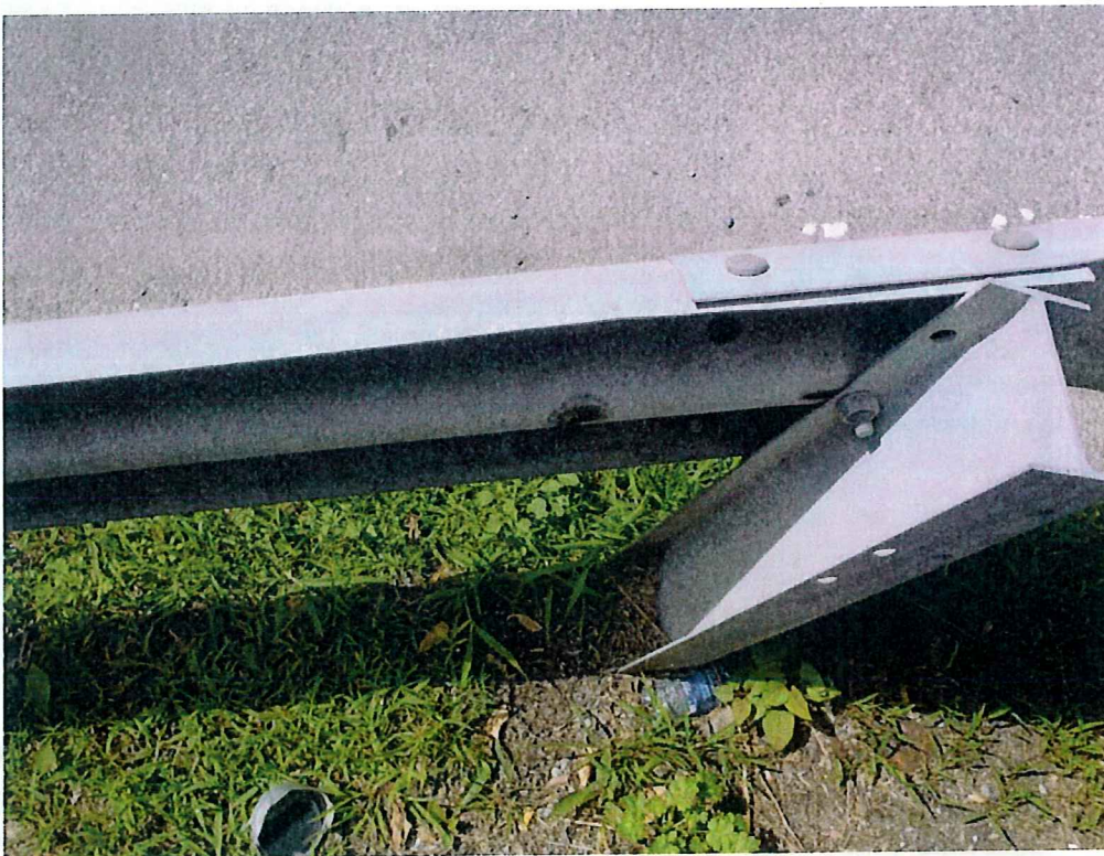
Photo 30: Typical bent guardrail post at the East side of the Northbound roadway
