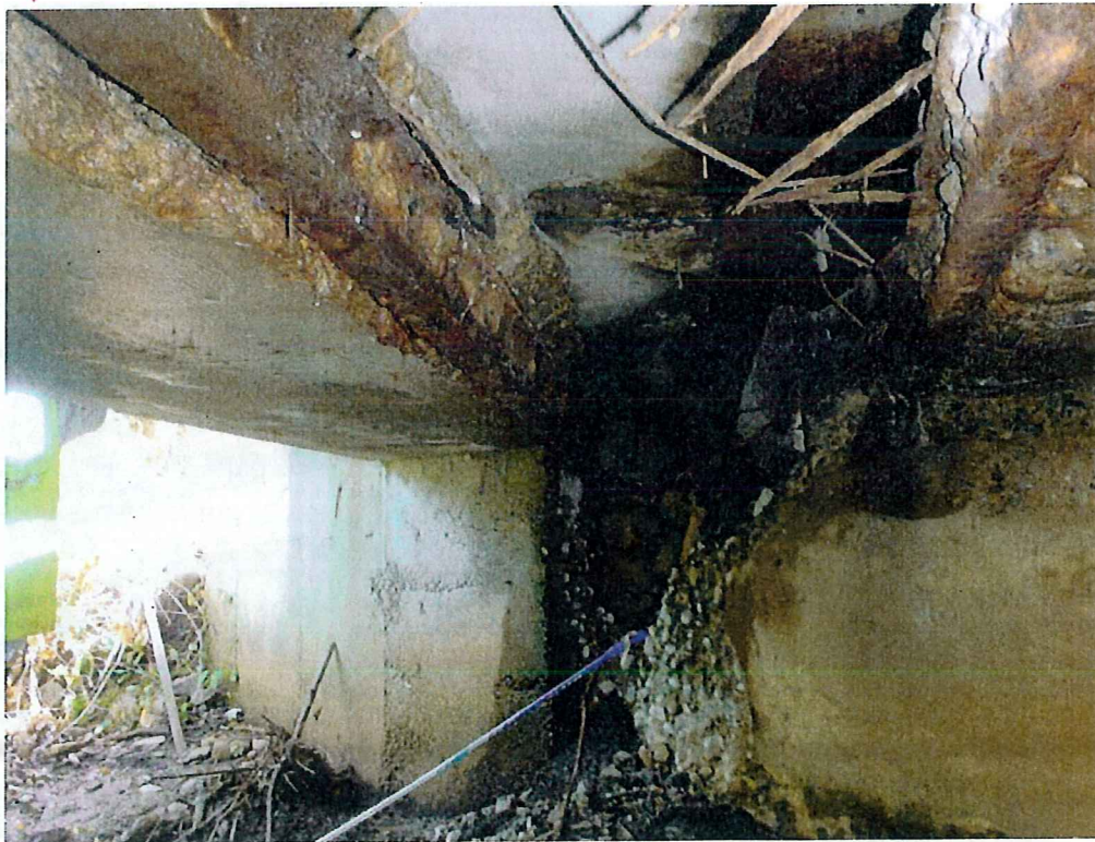
Photo 14: Large hole at the Southeast corner of the bridge in the South wall
