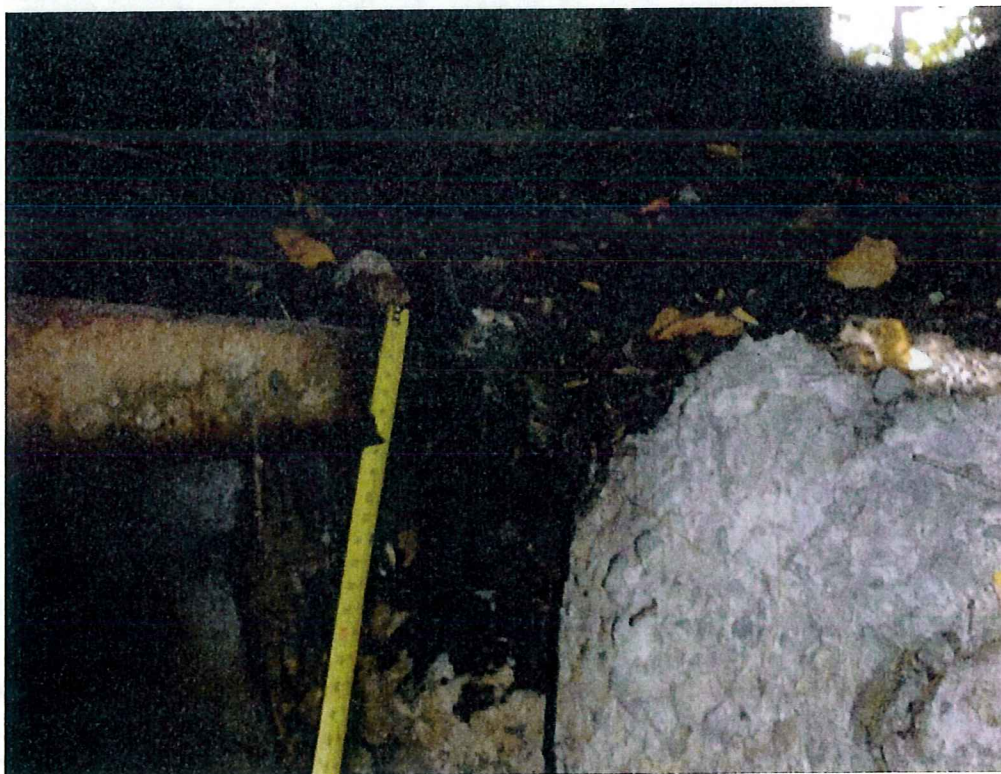
Photo 10: Unsupported rail at Southwest corner spall of South wall
