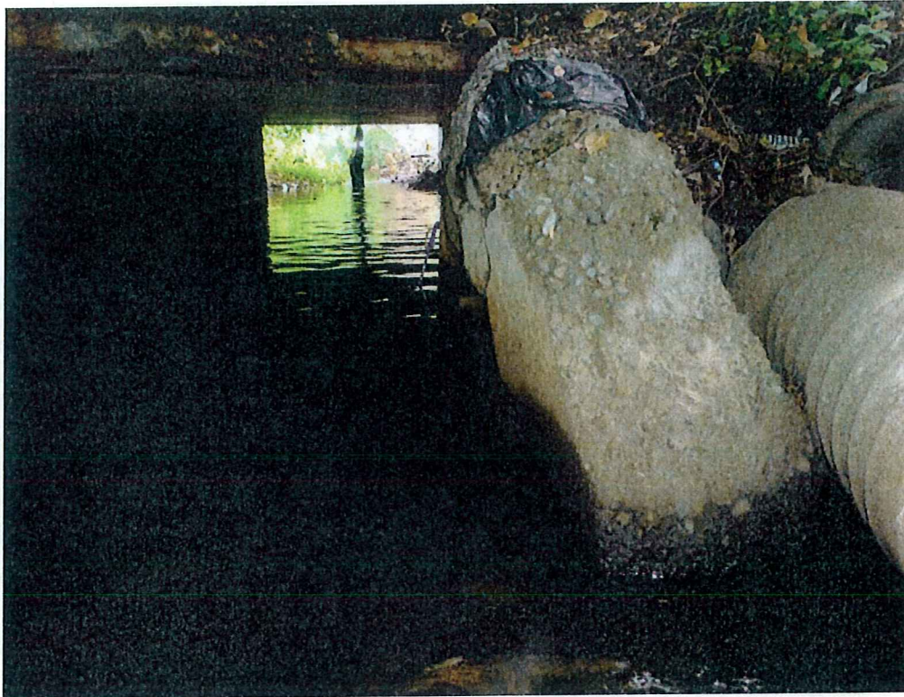
Photo 21: Southwest wingwall leaning in towards channel
