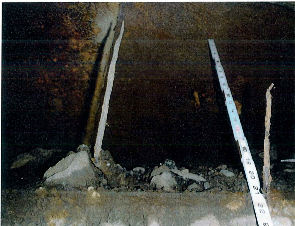
Photo 4: Hole in roof at the East end of the culvert measures 27" to the bottom of the steel street plates
