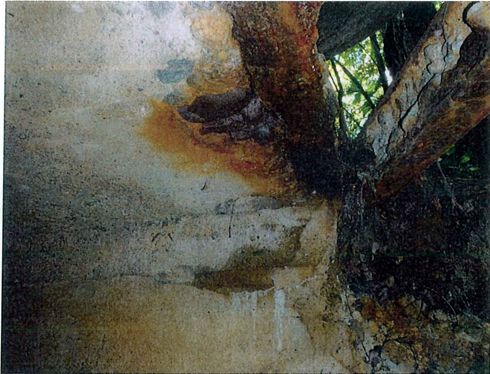
Photo 7: Southwest corner showing hole in roof and exposed and unsupported railroad rail
