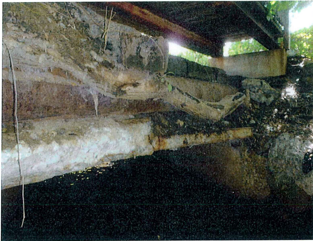
Photo 25: Tree root & 12" CI pipe along West end of roof
