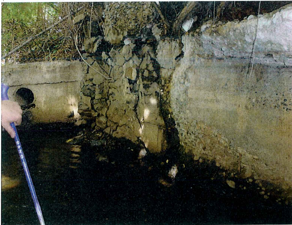
Photo 18: Northwest wingwall is crumbling and leaning in towards the channel
