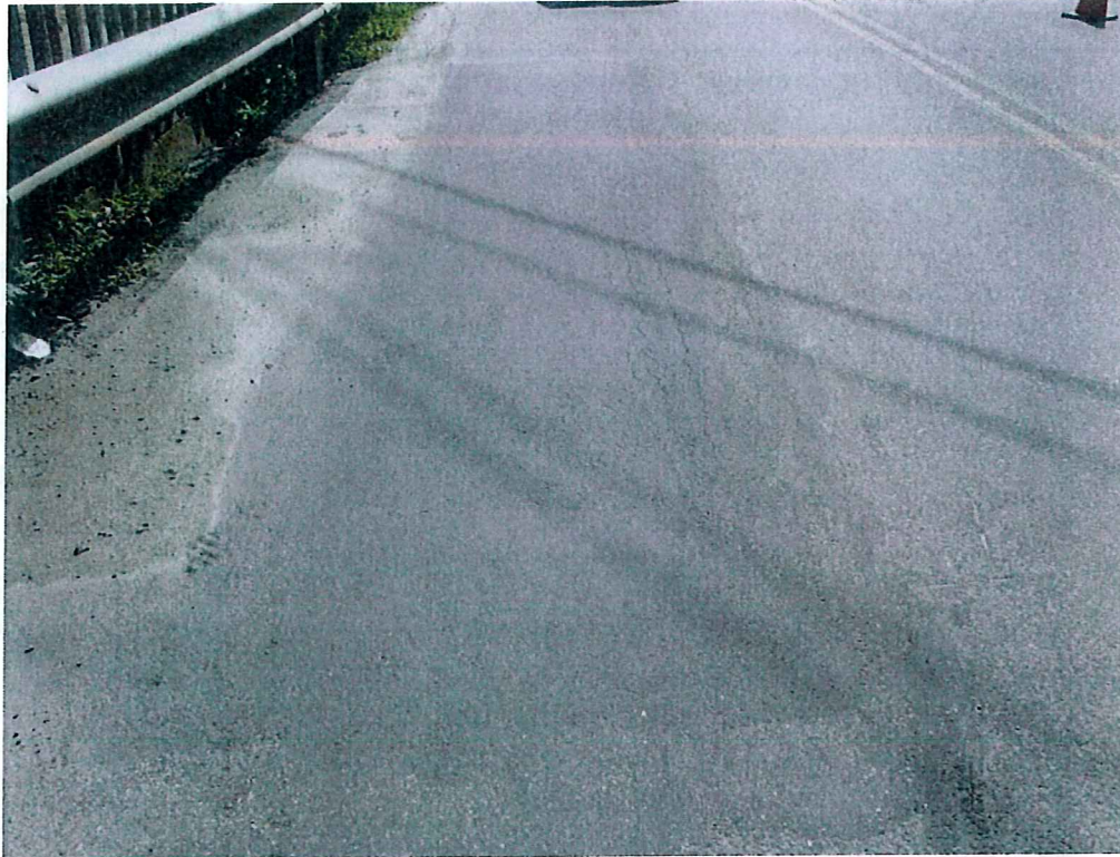
Photo 23: Longitudinal cracking are present in the asphalt patch over the steel road plates on the Northbound travel lane
