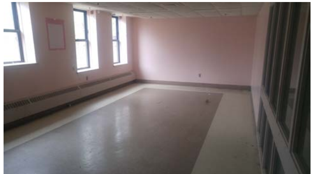
Building 46, suspect floor tile
