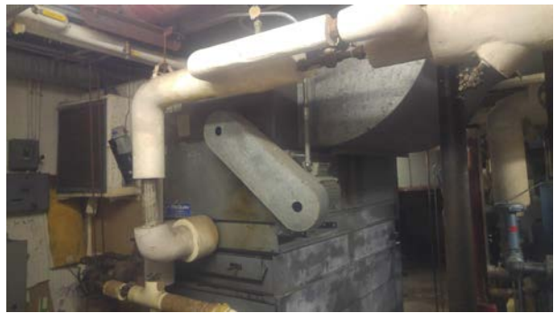
Building 37, mechanical room
