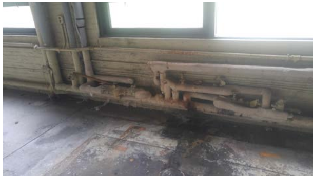
Building 22, pipe insulation
