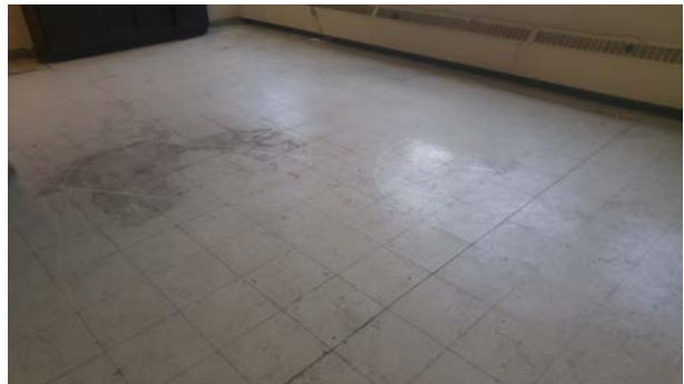
Building 22, suspect floor tile
