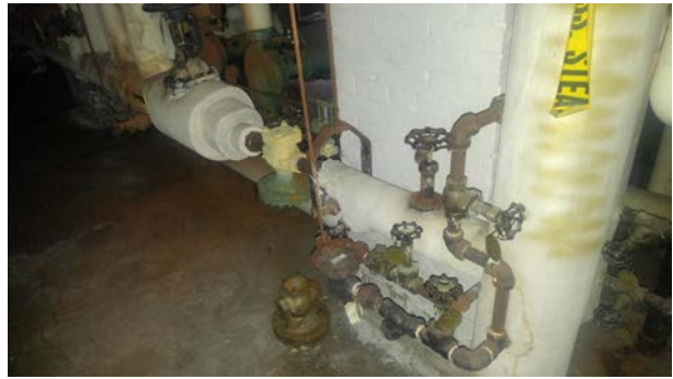
Building 36, mechanical room
