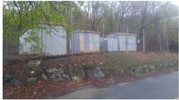
Building 122, electrical substation
