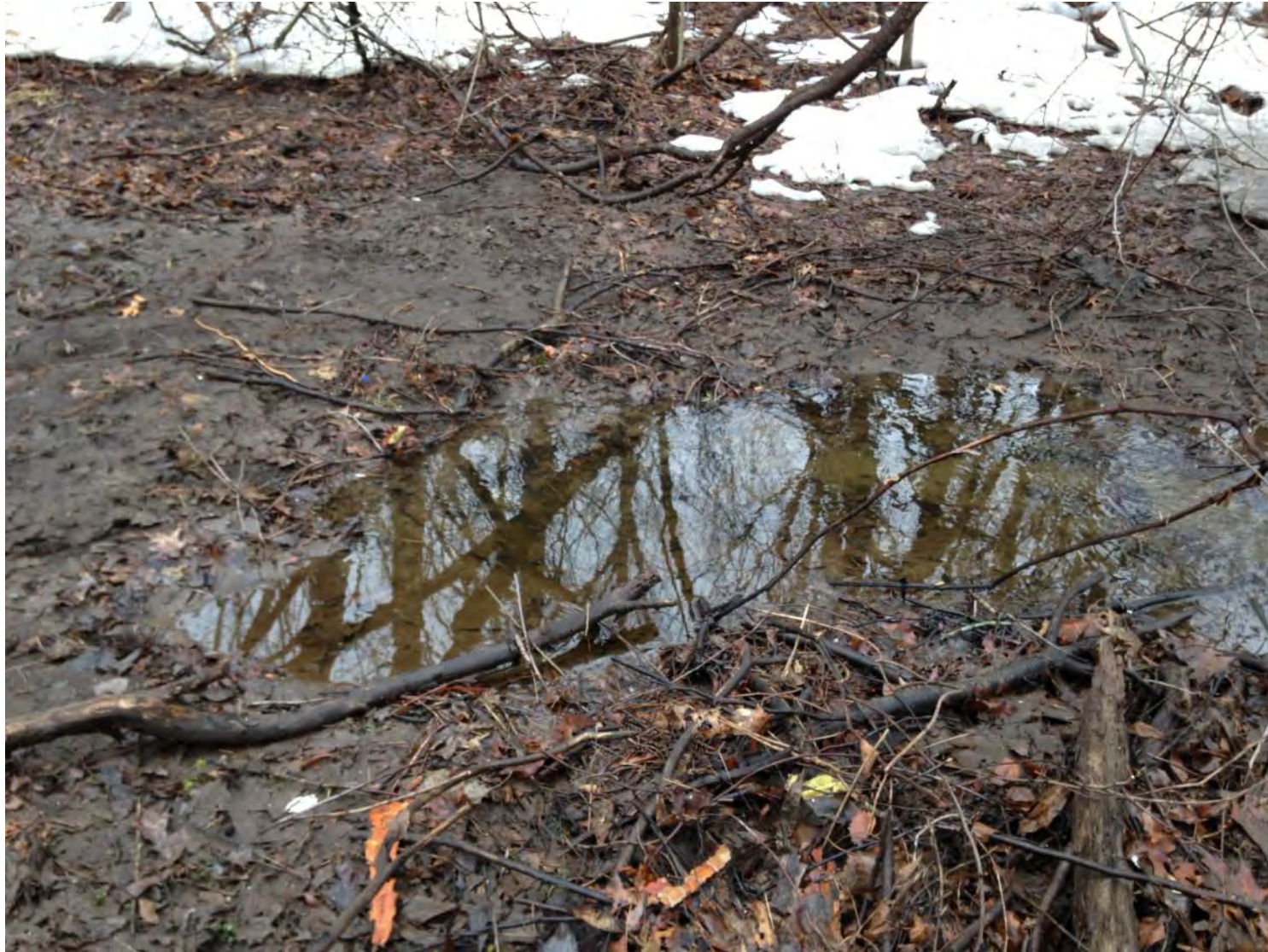
Photo 6 18-inch Inlet (covered in sediment) on National Archives Property
