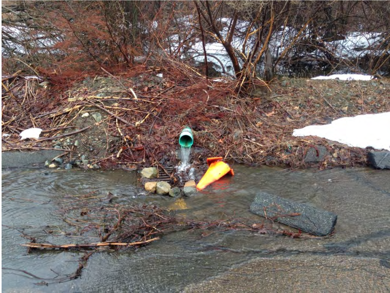
Photo 4 Recently Installed 4-inch Pipe by the State Discharging to Catch Basin
