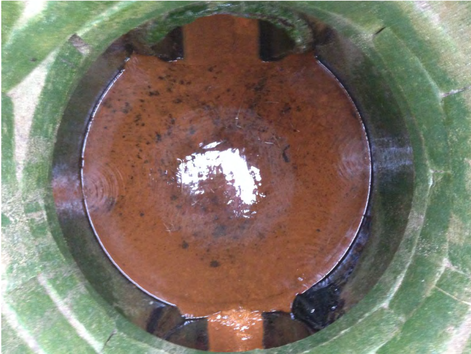
Photo 2 Catch Basin Over 21-inch Drain - Minimal Flow Through
