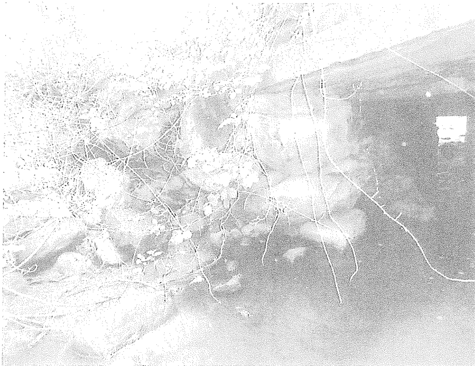
Photo 24: Southwest wingwall-Several displaced stones.
