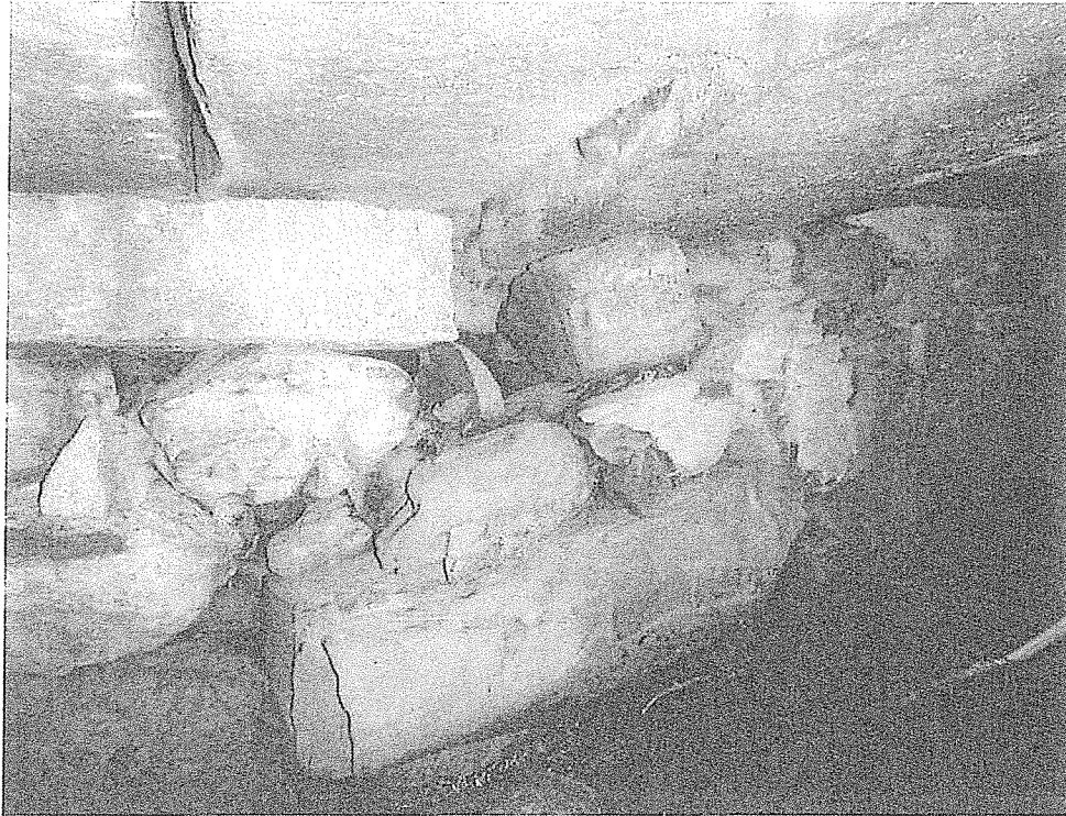
Photo 17: West breastwall-Void at the top measuring: 15" W x 21" H x 30" D.
