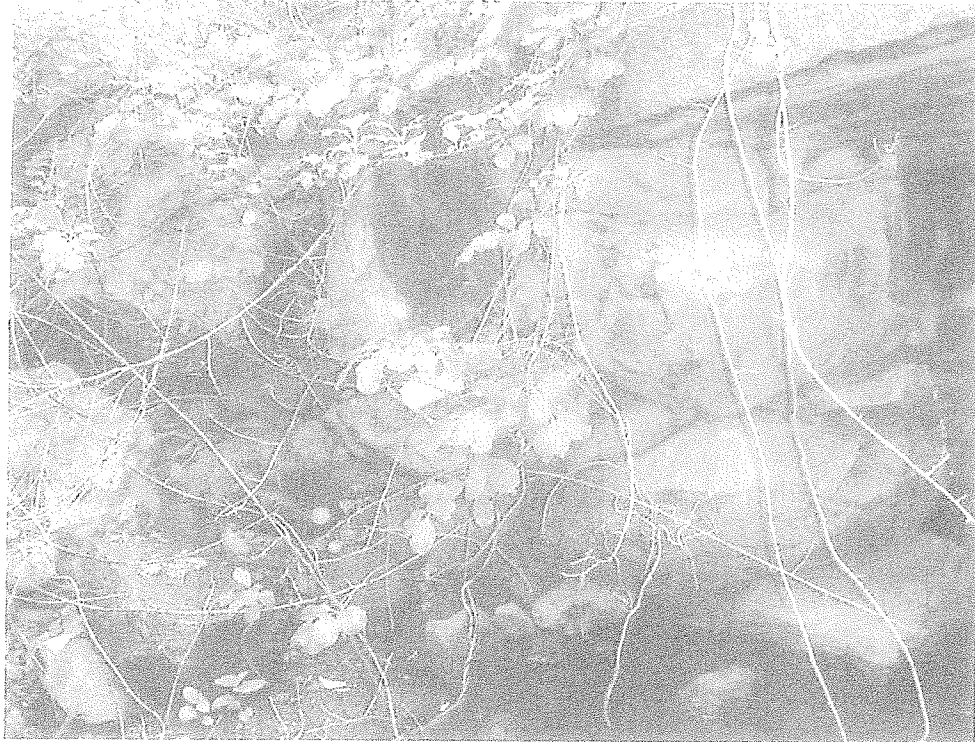
Photo 23: Southwest wingwall-Several displaced stones.
