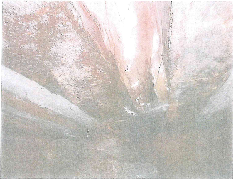
Photo 11: Typical condition of the bottom flanges of the steel I-Beams showing severe rust, lamination, and some section loss/ Wooden planks between beams.
