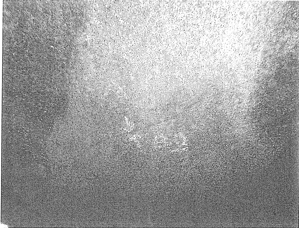
Photo 5: Slab 3-Hairline diagonal crack at mid-span.
