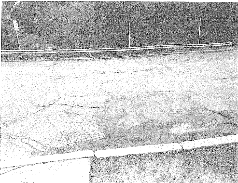
Photo 2: Typical wearing surface photo showing heavy cracking throughout.
