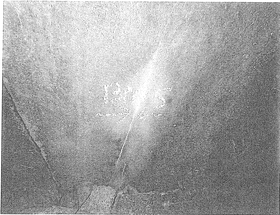
Photo 7: Slab 5-Longitudinal hairline crack at the east end measuring 2' long.
