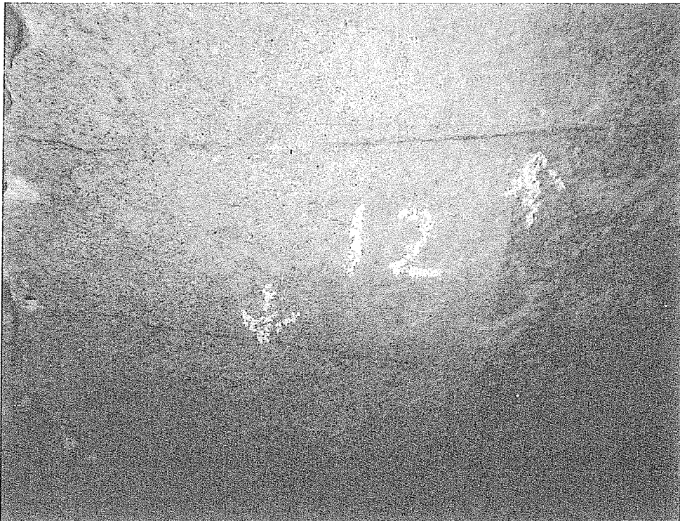
Photo 10: Slab 12-2 partial width hairline transverse cracks near midspan.
