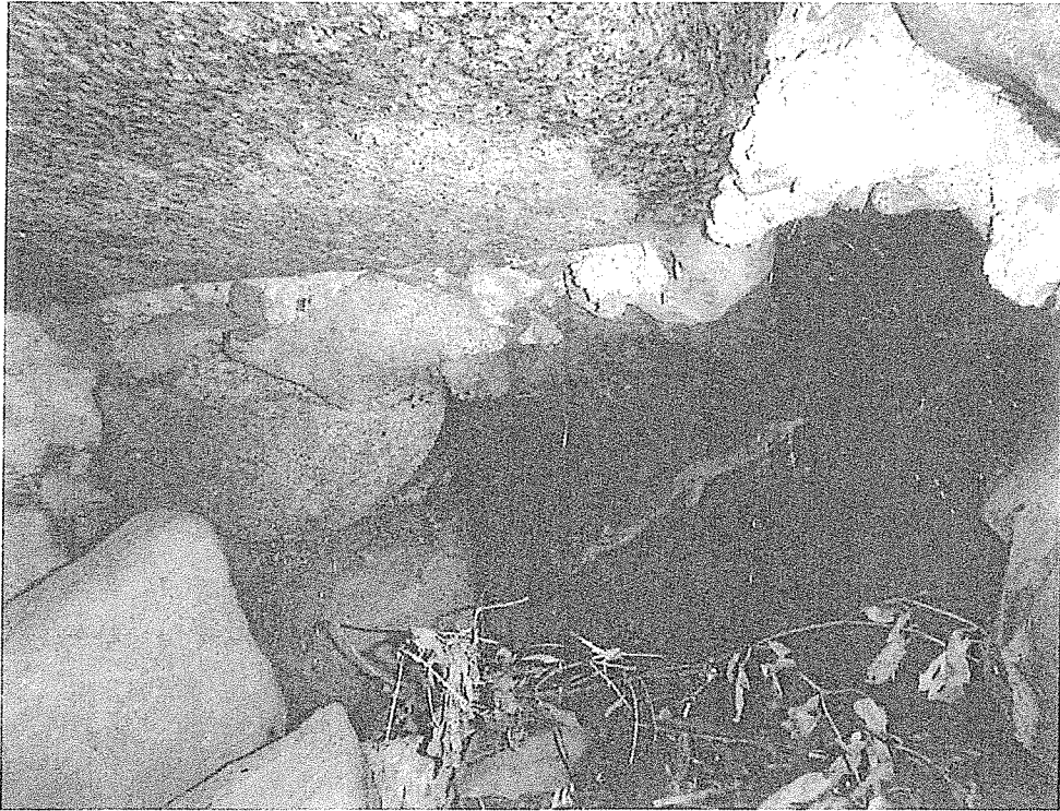
Photo 13: Slab 14-Complete loss of bearing area at the west breastwall.
