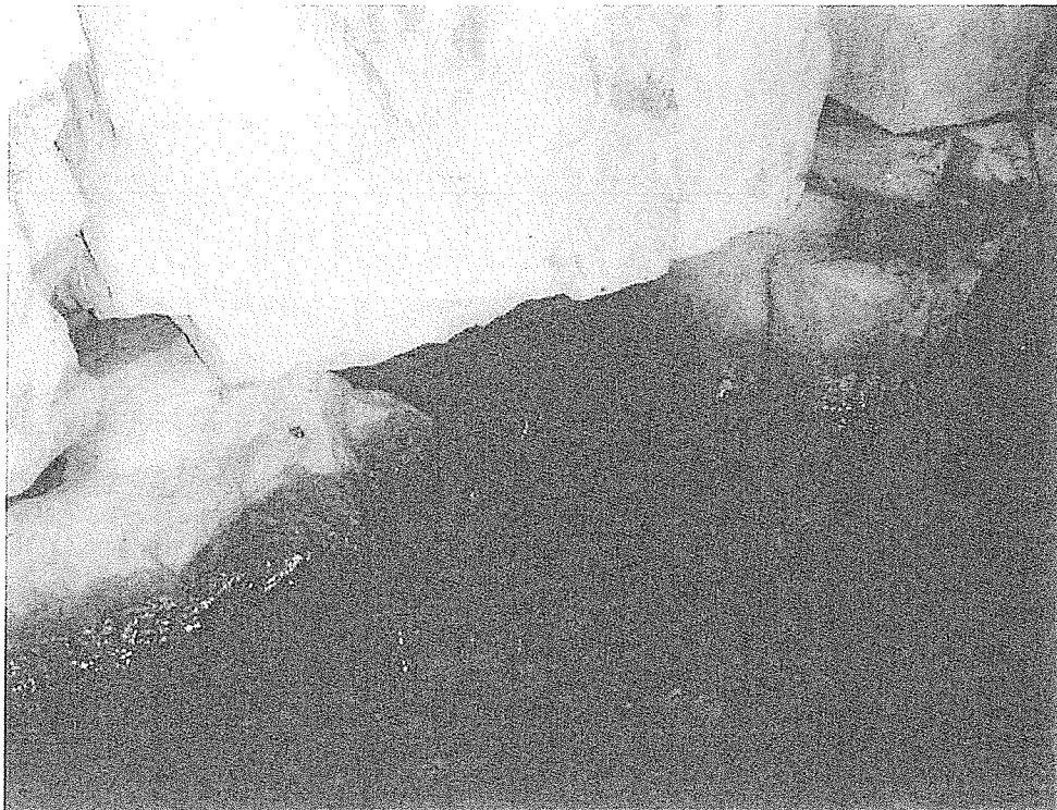
Photo 16: West breastwall-Void below the reinforced concrete slab measuring: 20" W x 15" H x 24" D.
