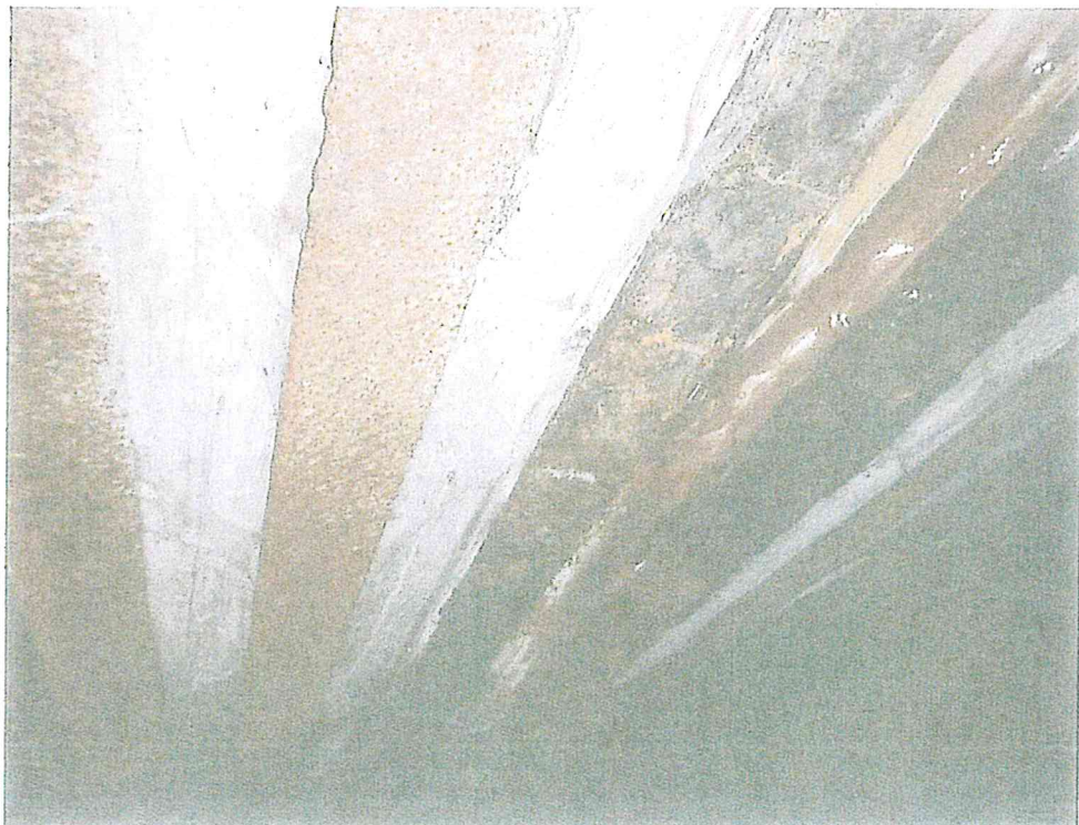
Photo 12: Typical condition of steel I-Beams showing severe rust on the bottom flanges of several beams with lamination. Note: webs are hidden due to wooden planks between.
