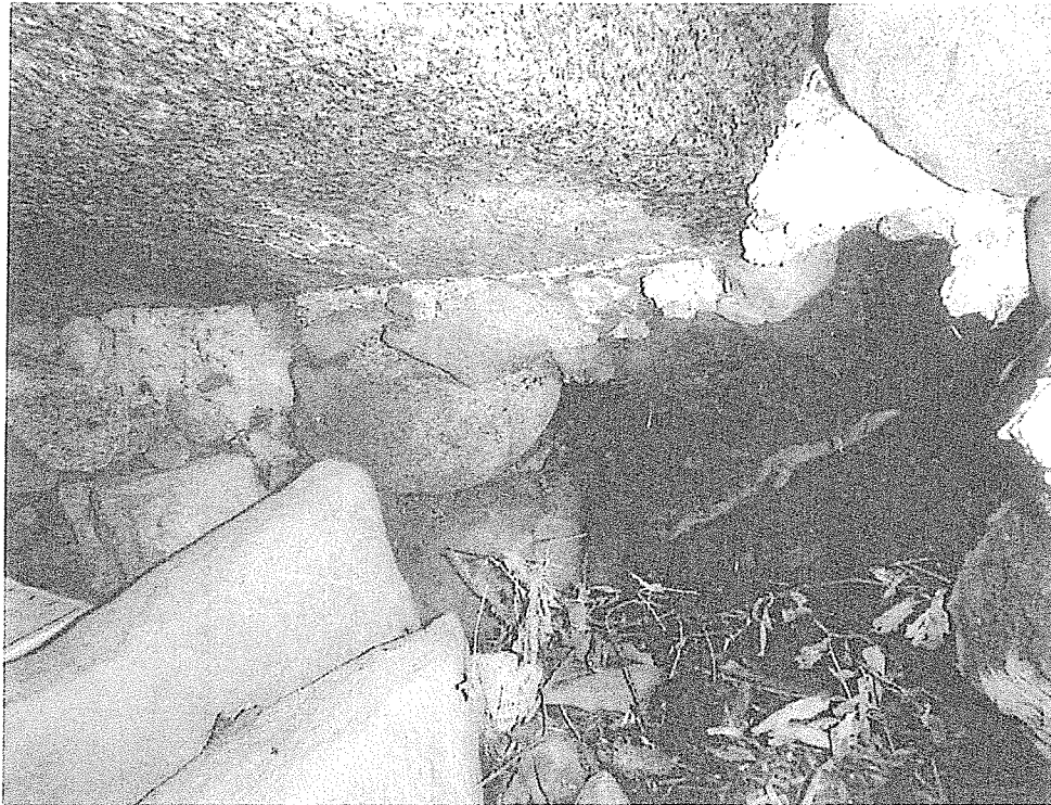
Photo 15: Slab 14-Complete loss of bearing area at the west breastwall.
