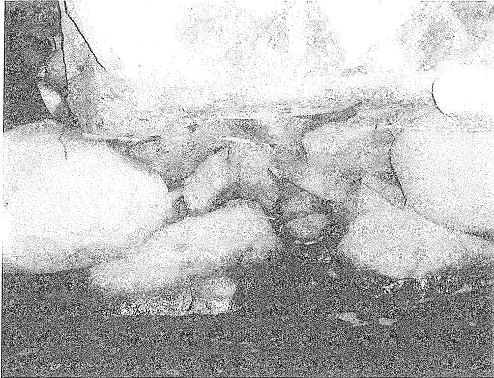
Photo 19: West breastwall, below beam 5-Void measuring: 27" W x 17" H x 14" D.
