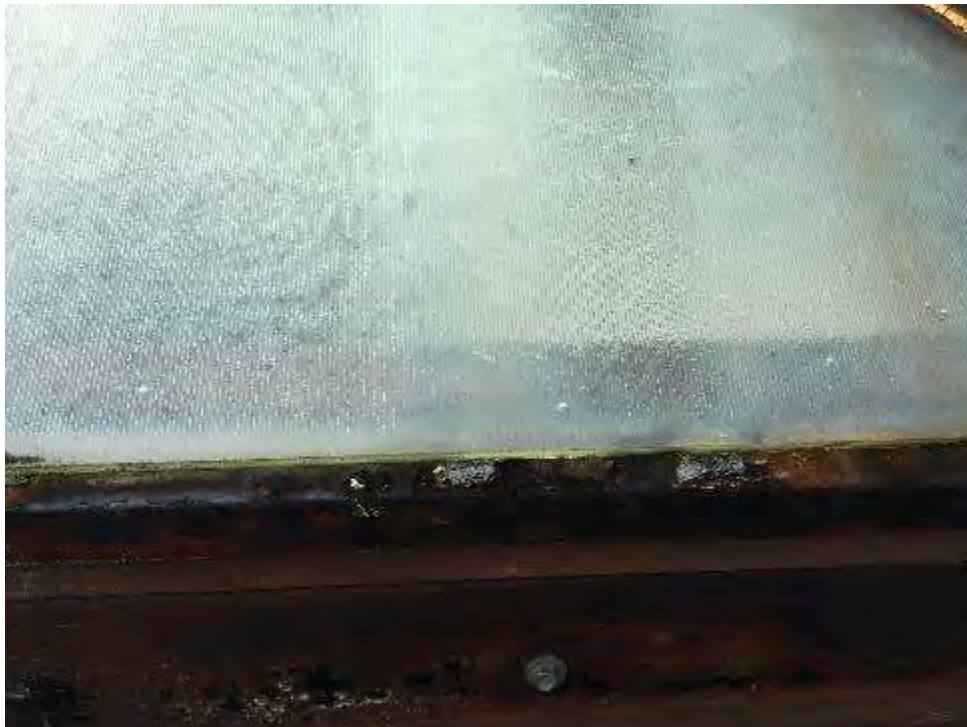
Roof Skylight Caulking
