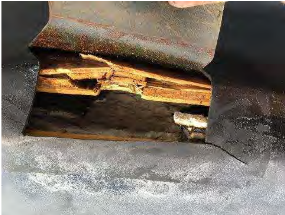
Black Mastic at Parapeet Behind Rubber and Plywood
