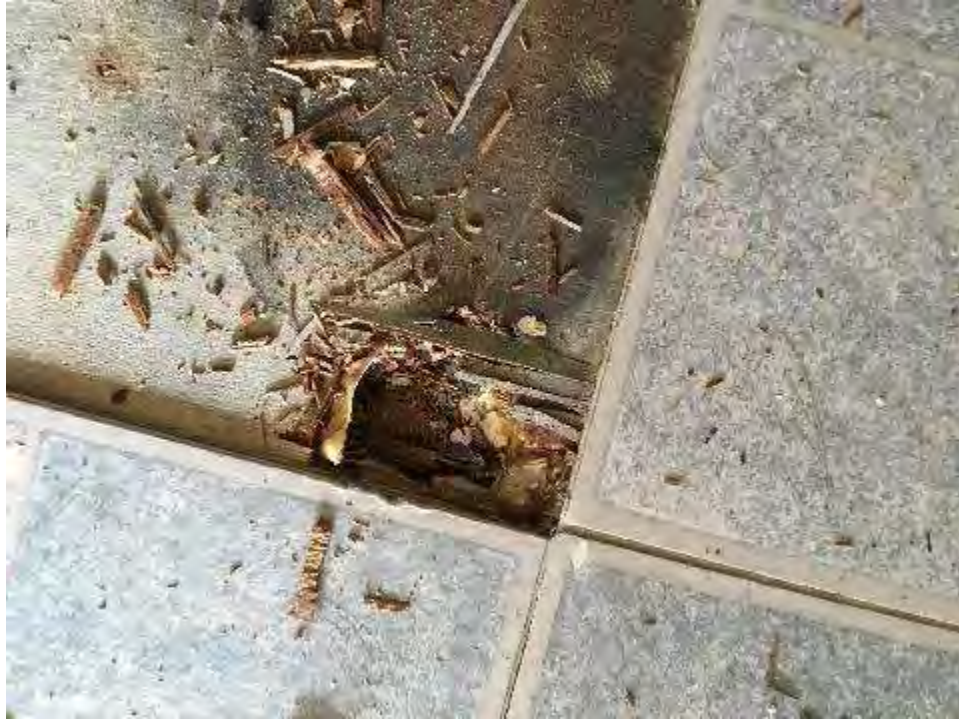
Yellow Pattern Linoleum Under Plywood, Orange Sheet Flooring and Red Paper and Associated Mastics
