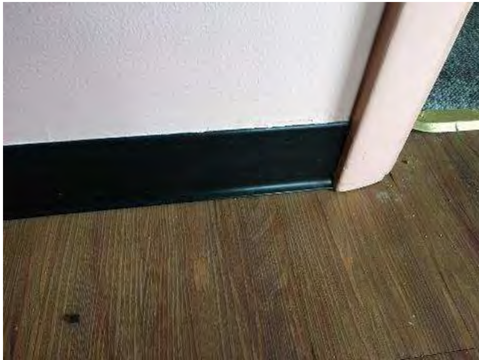
Faux Wood Floor Paneling, Black Cove Base and Associated Mastics
