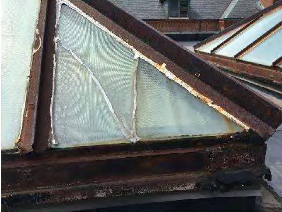
Roof Skylight Glazing
