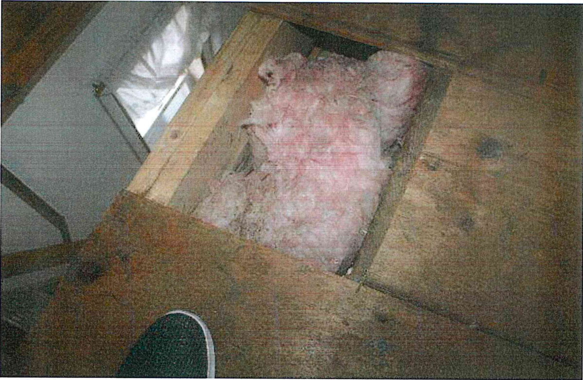
Figure 11: Fiberglass insulation in attic
