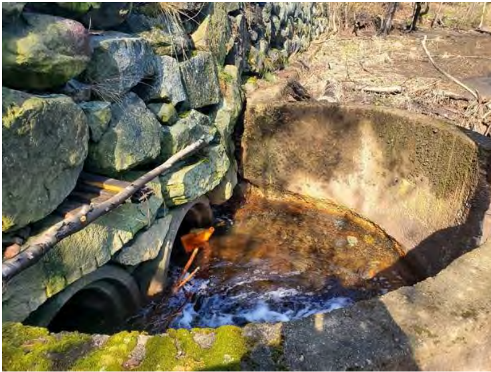
Photo 1: View of the outlet structure on the northern side of the entrance drive to the YMCA.
