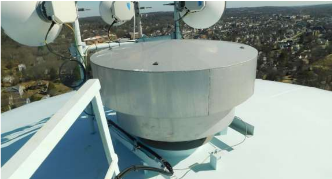
Photos show the existing roof vent, which appears to be in good condition
