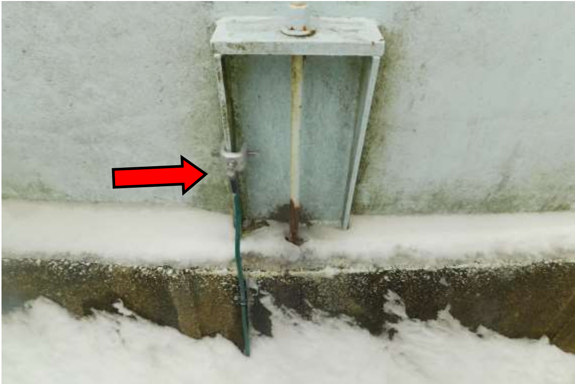
Photo shows the tank is electrically grounded for lightning protection as required by OSH Act of 1970 Section 5 and appears to be in good condition.
