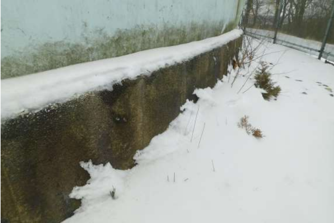
Photo shows the area around the tank foundation is properly graded and in compliance with AWWA D100-11; 12.7.1 Height aboveground.
