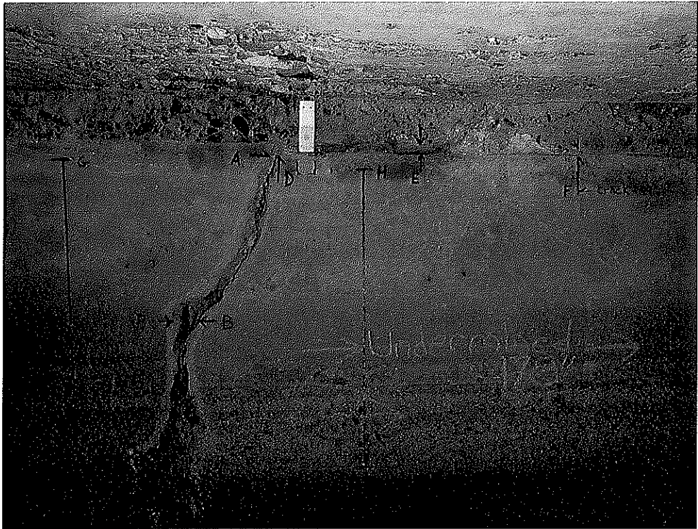
Photo 1: South wall, locations of measurements being taken at settlement cracks
