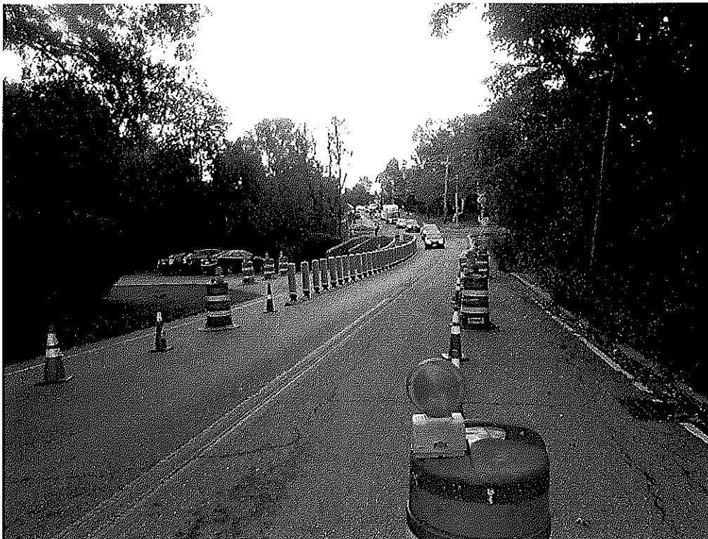
Photo 4: Traffic has been restricted to a single lane travelling Northbound over the center of the culvert
