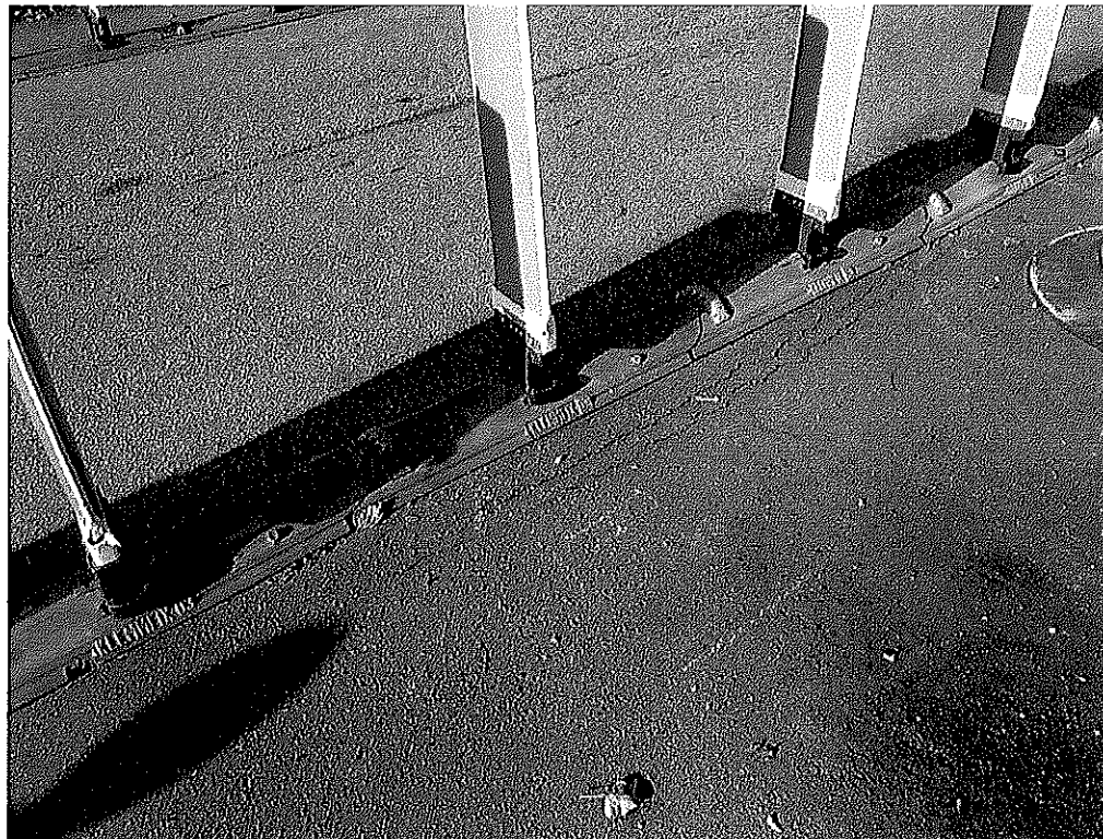
Photo 6: Cracks in pavement indicate the approximate limits of the steel plates present under the wearing surface
