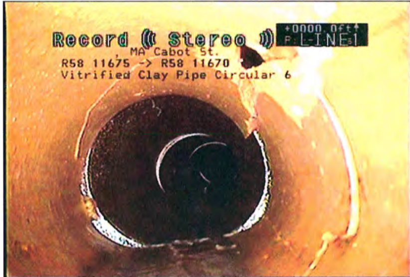
Photo: 56_57_270_A.jpg, VCR No.: Waltham TV #1 2.1FT, Fracture Multiple, from 10 to 06 o'clock, within 8 inches of joint: YES
