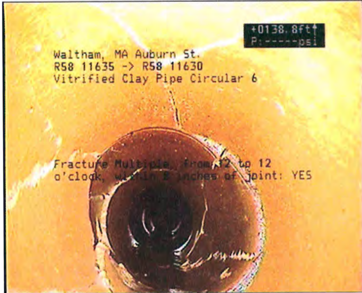
Photo: 1_1_9_A.JPG, VCR No.: Waltham TV #1 138.8FT, Fracture Multiple, from 12 to 12 o'clock, within 8 inches of joint: YES
