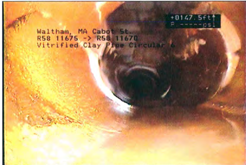
Photo: 56_57_280_A.jpg, VCR No.: Waltham TV #1 147.5FT, Fracture Multiple, from 12 to 12 o'clock, within 8 inches of joint: YES
