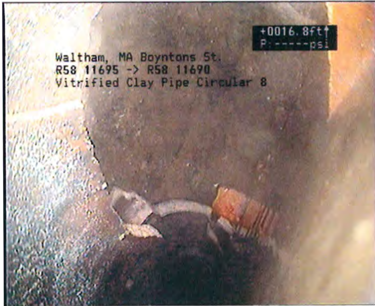
Photo: 35_36_187_A.JPG, VCR No.: Waltham TV #1 16.8FT, Hole Void Visible, from 12 to 06 o'clock, within 8 inches of joint: YES
