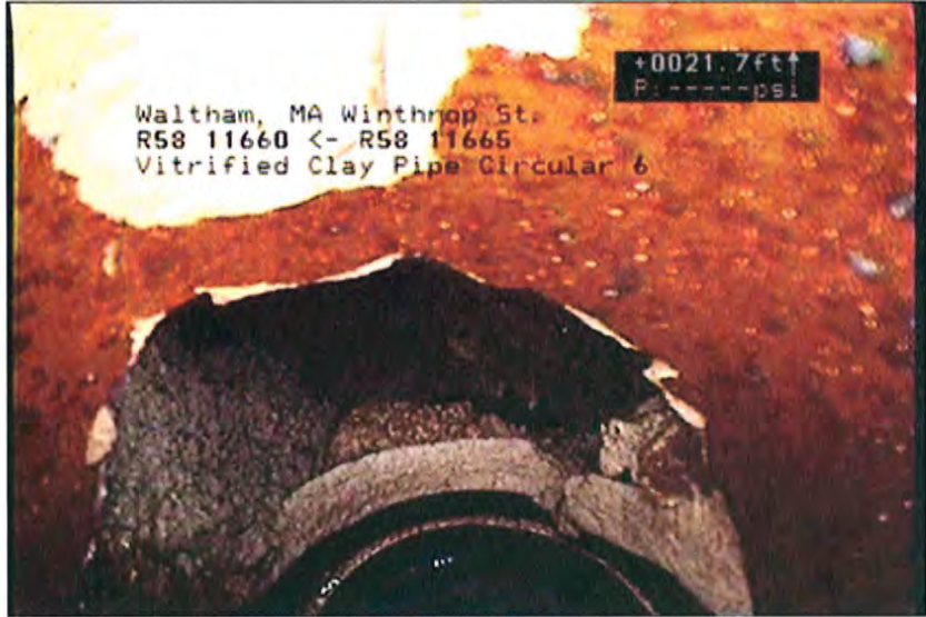
Photo: 52_53_254_A.jpg, VCR No.: Waltham TV #1 22.5FT, Hole, from 09 to 11 o'clock, within 8 inches of joint: YES
