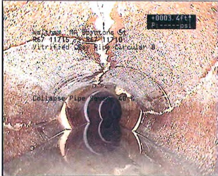
Photo: 36_37_190_A.JPG, VCR No.: Waltham TV #1 3.4FT, Collapse Pipe Sewer, 40 %
