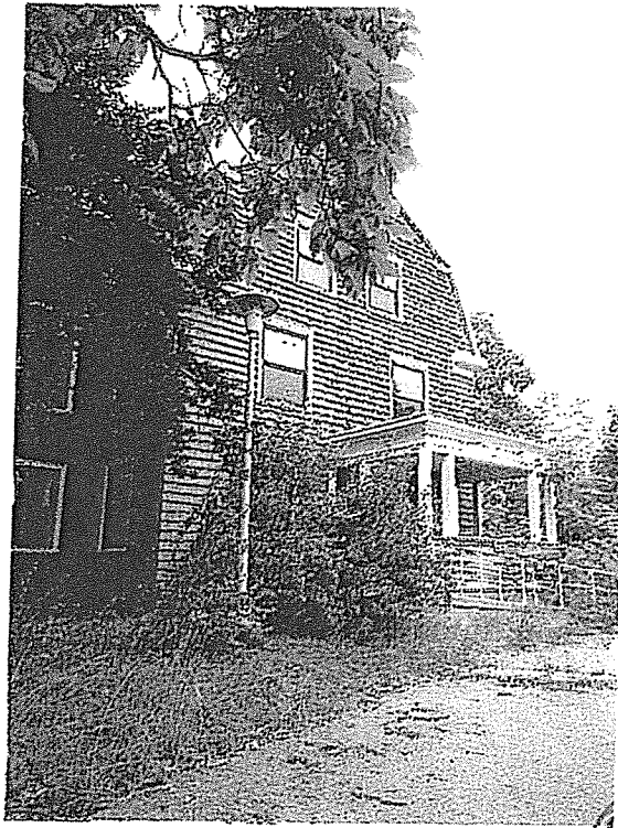
137. View West of East Elevation of Hillside Cottage Walter E. Fernald Developmental Center Waltham, MA
