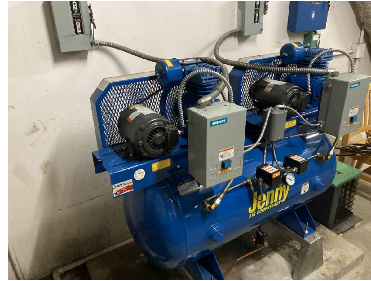
PHOTOGRAPH NO. 3 EXISTING AIR COMPRESSOR FOR PNEUMATIC CONTROLS TO BE REMOVED.
