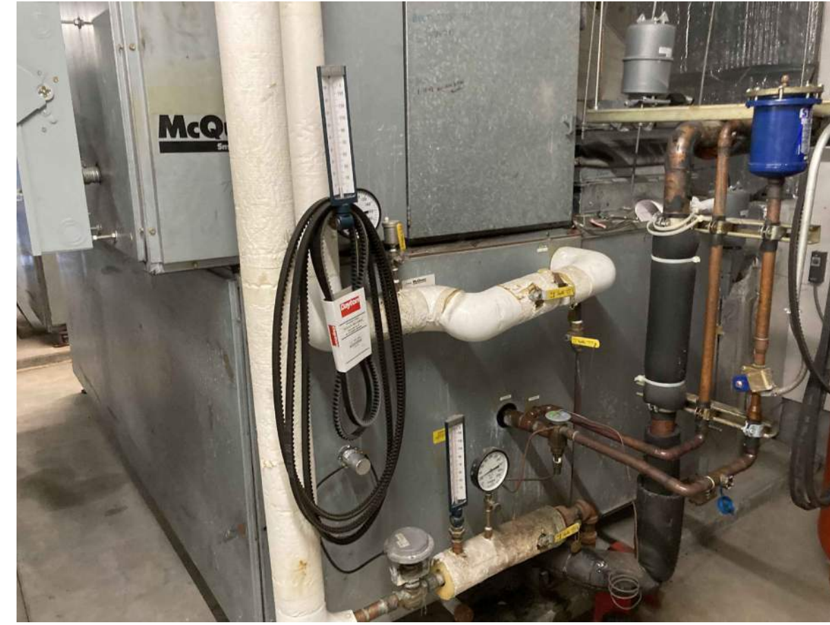
PHOTOGRAPH NO. 2 EXISTING AIR HANDLER IN MECHANICAL MEZZANINE TO BE REMOVED.
