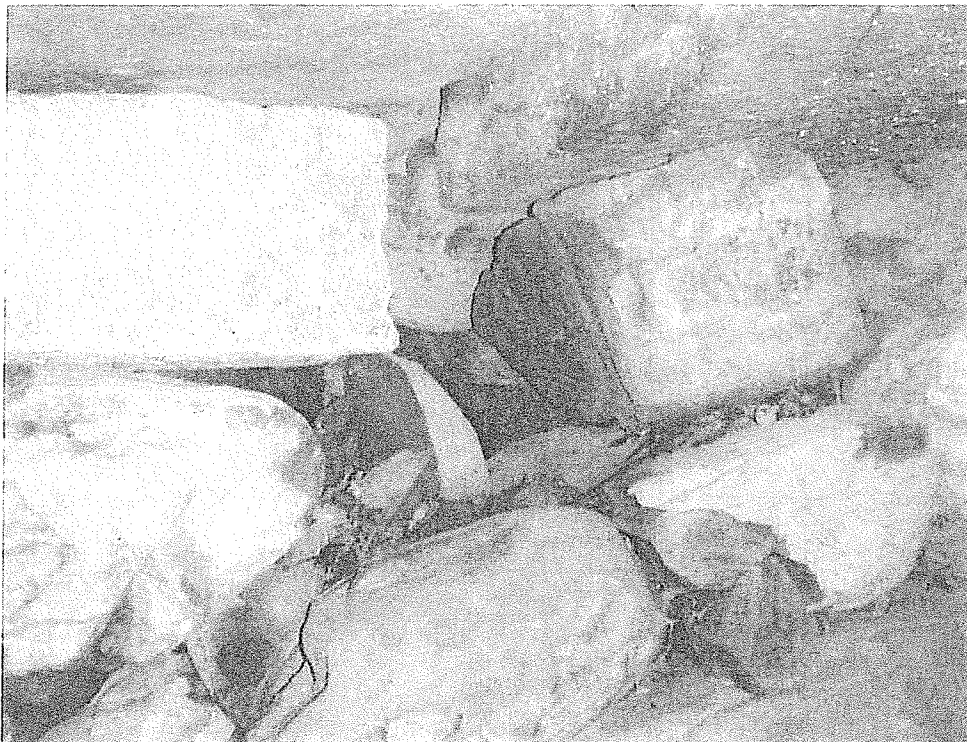
Photo 18: West breastwall-Void at the top measuring: 15" W x 21" H x 30" D.
