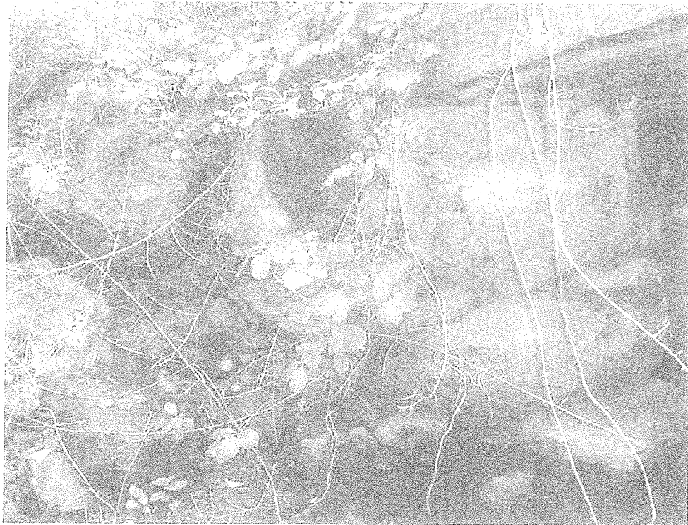
Photo 23: Southwest wingwall-Several displaced stones.
