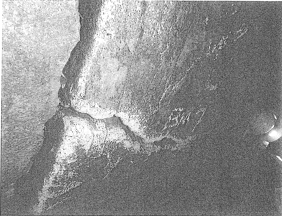
Photo 3: Slab 7-Full width transverse crack ranging from 3/4" to 2" wide.
