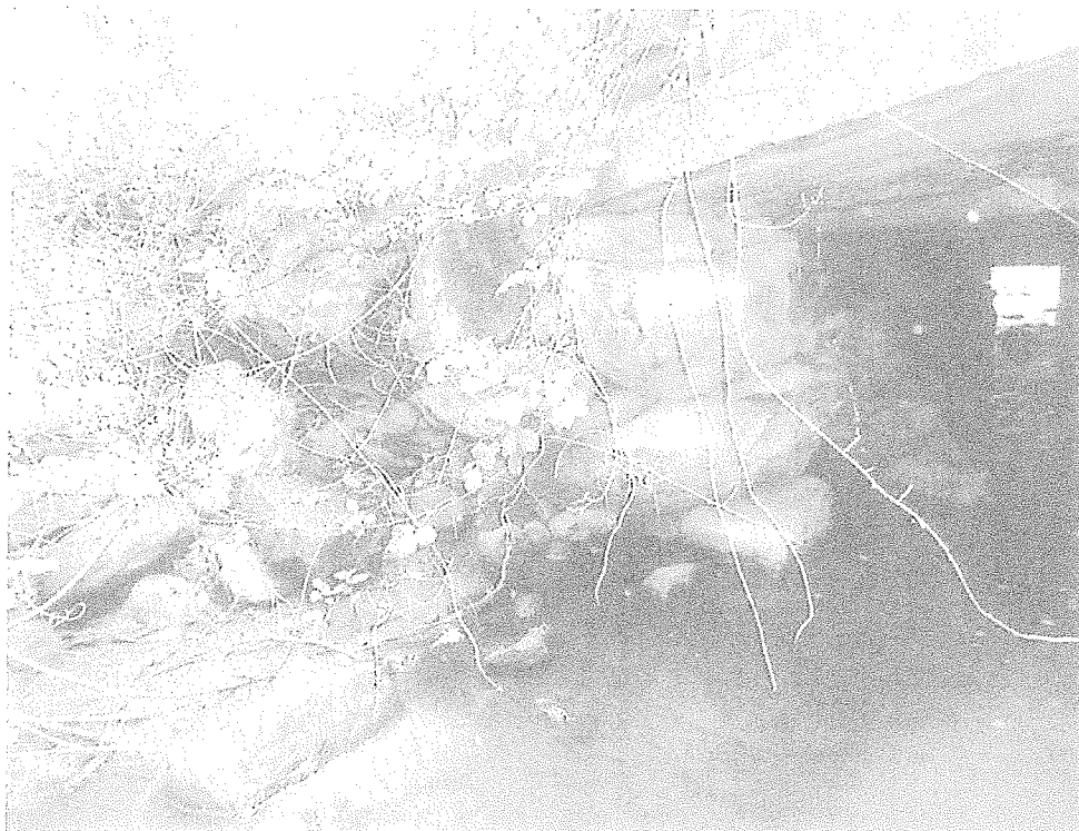
Photo 24: Southwest wingwall-Several displaced stones.
