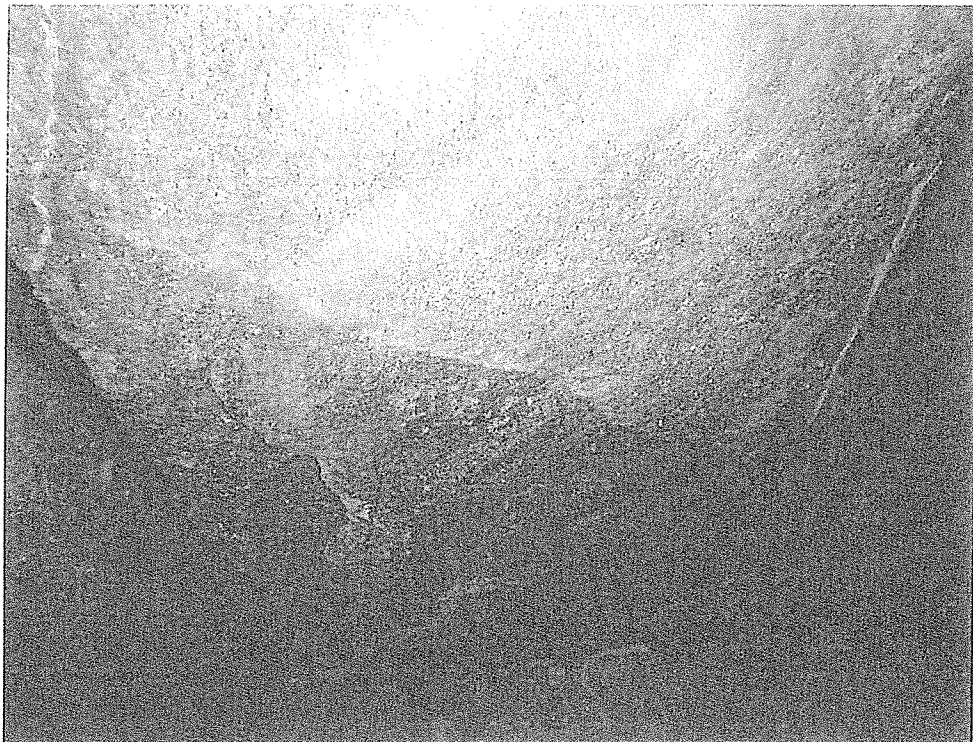
Photo 6: Slab 4-Hairline diagonal crack at midspan.
