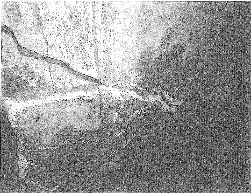
Photo 4: Slab 7-Full width crack ranging from 3/4" to 2".
