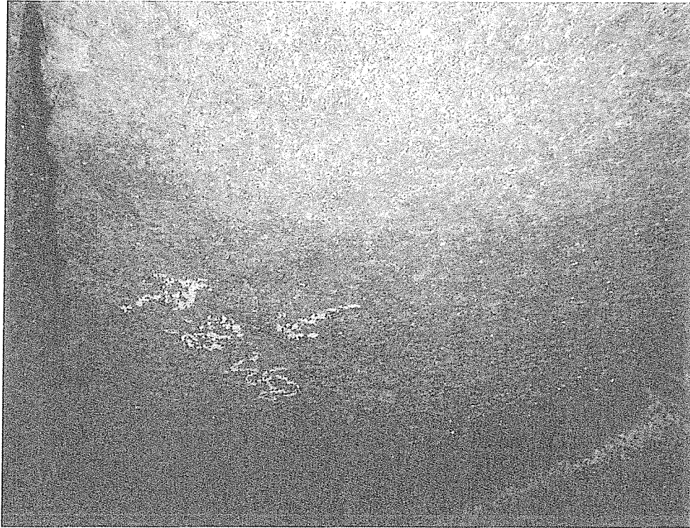
Photo 9: Slab 8-Full width partial transverse crack near mid-span.
