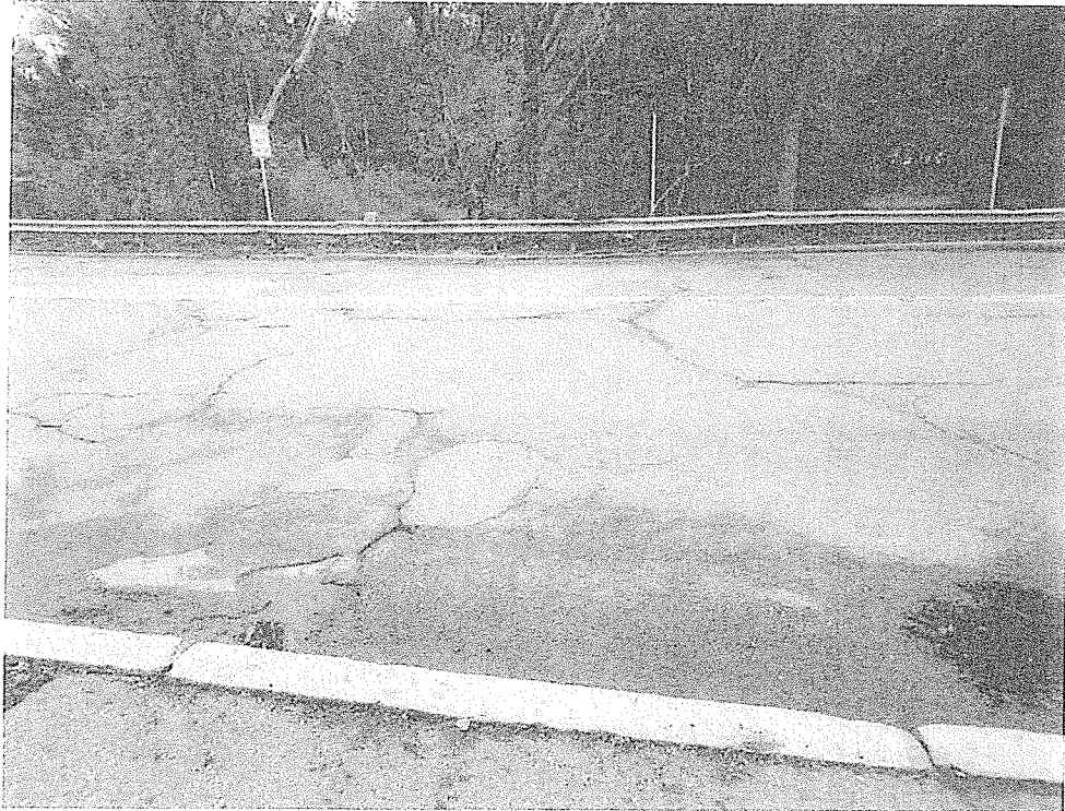
Photo 1: Typical wearing surface photo showing heavy cracking throughout.
