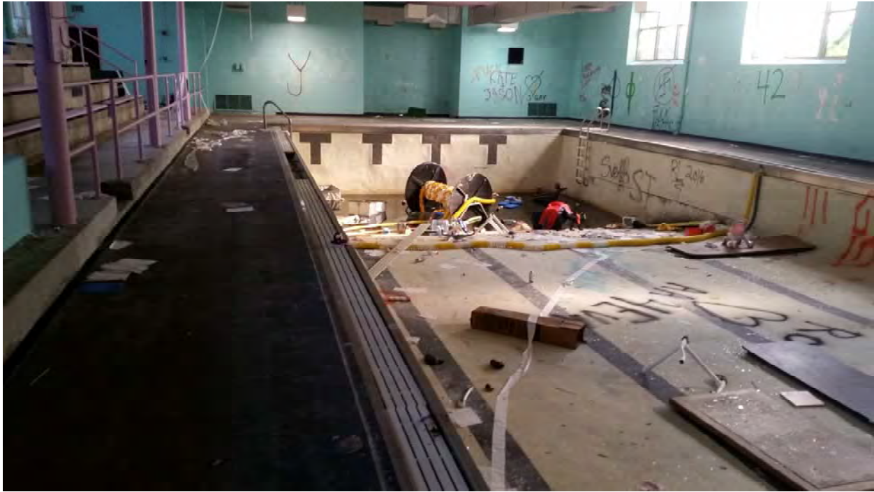
Pool area. Note pool liner, rubber tile mastic, textured paint, and black cove base and associated adhesive.
