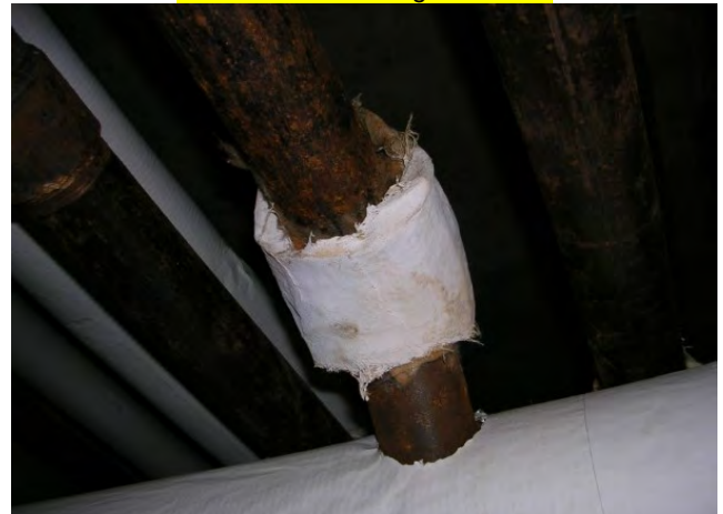
HA 03 Large Pipe Fitting on Fiberglass
