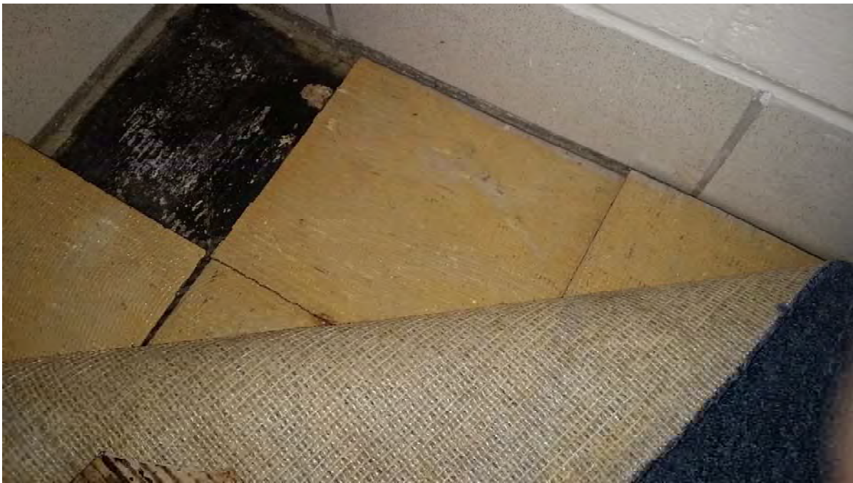
ACM 9"x9" grey streak floor tile and associated ACM mastic
