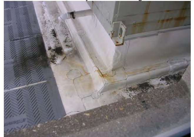
HA 92 White Caulking on PVC Roof
