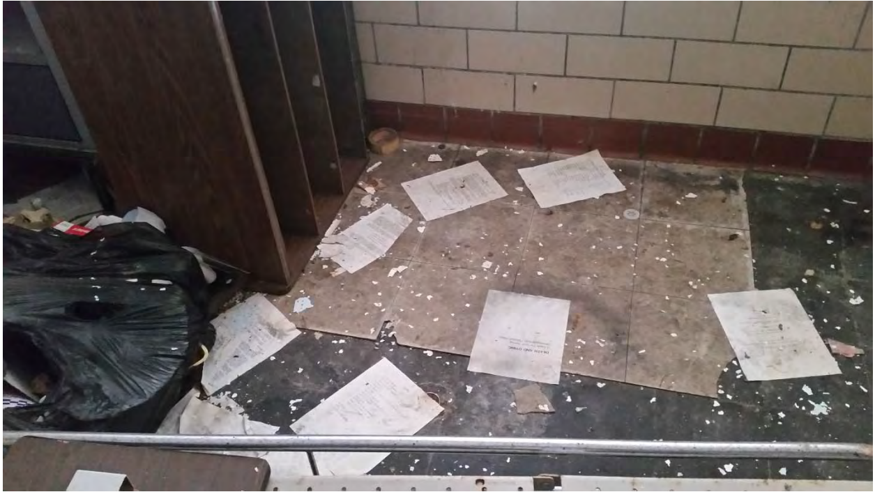
12"x12" white mottled floor tile, residual black mastic, and glazed block grout
