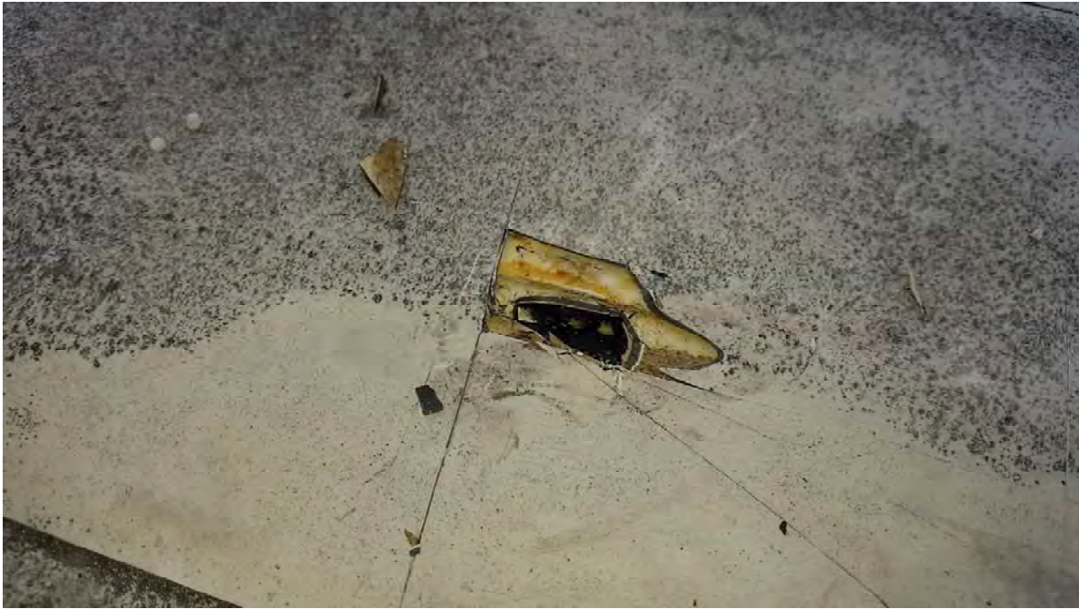
Black tar on roof flashing
