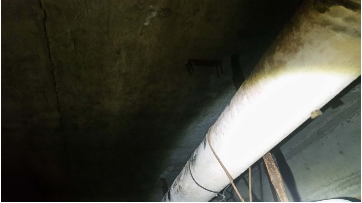
ACM pipe insulation
