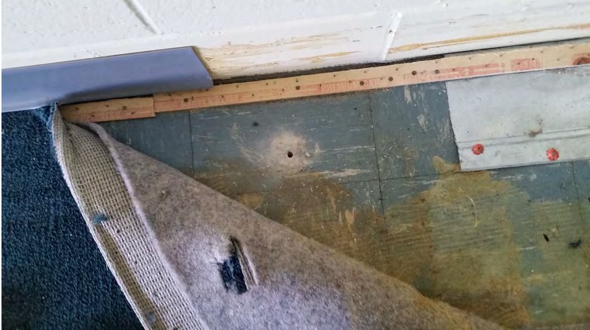
ACM 9"x9" blue streak floor tile and associated ACM mastic
