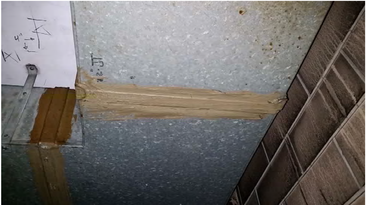
Yellow duct sealant
