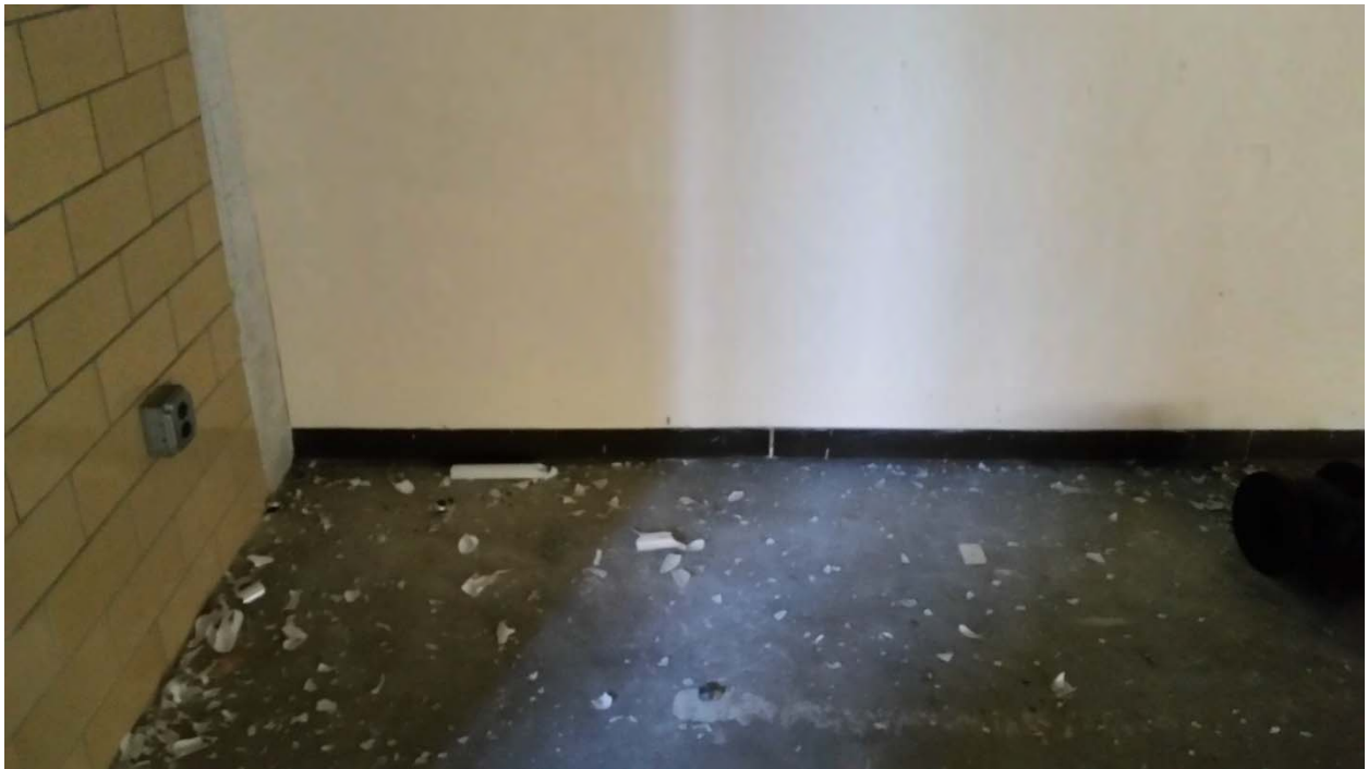
Plaster walls, glazed block walls, and black cove base and associated adhesive
