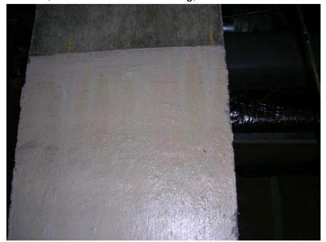
HA 69 Textured Paint on Concrete
