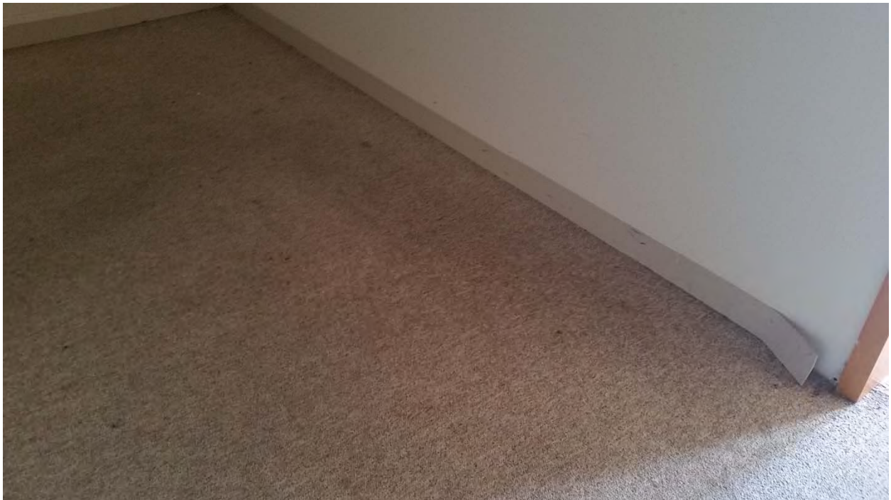
Beige cove base and associated mastic
