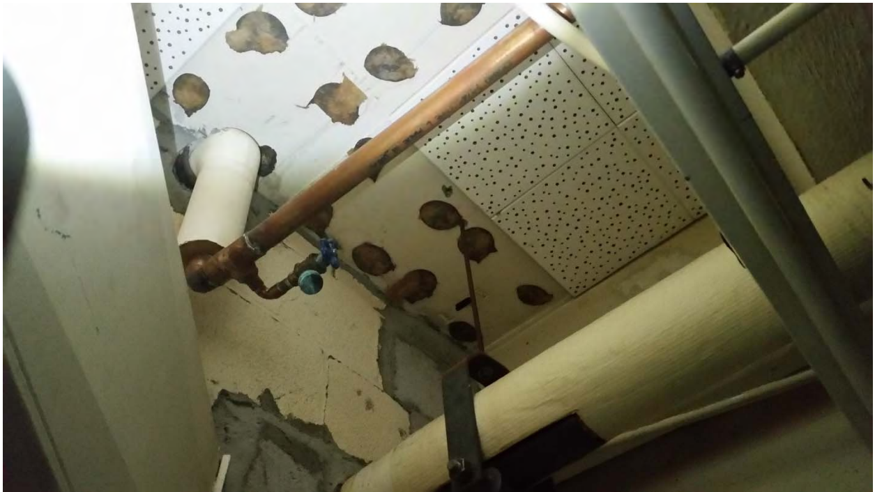
Brown glue daubs associated with 1'x1' fiberglass pinhole spline ceiling tiles
