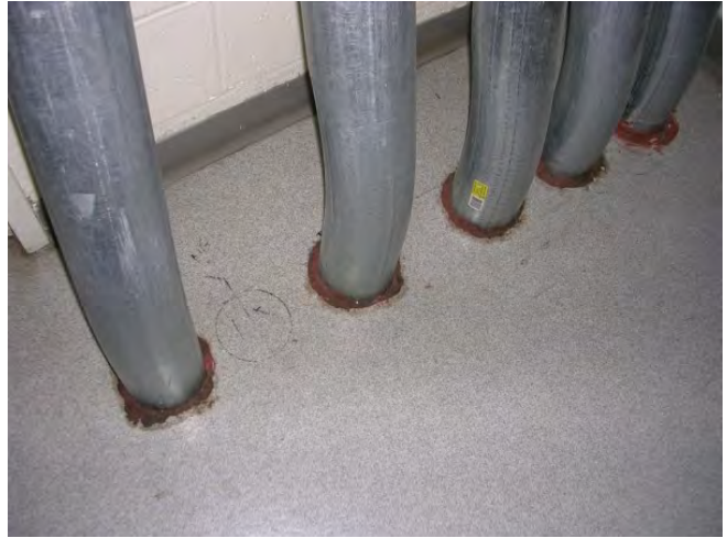
HA 47 Red Sealant on Electrical Conduit
