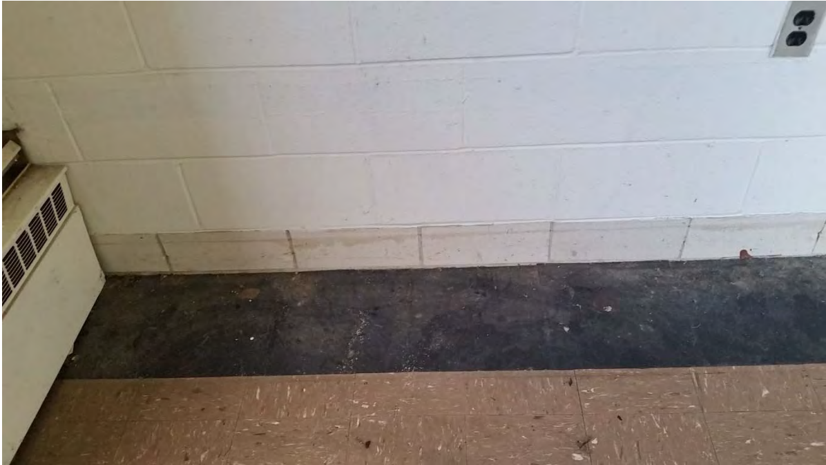
ACM 9"x9" brown floor tile and associated mastic; non-ACM 12"x12" black floor tile and associated non-ACM black mastic
