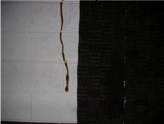
HA 74 Mastic on Wall
