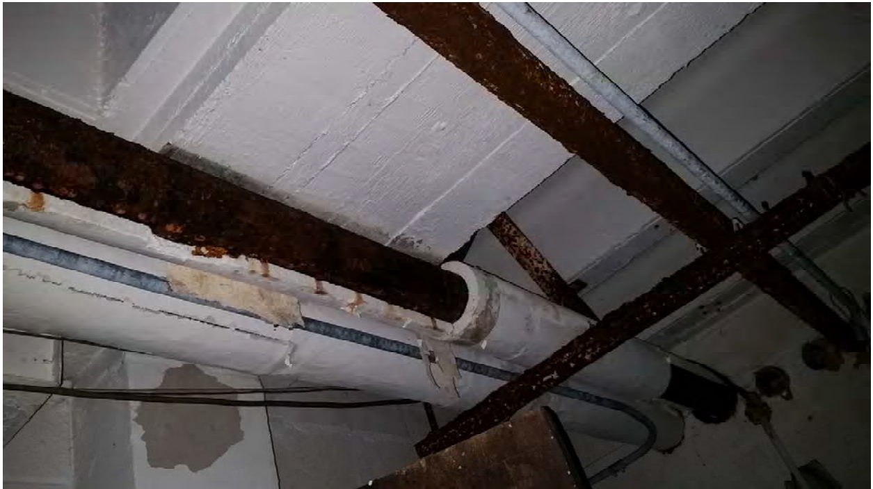
ACM white skim coat on concrete ceiling and ACM pipe insulation
