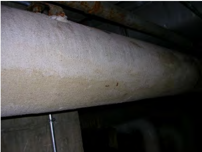
HA 76 Generator Exhaust Insulation
