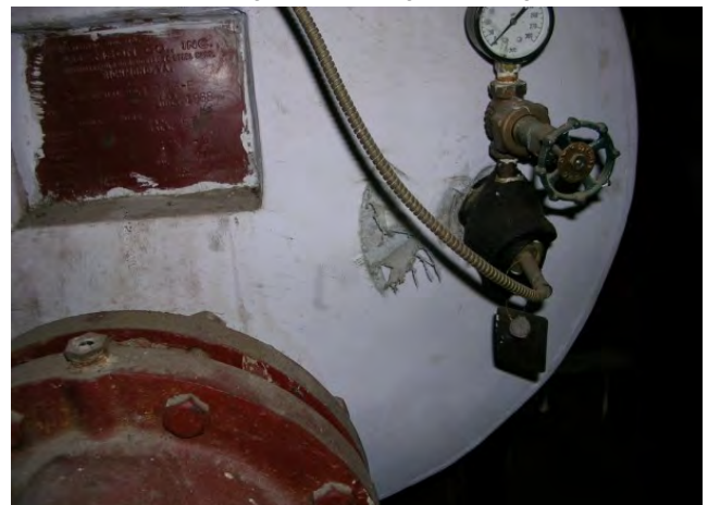
HA 01 Tank Insulation
