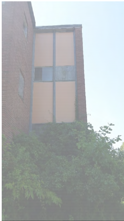
Exterior grey stairwell panel caulk
