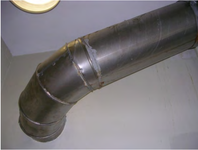
HA 26 Gray Sealant on Metal Fume Hood Exhaust
