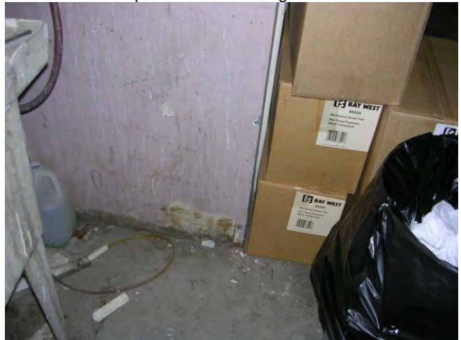
HA's 77,78 Sheetrock and Joint Compound
