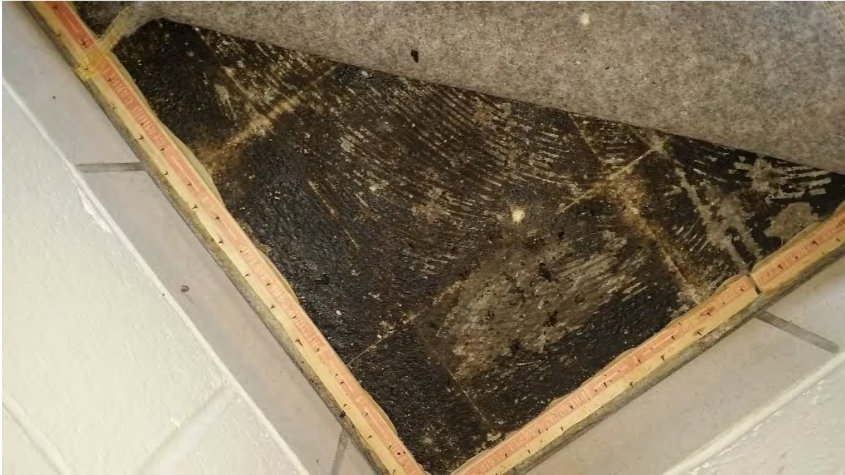
ACM residual black mastic (under carpet)
