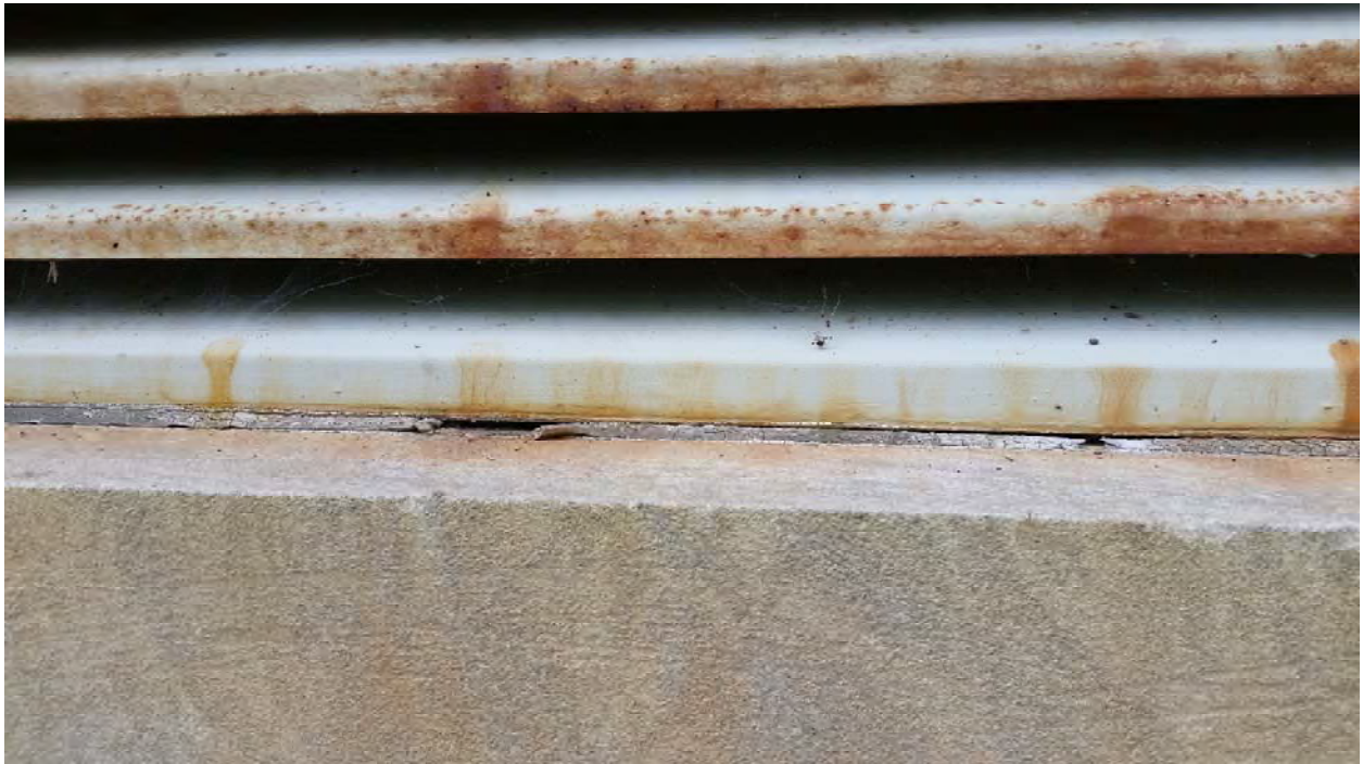
Non ACM beige vent caulk (top layer) and ACM brown vent caulk (bottom layer)
