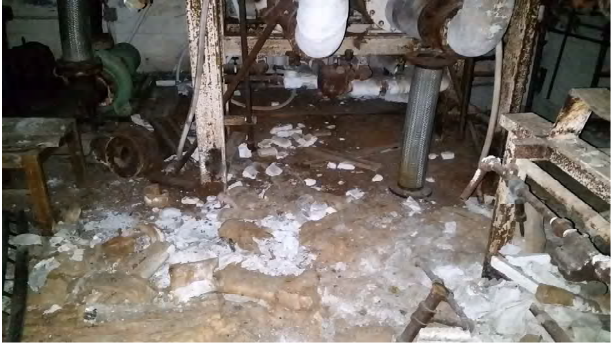
ACM pipe insulation and associated debris
