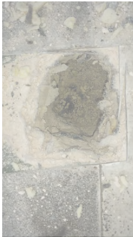
Pink fiberboard over Styrofoam, and black tar on roof deck (at depth)
