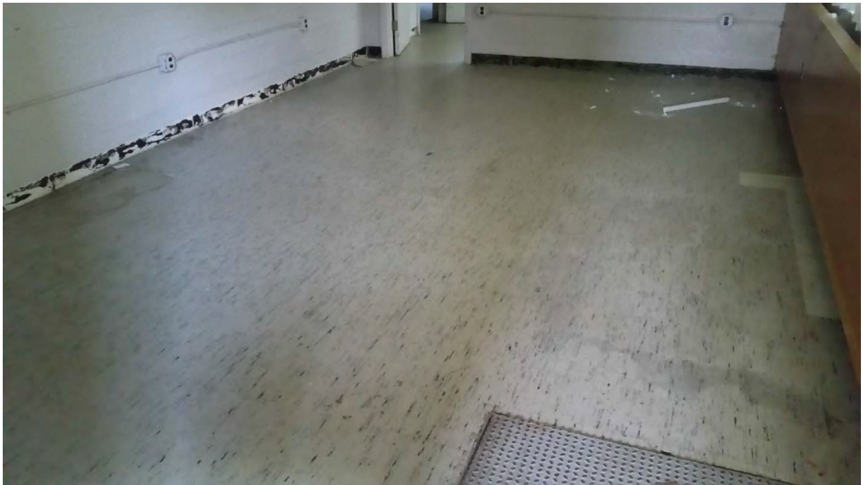
ACM 9"x9" beige with black streak floor tile and associated ACM black mastic.
