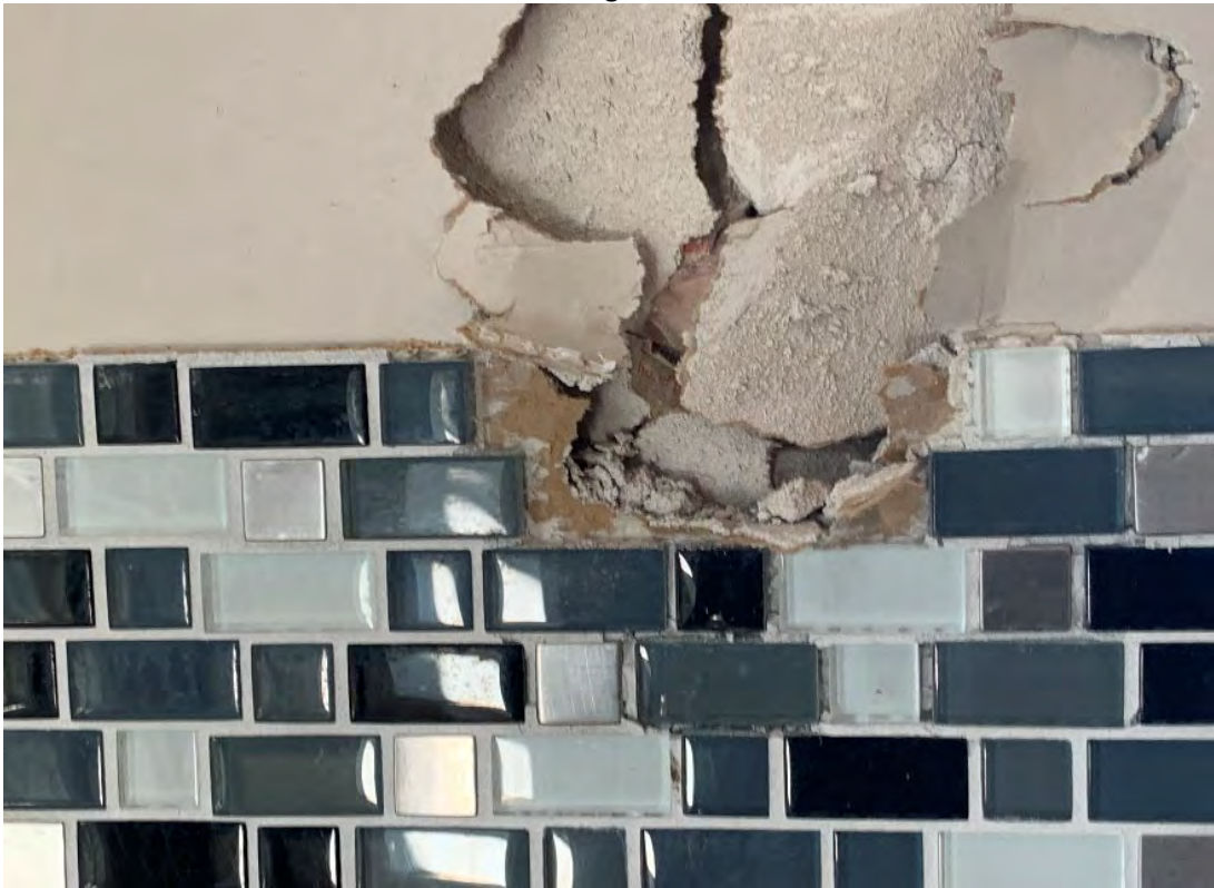
Kitchen ceramic wall tile on gypsum board
