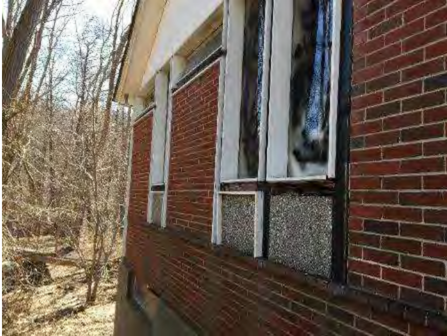
Exterior window system. Note ACM white window glaze, ACM residual grey window caulk, and ACM cement backing panel behind decorative cutouts (below windows)
