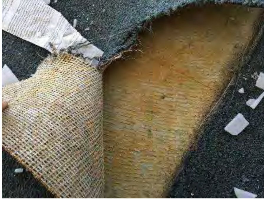
Yellow carpet mastic, and ACM 9"x9" grey with colored streak floor tile/mastic (under carpet)
