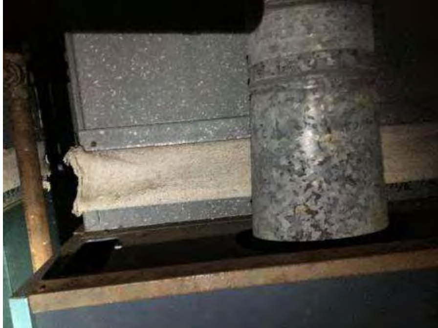
ACM vibration cloth on furnace
