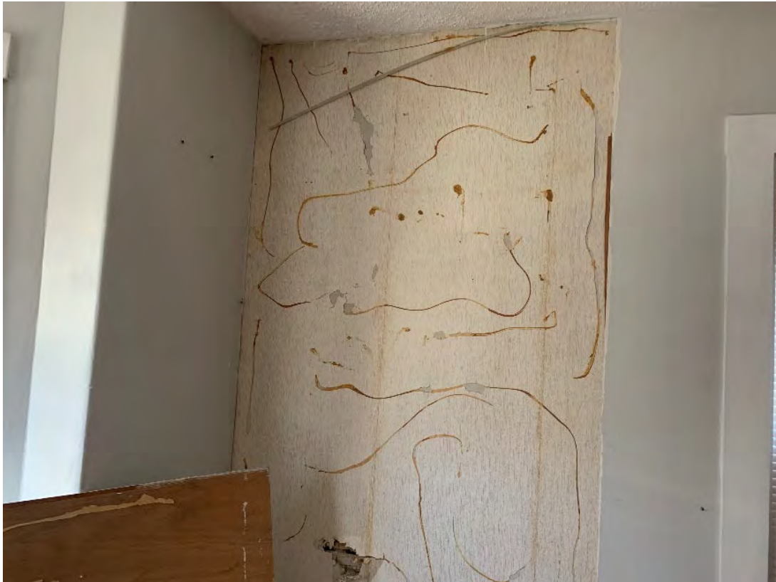
Adhesive on wall panel
