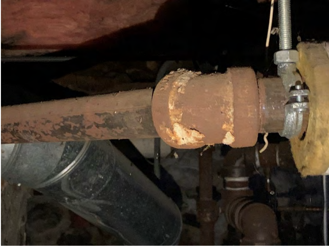
Residual ACM insulation on pipe fittings
