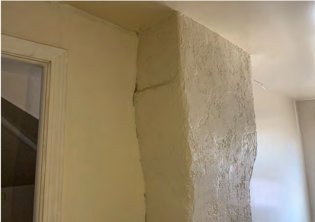
White coating on chimney
