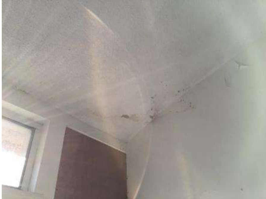
ACM ceiling texture
